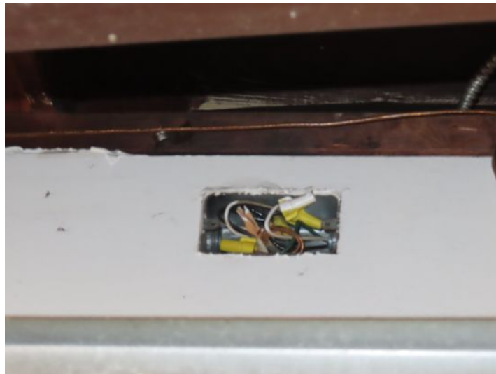
missing junction box cover
