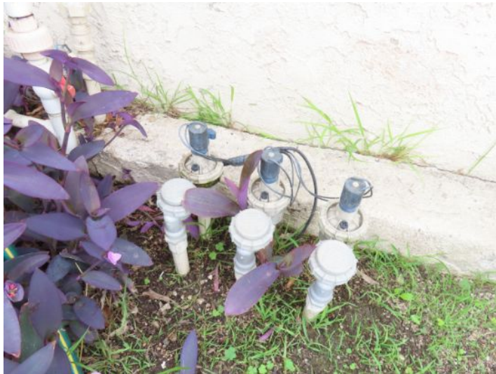
sprinkler valve is leaking
