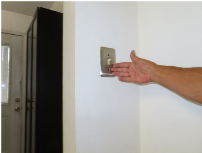
3 way switch is not operating properly at the south hall
