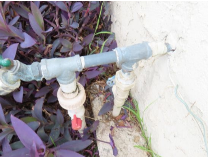
copper to galvanized missing proper connections at the back hose bib/sprinkler connection
