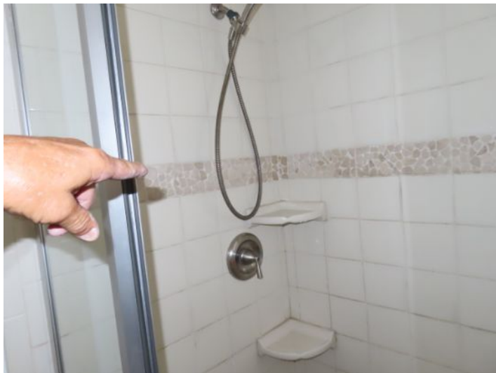
shower fixture drips
