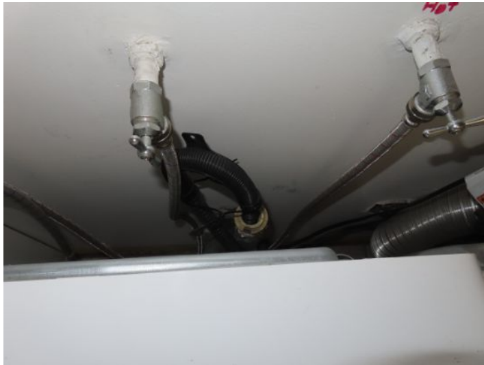
laundry drain pipe is to short
