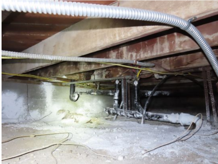
sewer drain line shows signs of leaking
