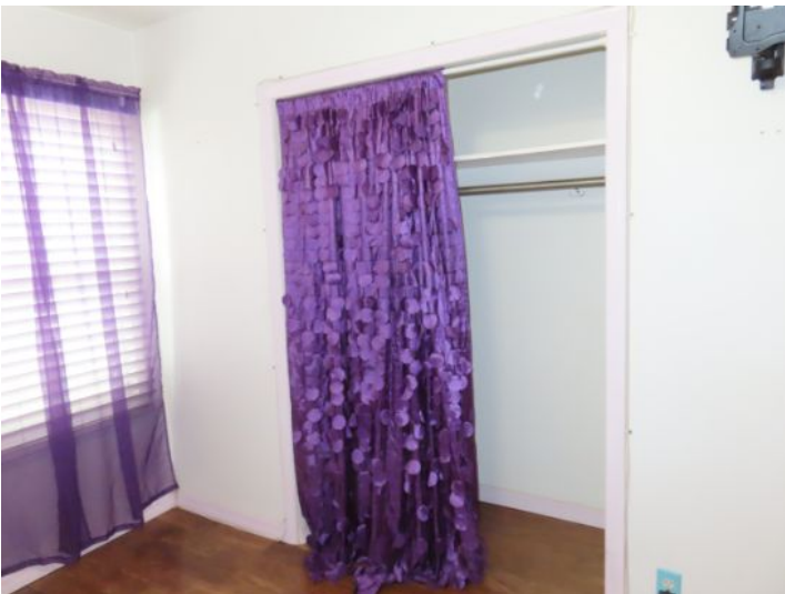
closet doors are missing
