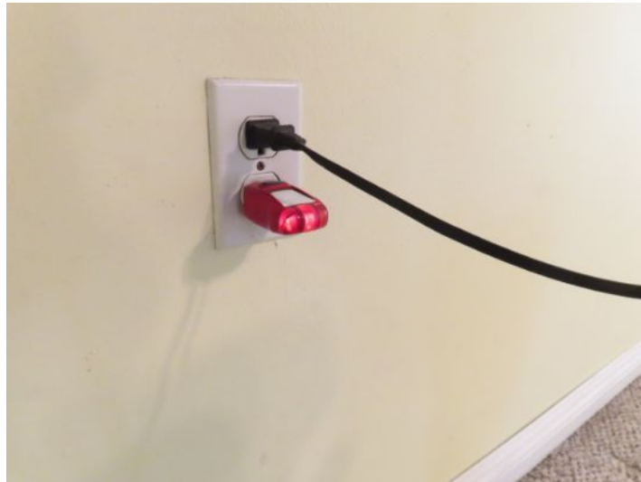
outlet hot wired in reverse at the SE bedroom
