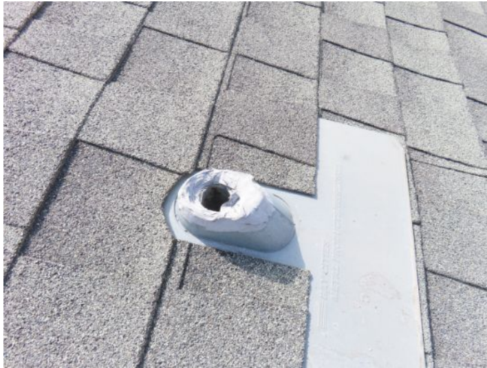
plumbing vent does not extent to proper height
