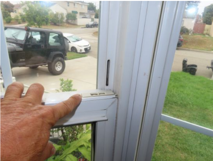
broken and missing secondary window locks at most windows throughout the structure
