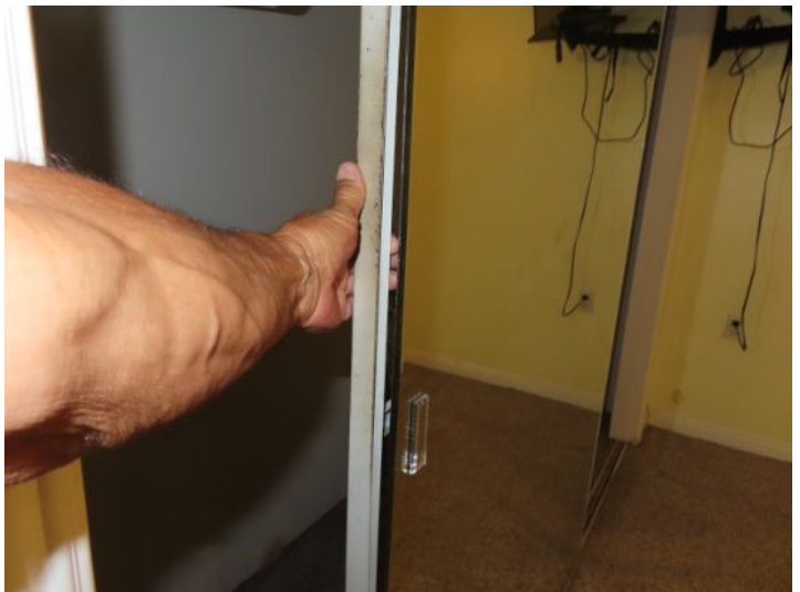
closet door frame is separating from the glass
