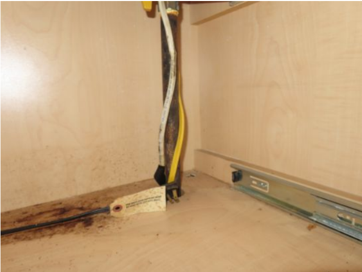
exposed romex wires in the cabinets
