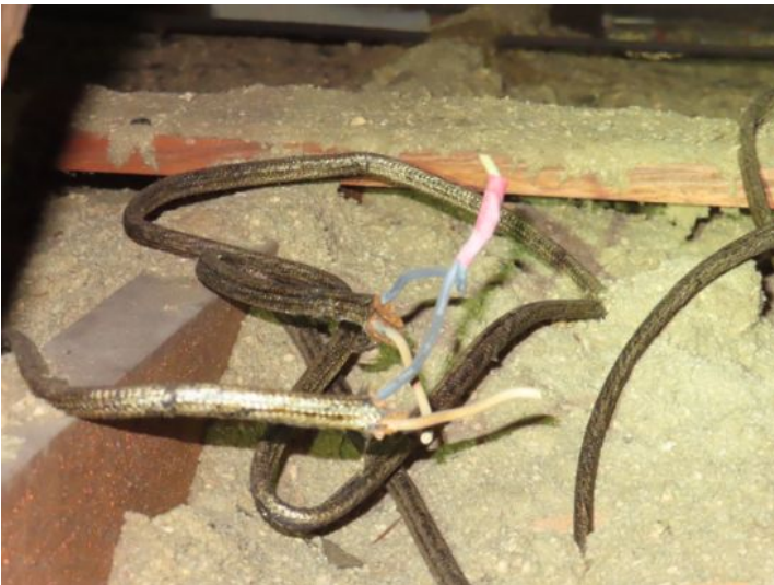
exposed wires and connections
