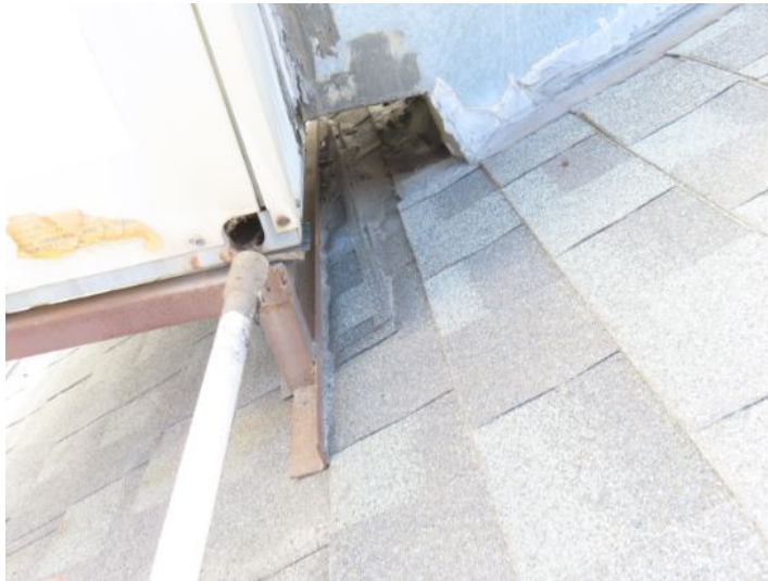
condensation drain line is broken
