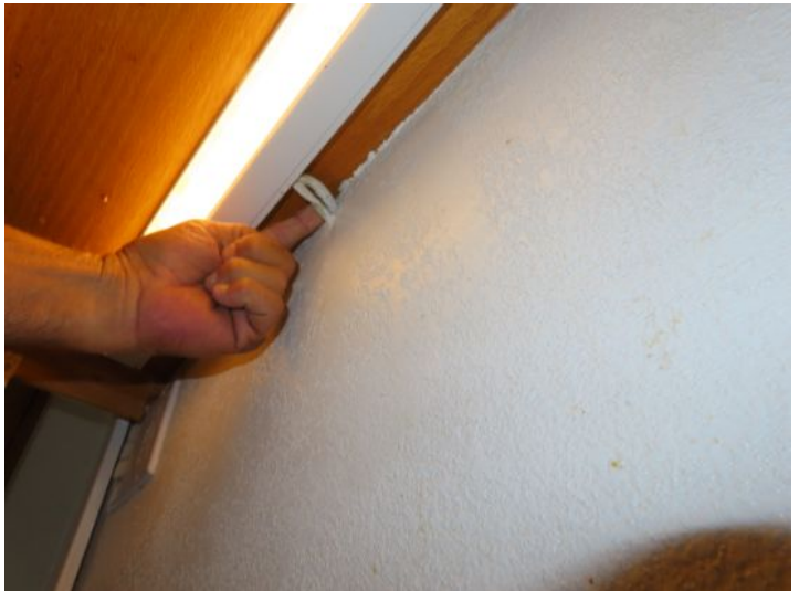
exposed wires at the counter lighting
