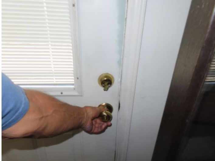
laundry exterior door did not latch
