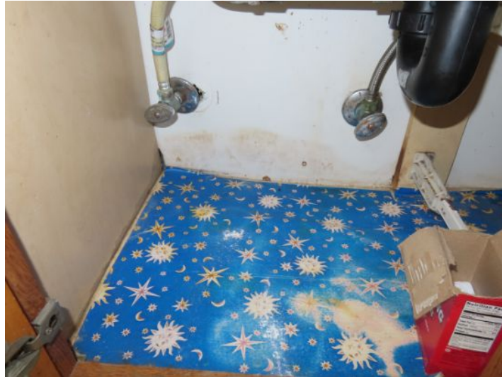
cabinet has water damage under the sink
