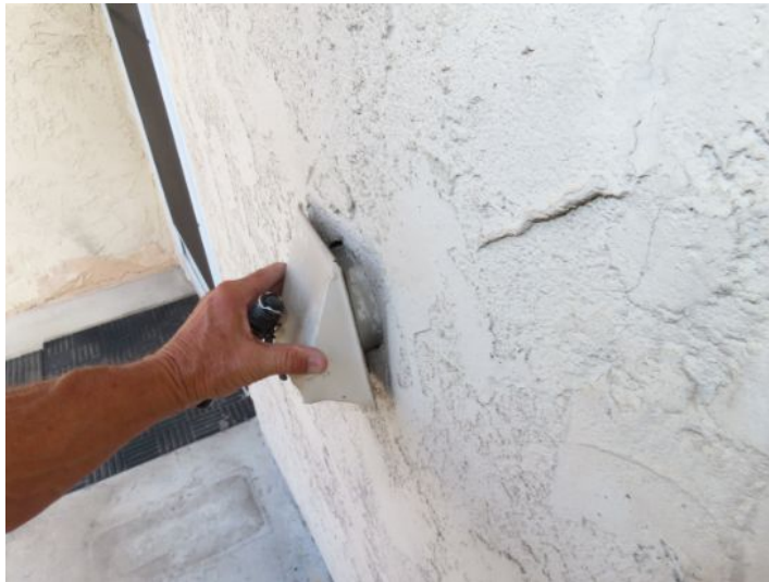
loose exterior cover
