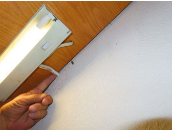
exposed wires at the counter lighting
