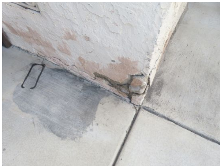
missing in areas
