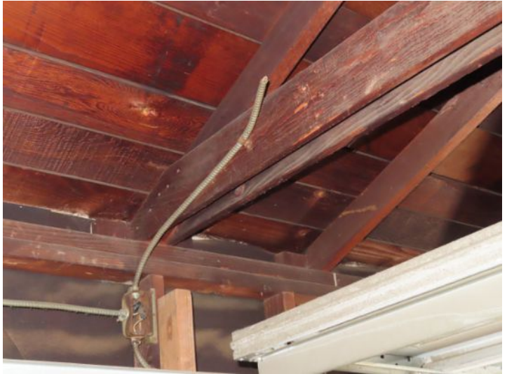
exposed wires, recmmend remove unused electrical
