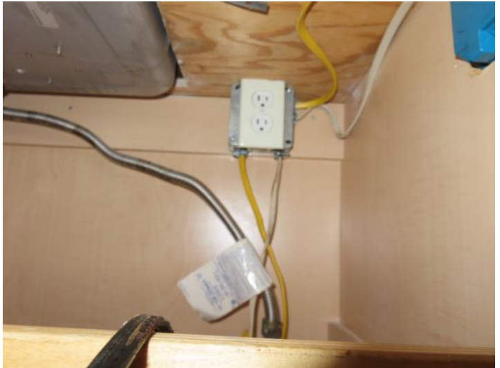
exposed romex wires in the cabinets
