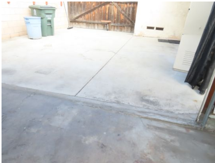
grade slopes toward the garage structure, poor drainage
