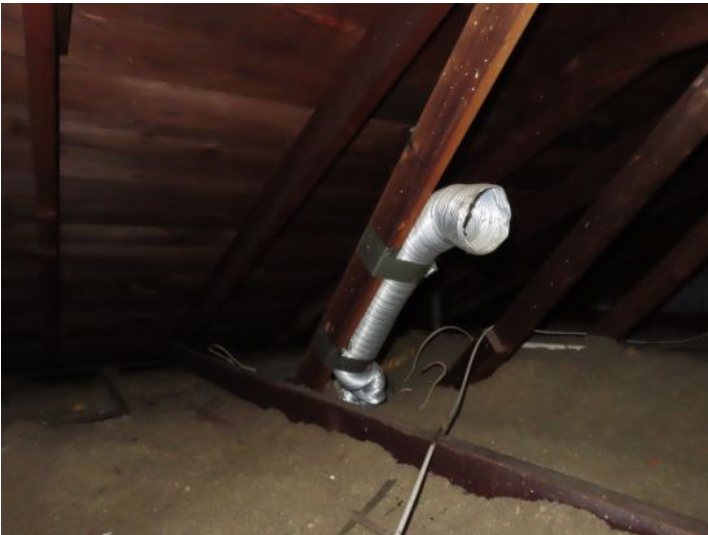
exhaust vent terminates in the attic over the bathrooms
