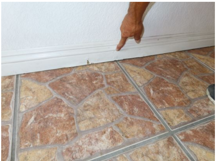
evidence of moisture entering structure at the bonus room
