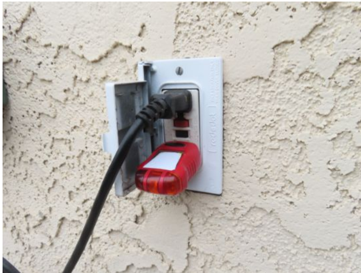
GFCI is not grounded, test did not operate
