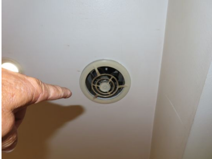
oven exhaust fan did not operate
