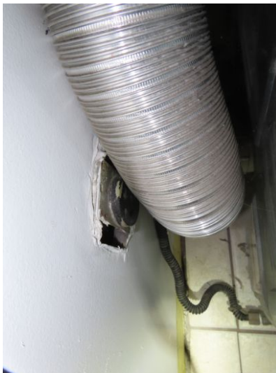
240 volt outlet present, could not access due to the location
