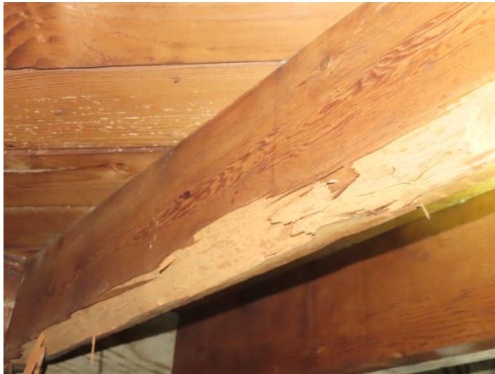
deteriorated wood in areas
