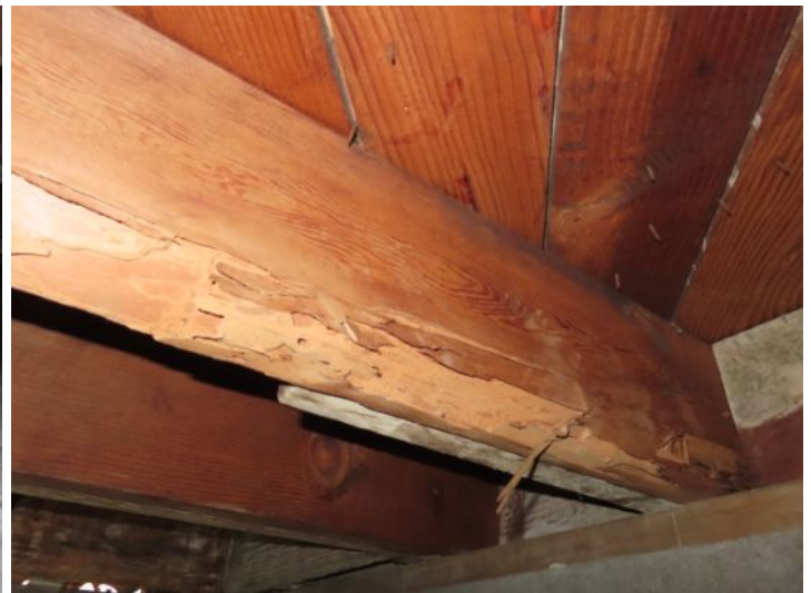
deteriorated wood in areas
