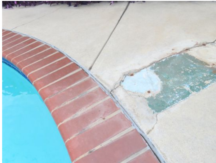
lifting and cracked concrete
