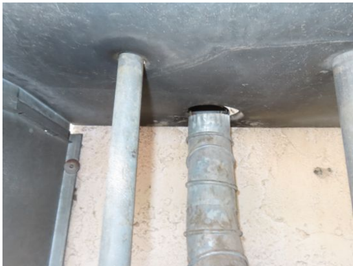
water heater vent pipe is disconnected
