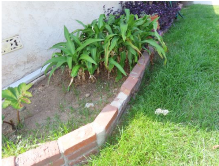
separating cracks, leaning and loose at the brick planter box
