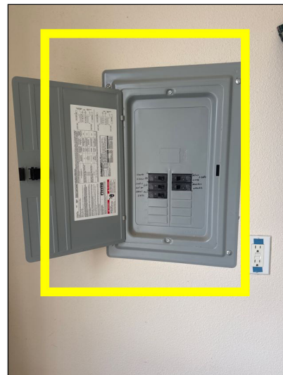
Sub panel to the home
