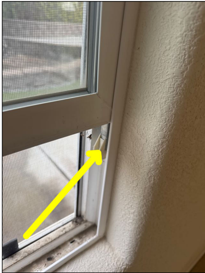
The sash bar has dropped out of place on a single-hung window
