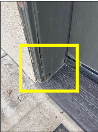
Moisture damage, wood rot, observed.
