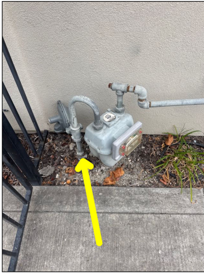
Main gas shut off to the home.
