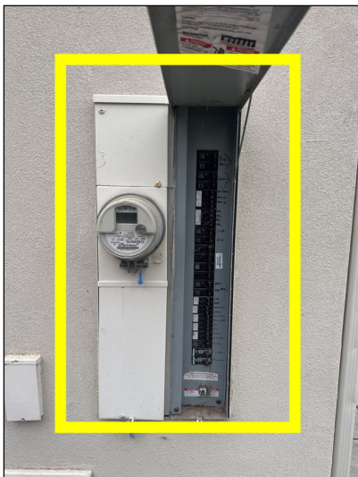
Main electrical service panel to the home.
