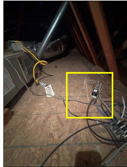
The furnace was plugged into an extension cord/power strip.
