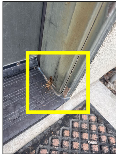
Moisture damage, wood rot, observed.
