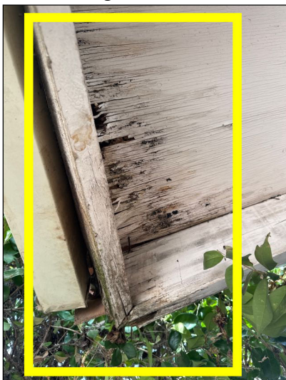
Moisture damage, wood rot, observed.
