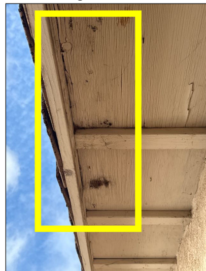
Moisture damage, wood rot, observed.
