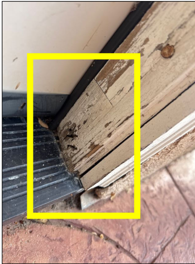
Moisture damage, wood rot, observed.
