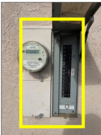
Main electrical service panel to the home.
