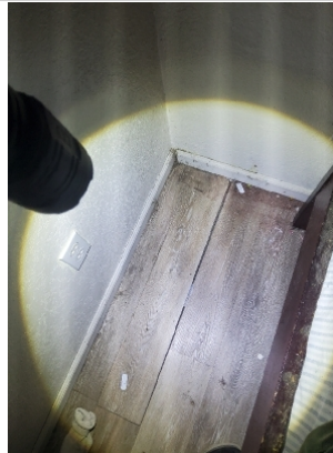
Disconnected flooring, recommend repair
