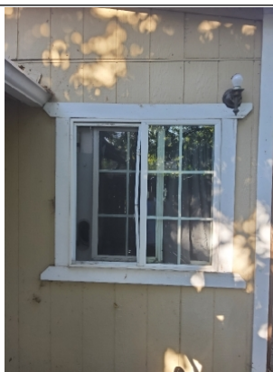
Bent screen, recommend replacing
