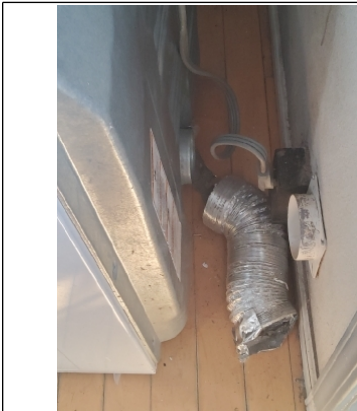
Dryer not venting to exterior, recommend repair
