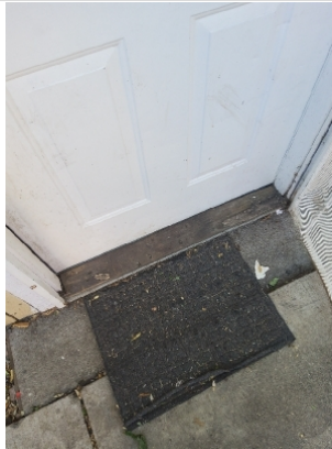
Recommend having threshold replaced by a licensed contractor
