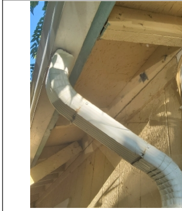
Active leak on downspout, recommend repair
