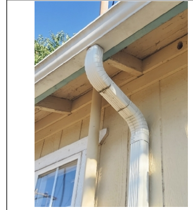
Active leak on downspout, recommend repair
