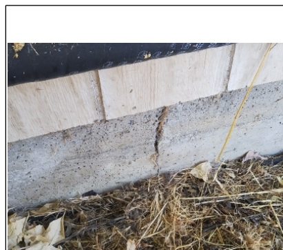
Foundation crack evident, recommend repair (Not as major of an issue as this home is built on a concrete slab). Epoxy injection can repair the crack
