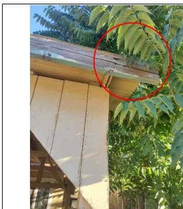
Moisture damage is evident on fascia, recommend replacing
