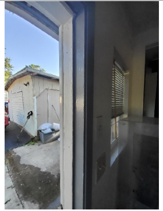
Missing weatherstripping, recommend installing
