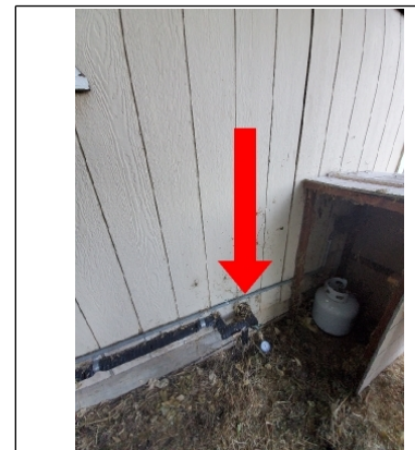
Water shut off location
