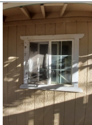
Bent screen, recommend replacing
