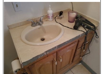
Missing corner pieces on countertop, recommend repair
