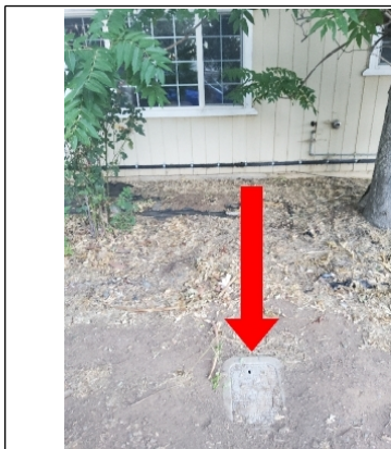
Water meter location
