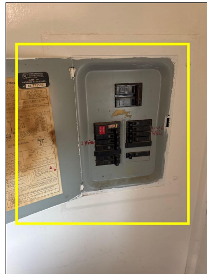
Sub panel to the home
