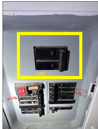
Main electrical shut off to the home
