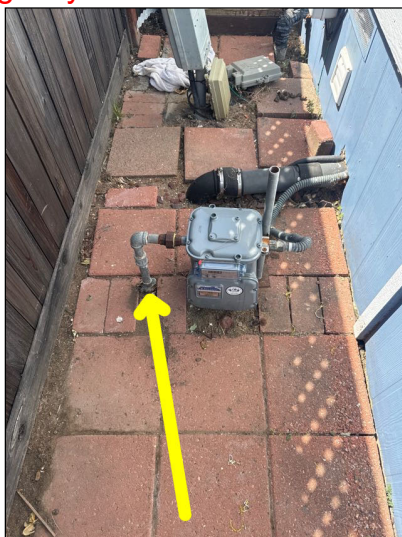
Main gas shut off to the home.
