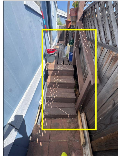
The rear stairs were old, damaged and appear unsafe.
