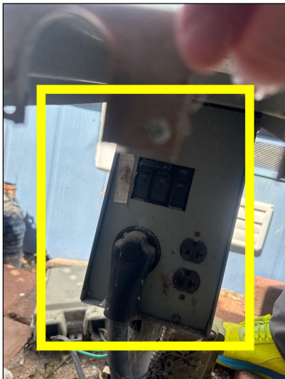
Main electrical service pedestal to the home.
