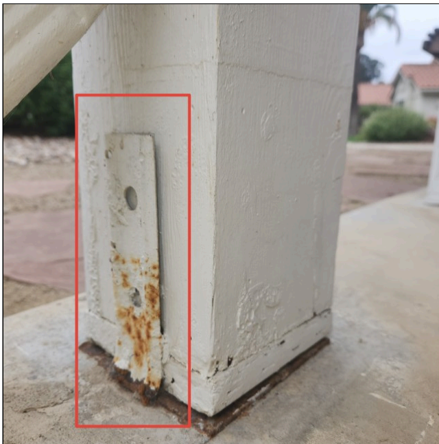
Rusting Bracket. Missing Fasteners.
