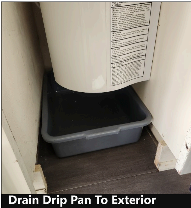
5.0.B WATER HEATER
