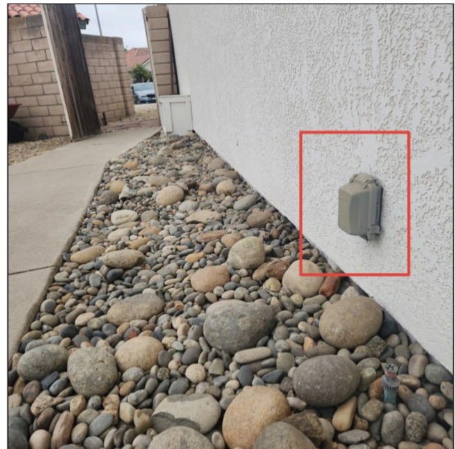
Outlet Without Power
