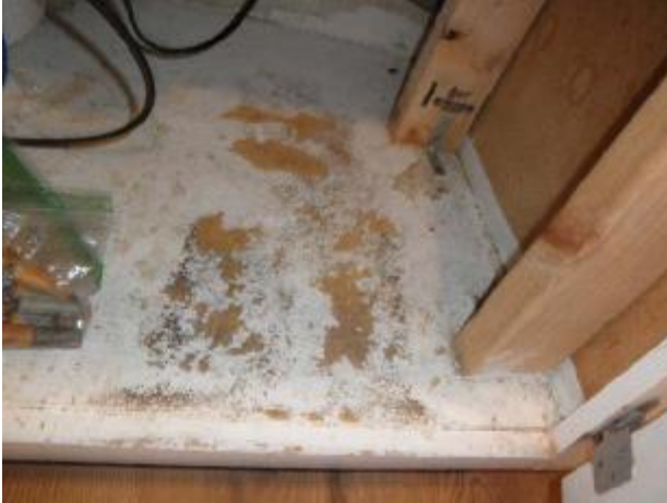
Moisture damage to the base of the kitchen sink cabinet.
