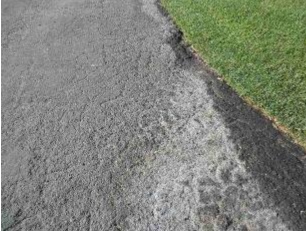
The asphalt driveway needs to be sealed.
