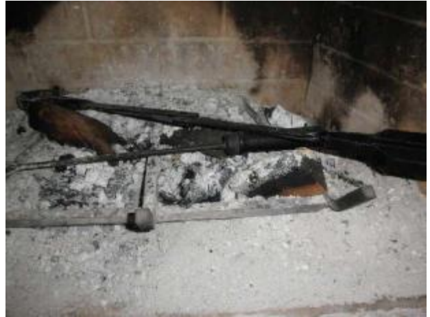
Example of heavy ash in the firebox.
