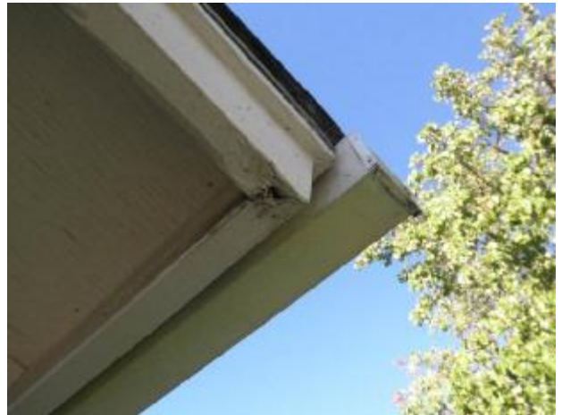
Moisture damage garage fascia.
