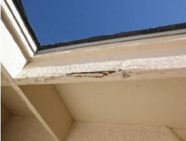
Moisture damage garage fascia.
