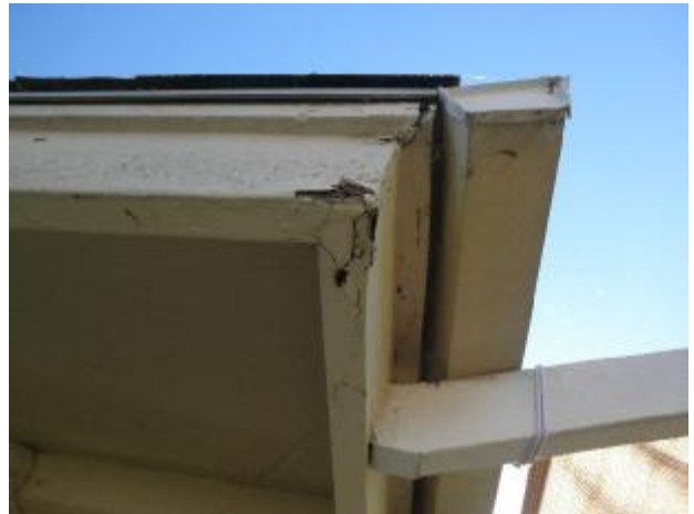
Moisture damage at the SW fascia and trim.
