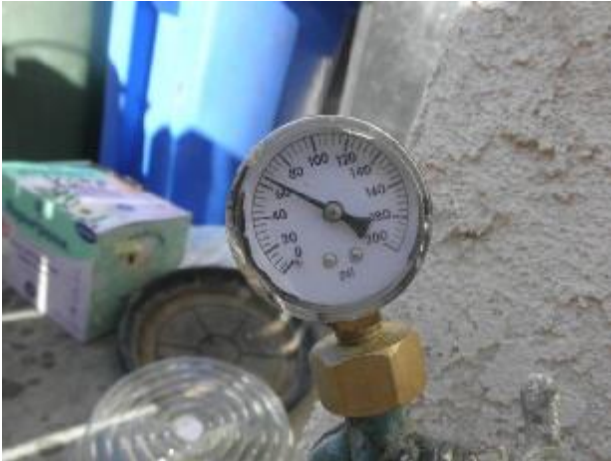
Water pressure is 60 psi.
