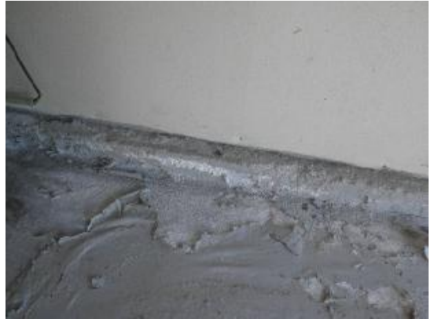
Efflorescence at the garage west wall.
