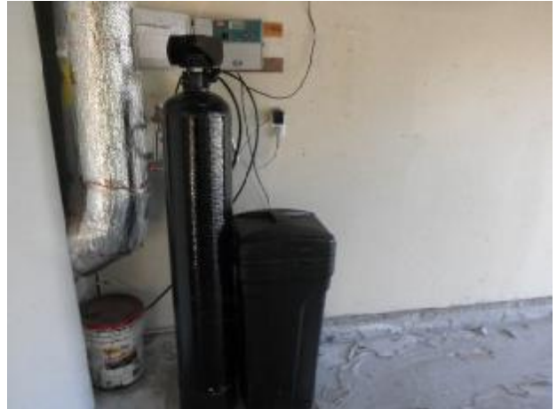
Water softener installed in the garage.
