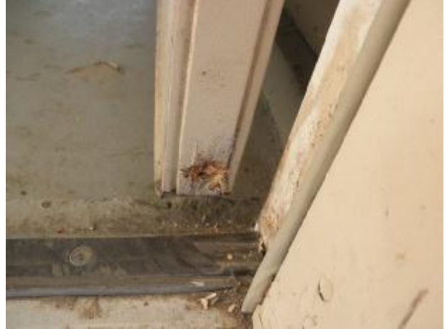
Moisture damage at the garage side door spine.
