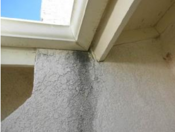
Gutter seam is leaking.
