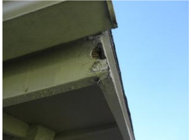
Moisture damage front entry fascia.
