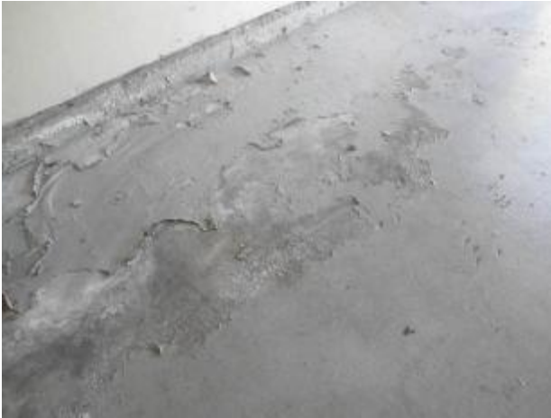
The seal at the garage slab is peeling.
