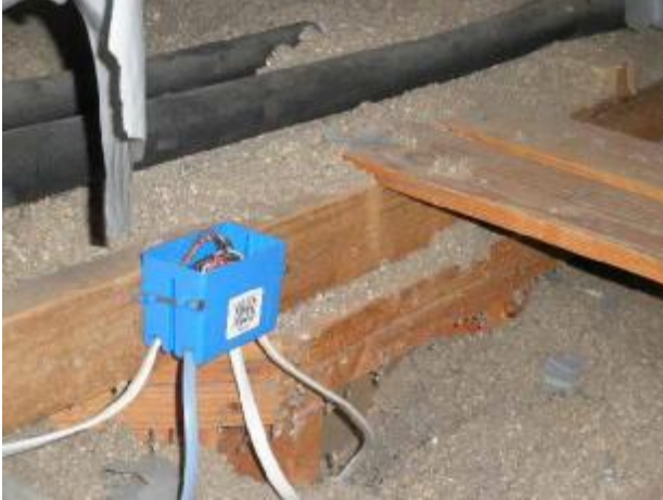
Example of open junction boxes in the attic.
