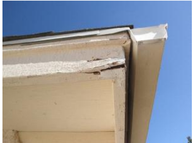
Moisture damage garage fascia.
