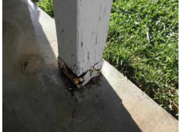
Example of moisture damage to the base of the trellis posts.
