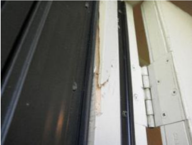
Entry door jamb cracked/damaged.
