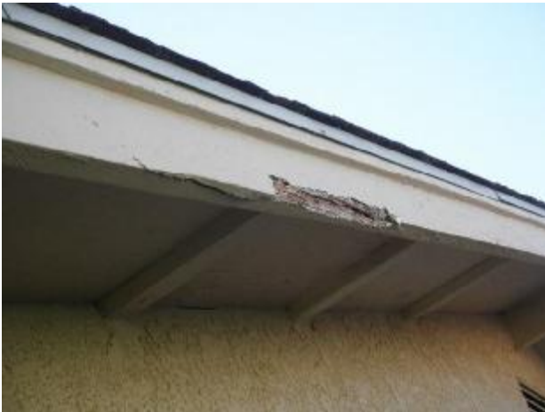
Moisture damage front entry fascia.
