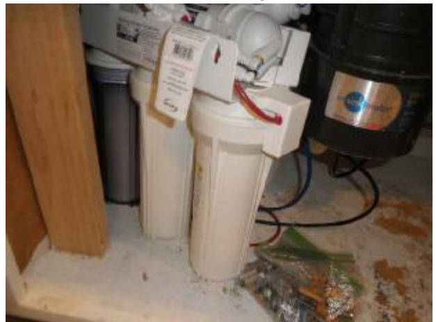
Reverse osmosis installed under the kitchen sink.
