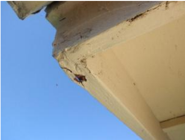
Moisture damage at the SE fascia.
