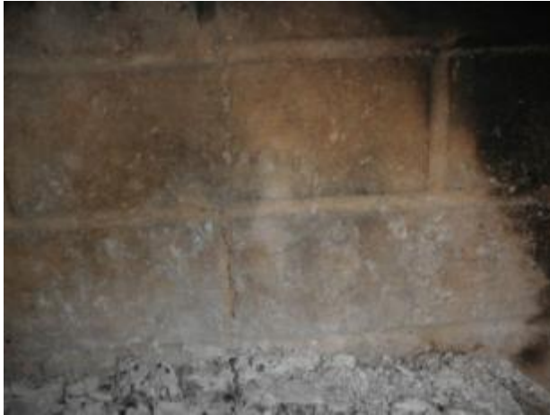
Cracks in the refractory plates inside the firebox.
