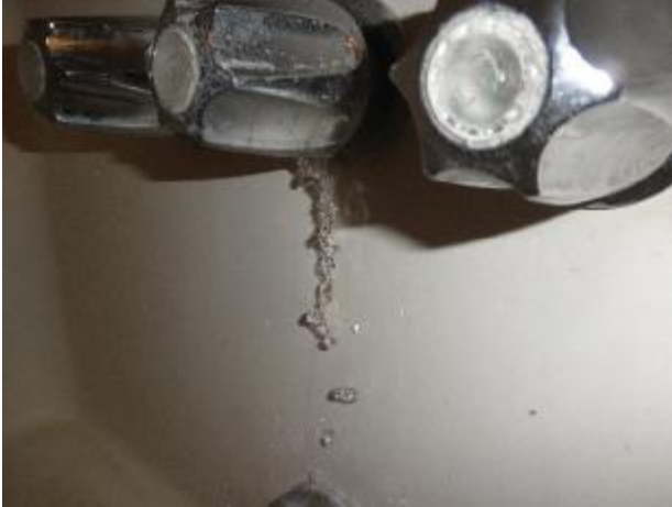
Hall bathroom shower handles leak when operated.
