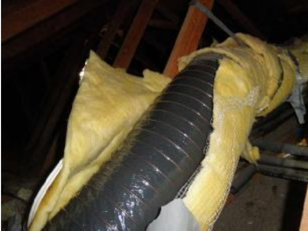
Insulation falling off some of the ducts in the attic.
