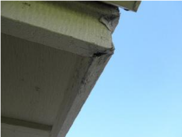
Moisture damage at the NW fascia.
