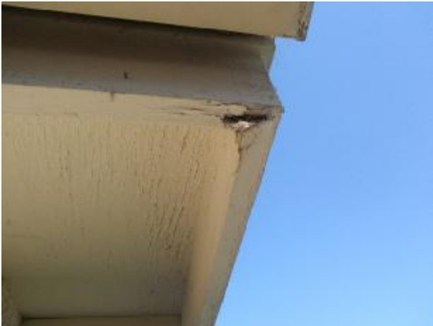
Moisture damage garage fascia.
