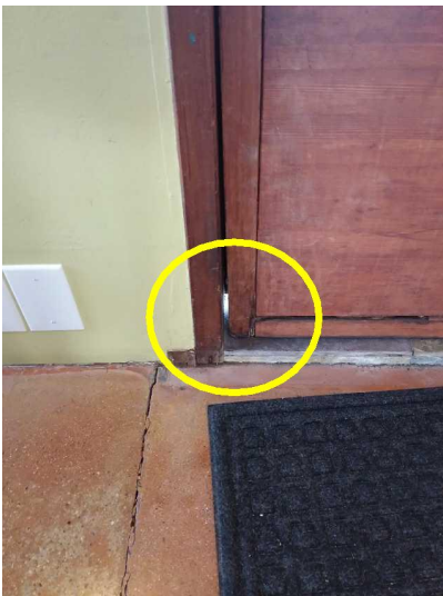
The front door is functional but not fully weather sealed.
