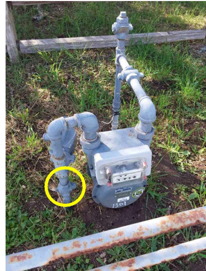
The gas meter and shut off are located at the street.
