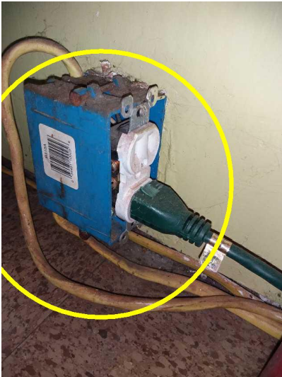
An outlet has an open ground, and should be serviced.
