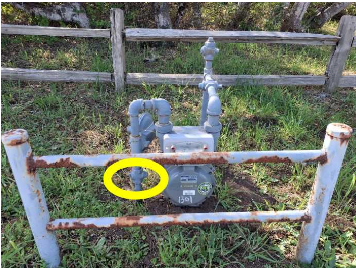
The gas main shut-off is located adjacent to the street.
