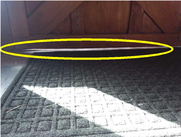
The front and rear door are functional but not fully weather sealed.
