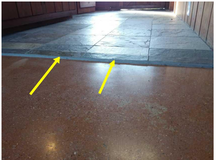
There are one or more offsets which could be a trip hazard that you may wish to have serviced.
