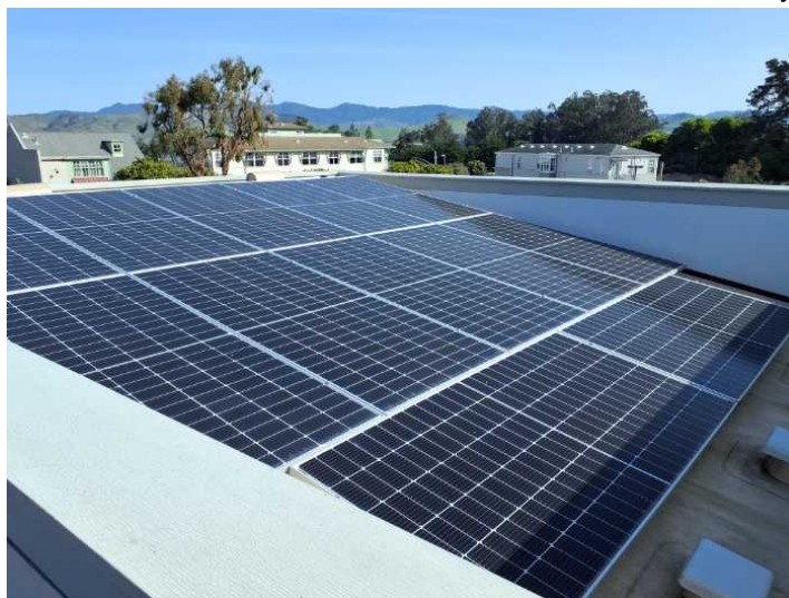
12 Panels on the roof
