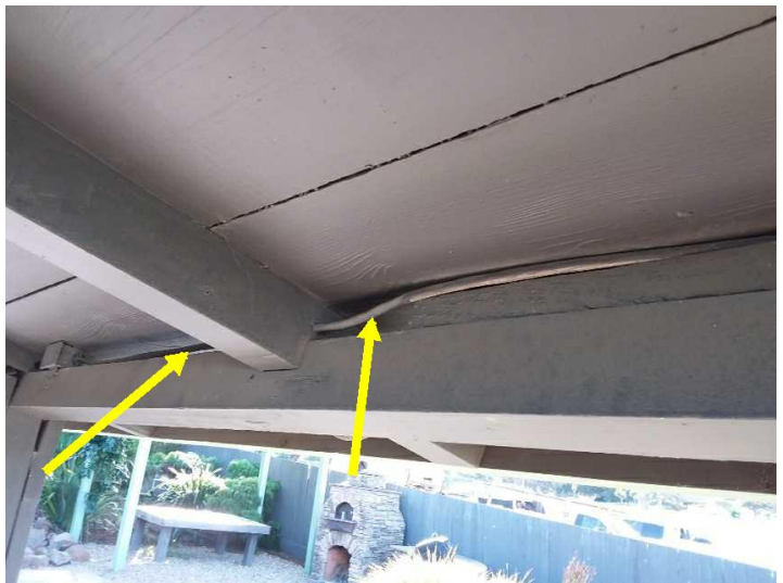
There's exposed romex electrical cable that should be protected inside conduit. A licensed electrician should evaluate and service this issue.
