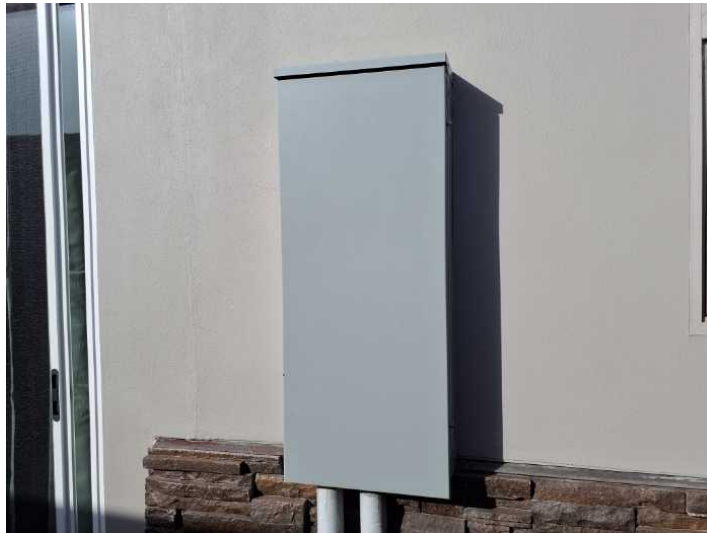
The sub panel is located at the left exterior side of the home.
