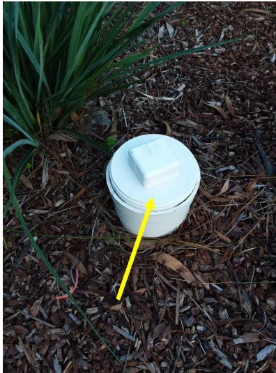
A clean-out is located at the front.
