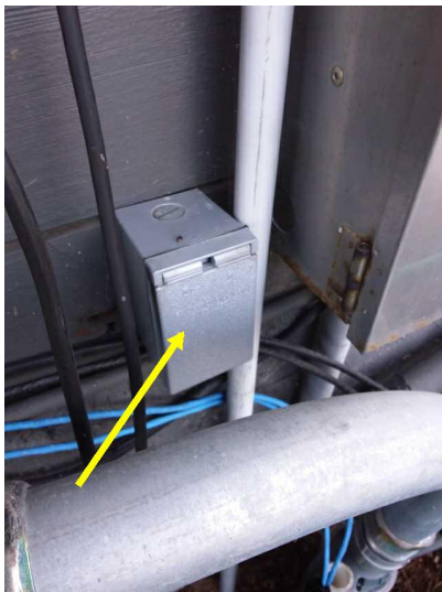
An outlet at the right side has an open-ground and should be evaluated and serviced by a licensed electrical contractor.
