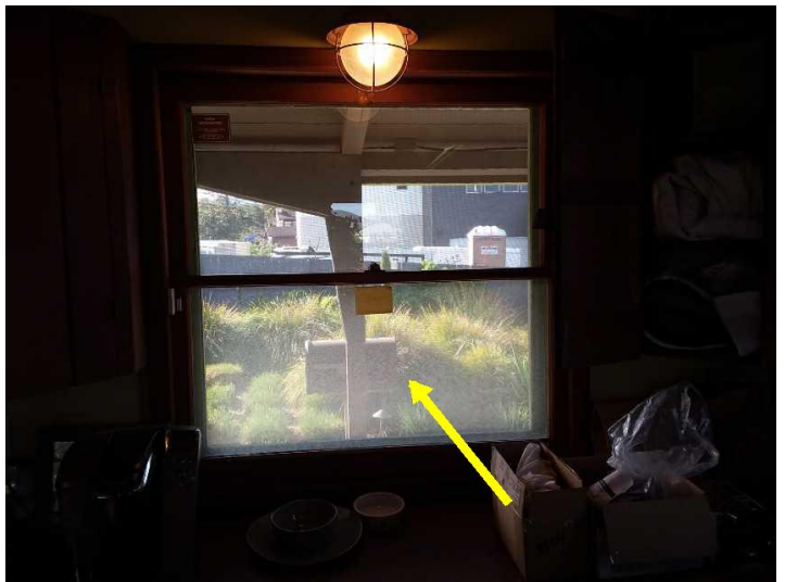
A single-hung window will need service such as adjusting or replacing the hardware to open and close smoothly and safely.
