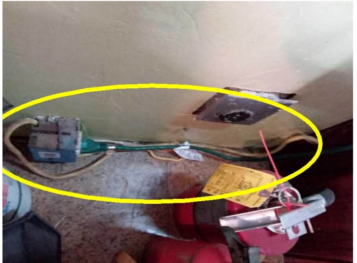
There is exposed romex that should be protected by installing the romex inside the wall cavity, or properly wired into conduit.
