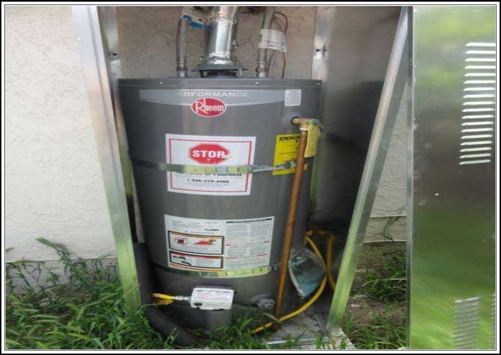
WATER HEATER ADU
