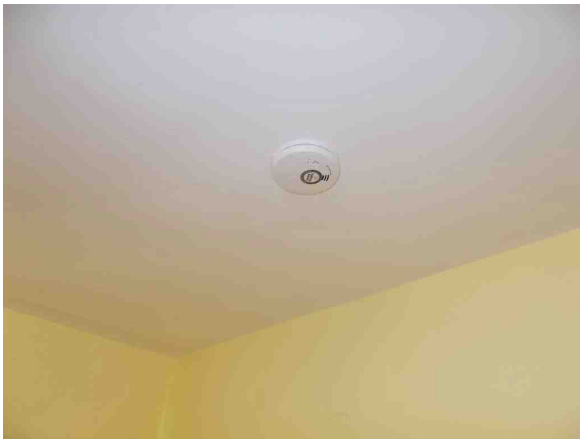
Bedroom 3 Smoke Detector
