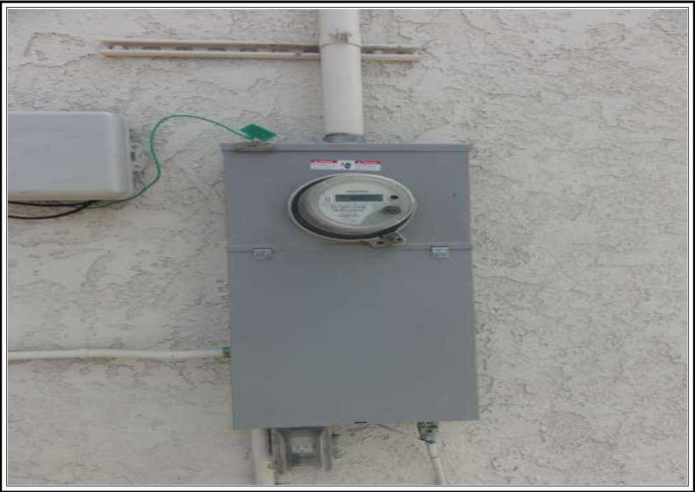
ELECTRIC METER ADU
