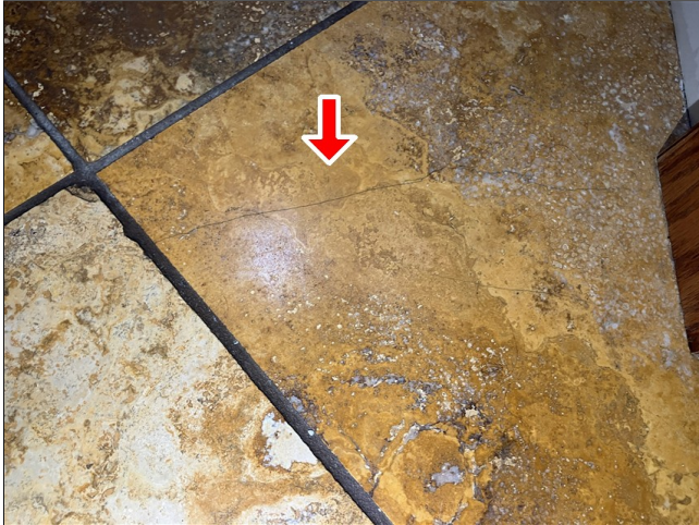
4.1 Item 1(Picture) hall bath: crack in floor tile visible
