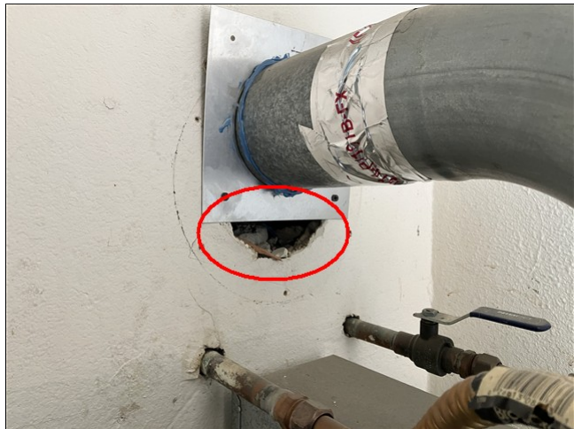
4.0 Item 1(Picture) front patio closet: hole in drywall observed
