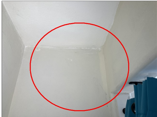
4.0 Item 4(Picture) interior: wall surface maintenance/repairs needed
