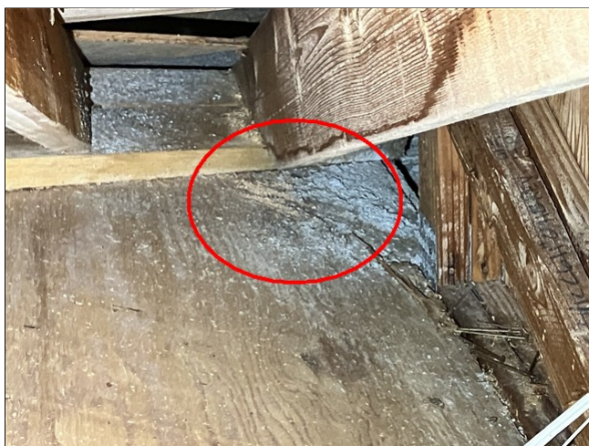
5.4 Item 1(Picture) possible WDO evidence or damage observed
