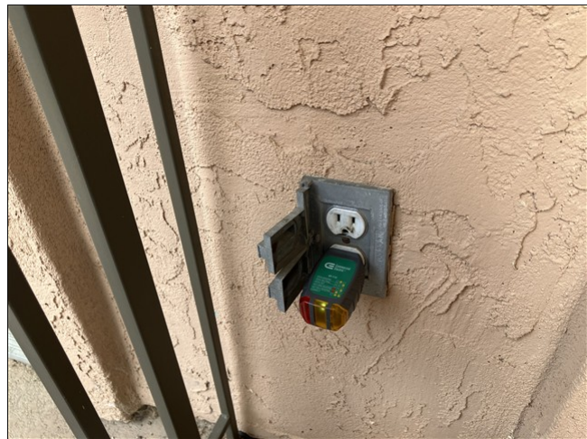
7.6 Item 3(Picture) exterior: recommend evaluation and upgrade of any non-GFCI outlets
