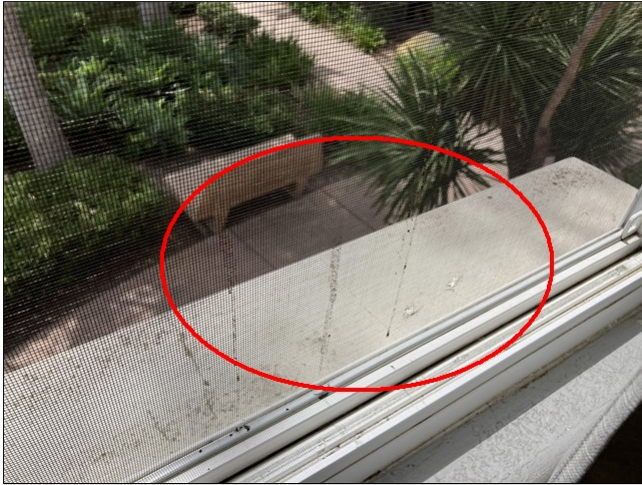
4.5 Item 1(Picture) bedroom window: screen damage visible
