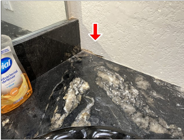
4.0 Item 11(Picture) primary bedroom bath: wall damage visible
