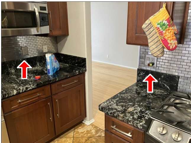
7.6 Item 4(Picture) kitchen: recommend evaluation and upgrade of any non-GFCI outlets
