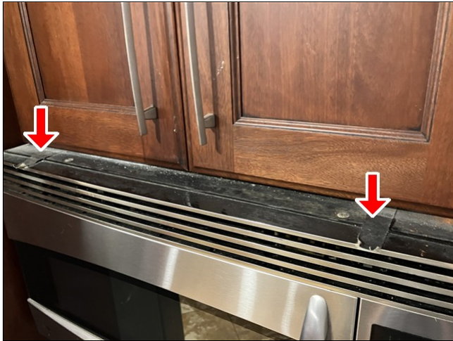
10.4 Item 1(Picture) microwave cover appeared loose (tape observed)
