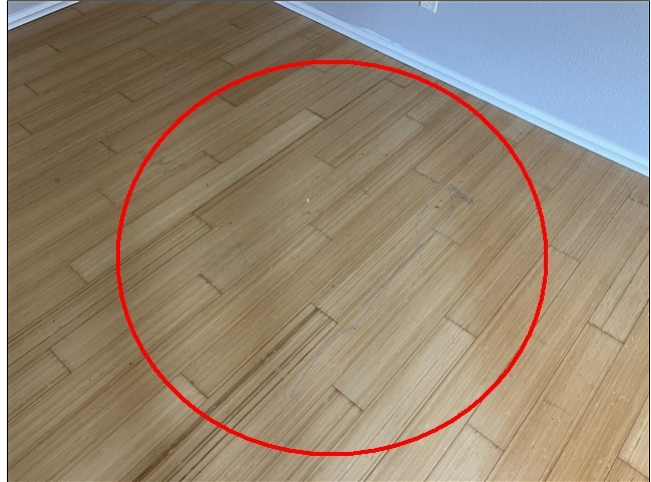
4.1 Item 2(Picture) primary bedroom: floor scratches observed
