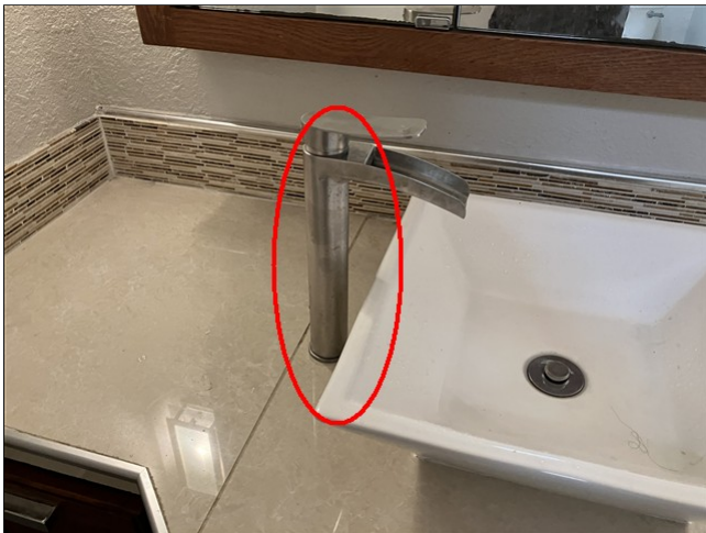
6.5 Item 1(Picture) hall bath: loose faucet fixture
