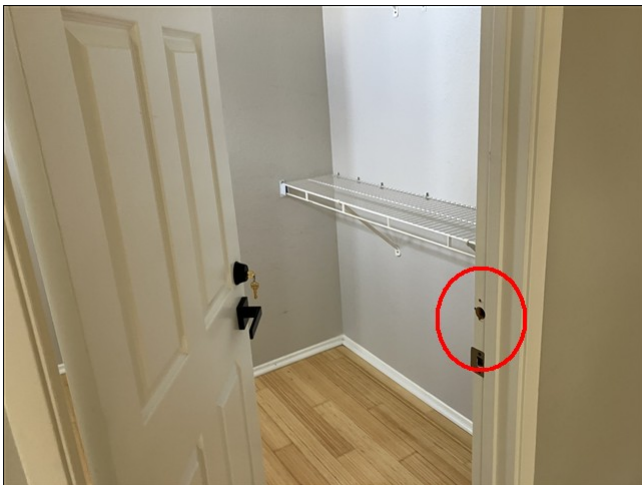
4.3 Item 1(Picture) primary bedroom closet: missing dead bolt latch receiver
