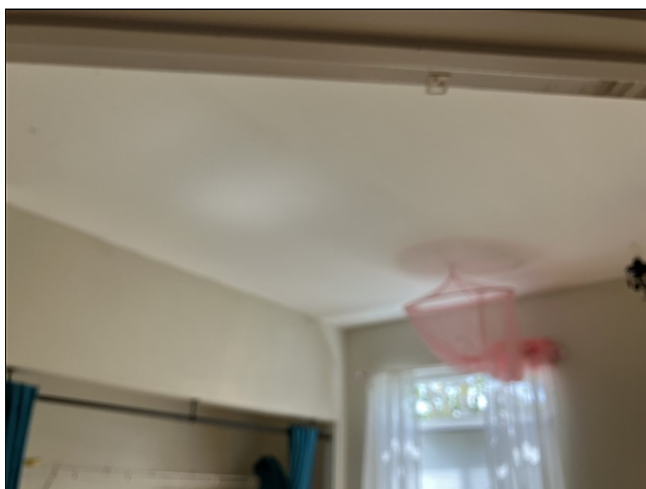
7.7 Item 1(Picture) bedroom: missing smoke detector
