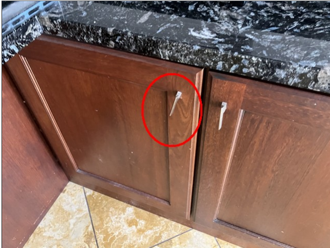
4.4 Item 1(Picture) dining area: loose handle
