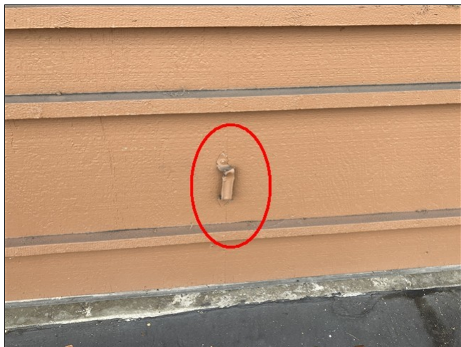
3.4 Item 1(Picture) handle damage visible
