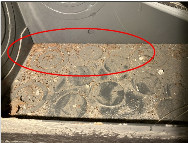
4.8 Item 1(Picture) inside electrical panel: possible WDO evidence or damage observed
