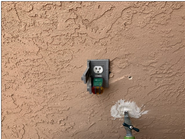
7.6 Item 2(Picture) exterior: recommend evaluation and upgrade of any non-GFCI outlets
