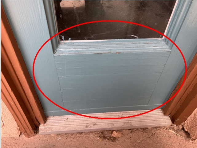
2.1 Item 3(Picture) front patio: door paint maintenance/repairs needed
