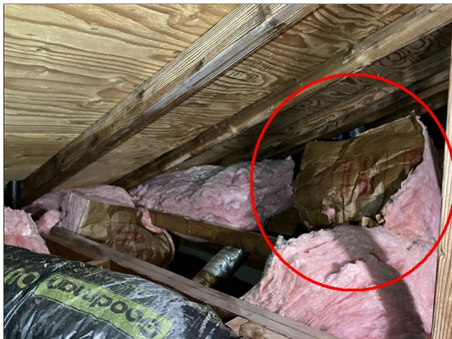
9.0 Item 1(Picture) displaced insulation observed (paper backing should not be exposed)
