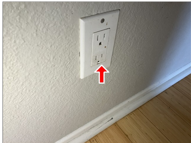
7.5 Item 6(Picture) damaged outlet
