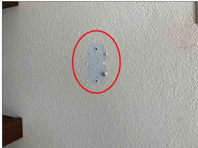
4.0 Item 2(Picture) interior: wall surface maintenance/repairs needed
