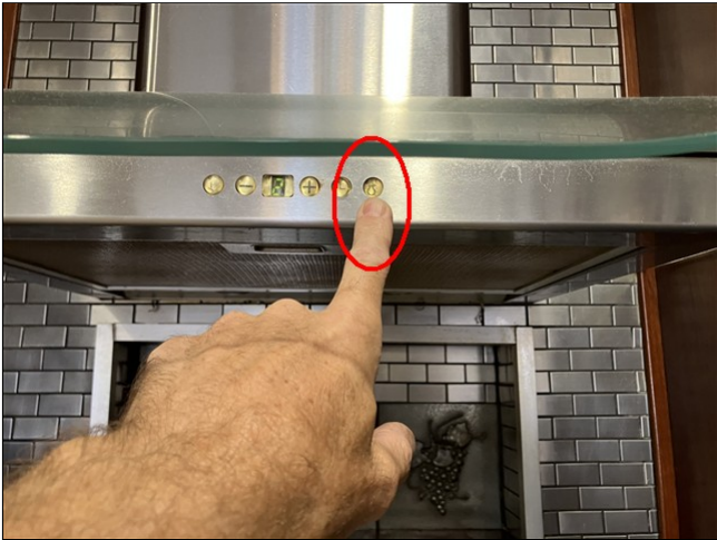
10.2 Item 1(Picture) hood light did not turn on when tested
