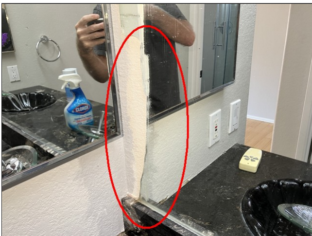
4.4 Item 5(Picture) primary bedroom bath: broken mirror observed
