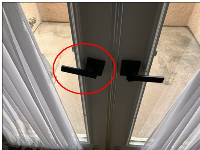
2.1 Item 2(Picture) dining area patio: loose door handle
