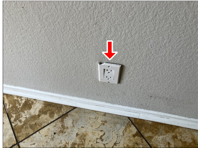
7.5 Item 4(Picture) damaged outlet cover
