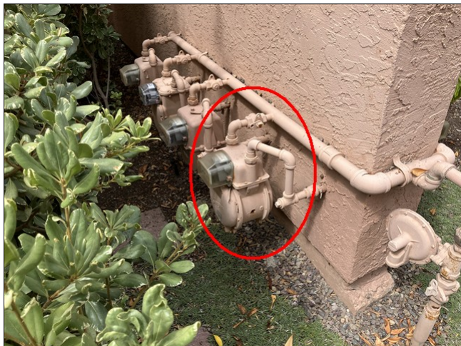
6.1 Item 1(Picture) gas meter and shut-off valve for unit 87
