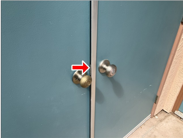
2.1 Item 5(Picture) front patio closet door did not latch when tested
