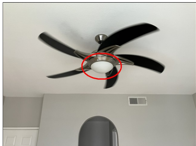
7.5 Item 8(Picture) primary bedroom fan light did not turn on when tested
