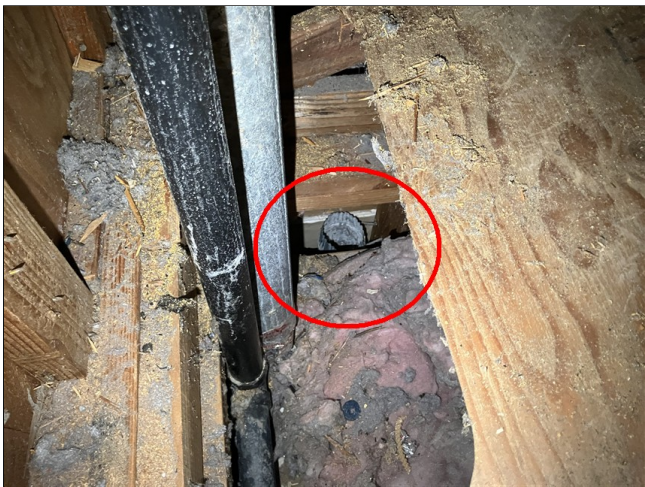
9.1 Item 1(Picture) recommend evaluation and proper removal of abandoned dryer ducting materials
