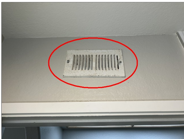
8.7 Item 2(Picture) bedroom bath: oxidation visible at register
