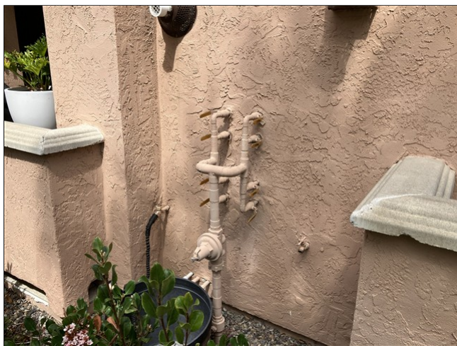
6.0 Item 1(Picture) house water shut off valves (not labelled) / corresponding valve was not identified
