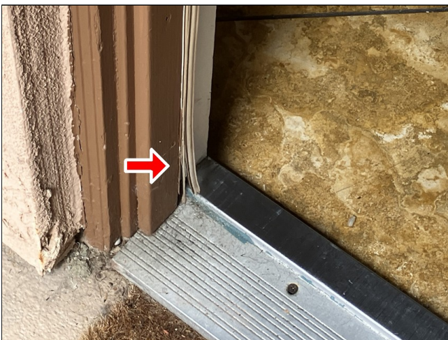
2.1 Item 1(Picture) front door: weather stripping maintenance/repairs needed
