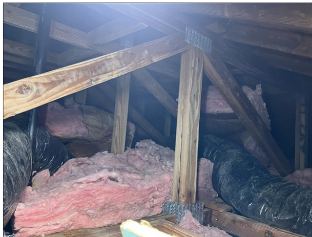
9.0 Item 2(Picture) displaced insulation observed
