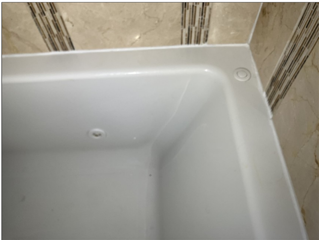
6.8 Item 3(Picture) tub spa jets were not inspected or tested as part of the scope of this inspection
