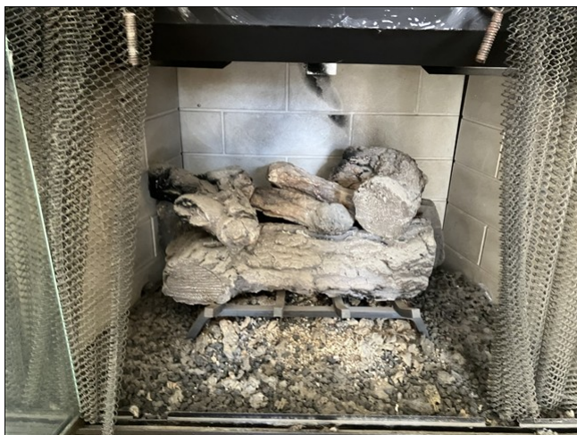
8.9 Item 1(Picture) a fireplace and chimney flue performance and safety inspection by a qualified person is recommended
