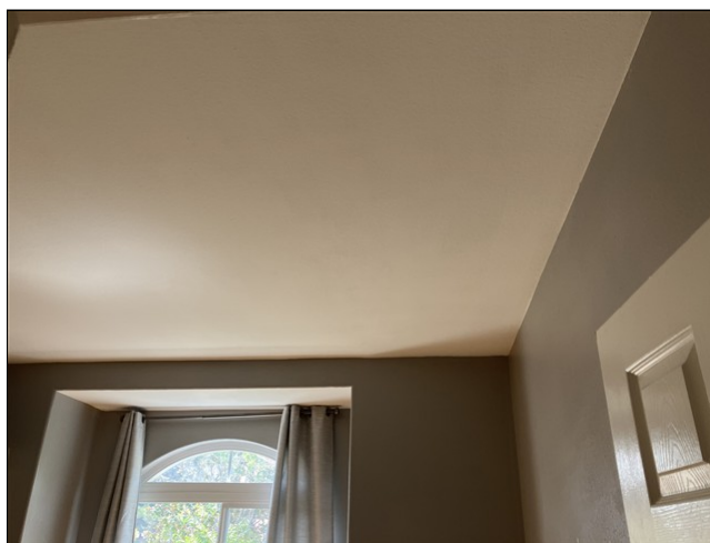
7.7 Item 2(Picture) bedroom: missing smoke detector
