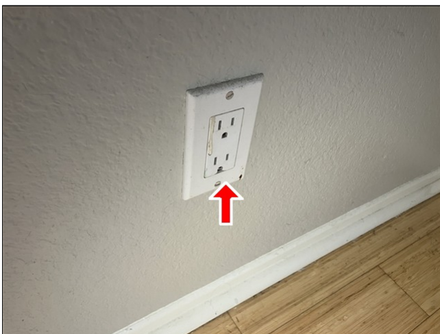
7.5 Item 7(Picture) damaged outlet
