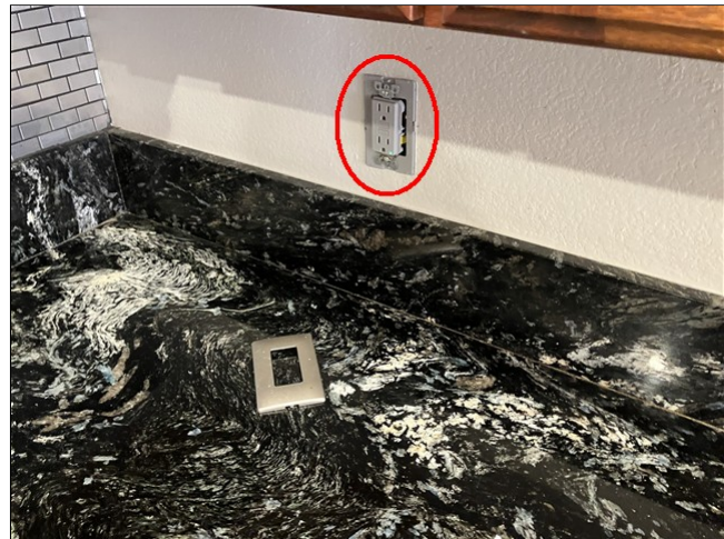
7.5 Item 2(Picture) kitchen : outlet cover maintenance/ repairs needed
