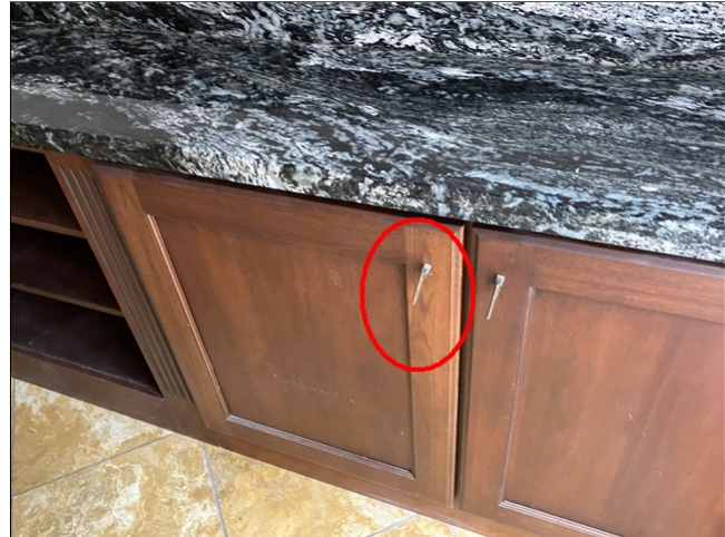
4.4 Item 2(Picture) dining area: loose handle
