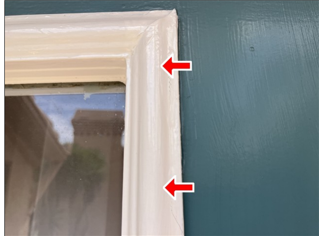
2.1 Item 4(Picture) front patio: door paint maintenance/repairs needed
