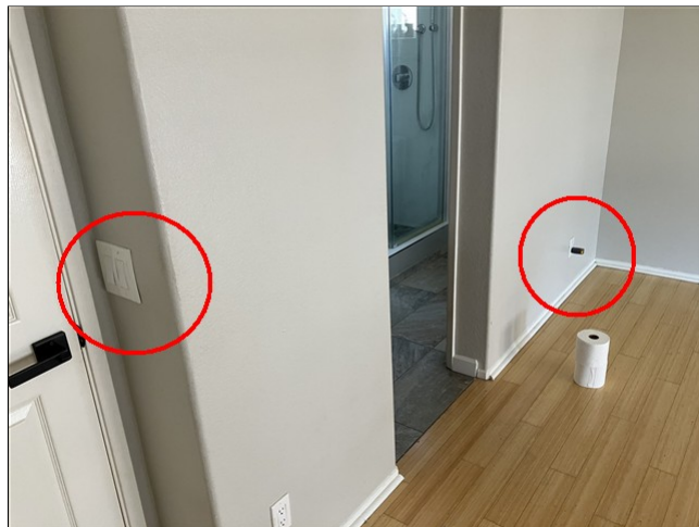
7.5 Item 11(Picture) primary bedroom: switch and corresponding outlet were not identified / recommend further evaluation
