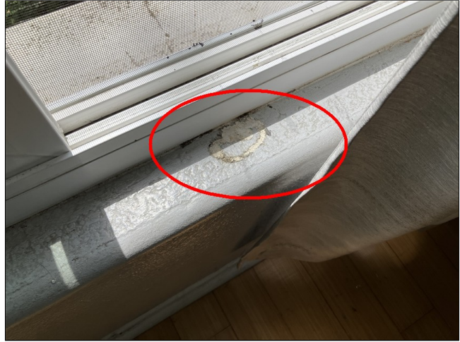
4.0 Item 6(Picture) interior: wall surface maintenance/ repairs needed
