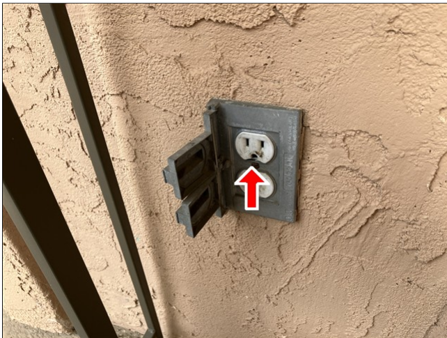
7.5 Item 1(Picture) exterior: damage outlet
