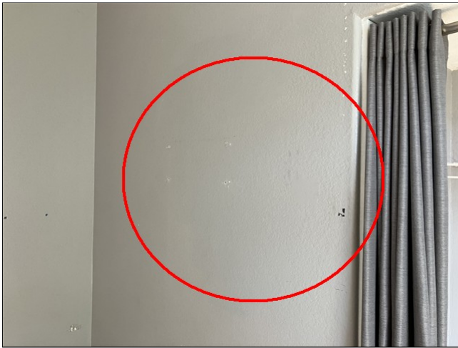
4.0 Item 7(Picture) interior: wall surface maintenance/ repairs needed
