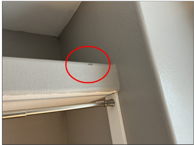
4.0 Item 8(Picture) interior: wall surface maintenance/ repairs needed
