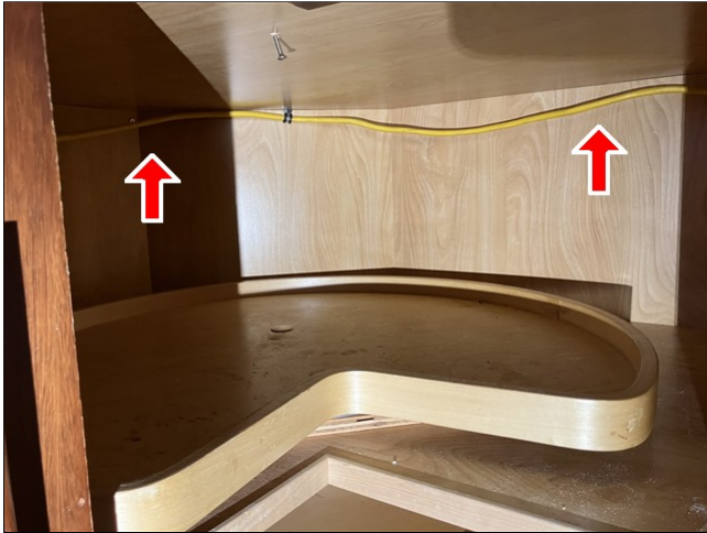
7.4 Item 1(Picture) kitchen: exposed wiring appeared susceptible to damage / recommend further evaluation
