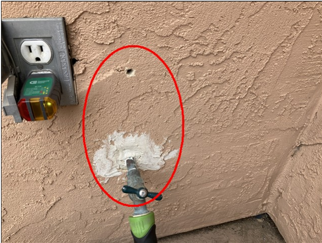
2.0 Item 1(Picture) patio: stucco maintenance/repairs needed
