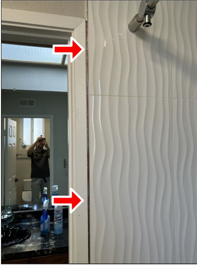
4.6 Item 3(Picture) primary bedroom bath: caulking or appropriate sealant maintenance/repairs needed
