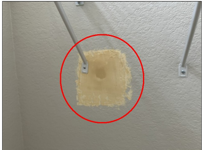
4.0 Item 10(Picture) interior: wall surface maintenance/ repairs needed
