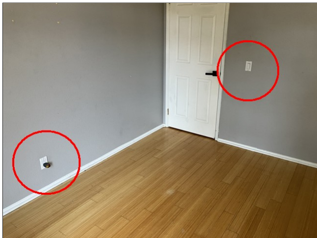
7.5 Item 10(Picture) bedroom: switch and corresponding outlet were not identified / recommend further evaluation
