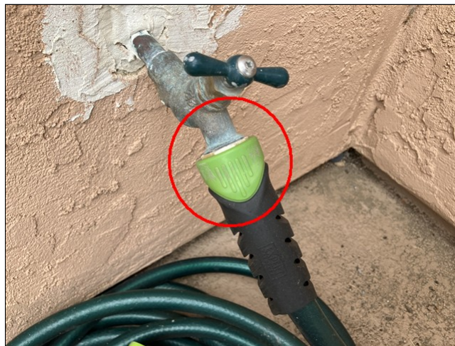
6.4 Item 2(Picture) vacuum breaker (anti-siphon device) upgrade recommended at exterior spigot(s)
