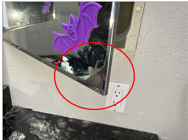
4.4 Item 4(Picture) primary bedroom bath: medicine cabinet oxidation visible
