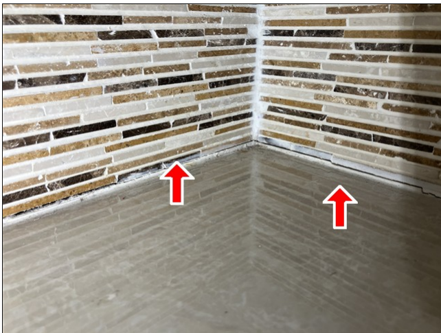
4.6 Item 1(Picture) hall bath: caulking or appropriate sealant maintenance/repairs needed
