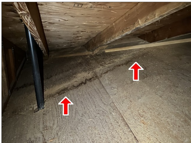
5.4 Item 2(Picture) attic: stains visible
