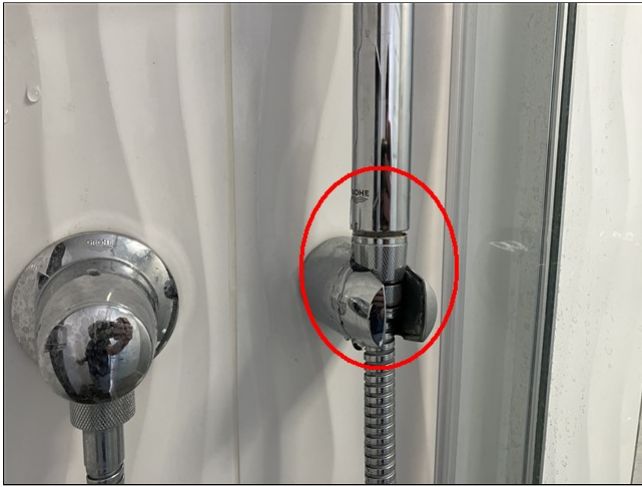
6.5 Item 3(Picture) primary bedroom bath: leaked when tested
