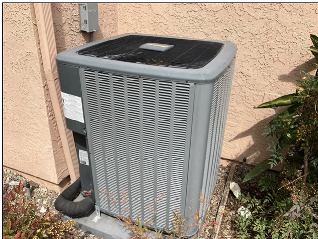
8.4 Item 1(Picture) a/c condenser: no visible maintenance record observed
