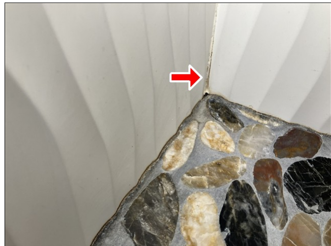
4.6 Item 2(Picture) primary bedroom bath: caulking or appropriate sealant maintenance/repairs needed
