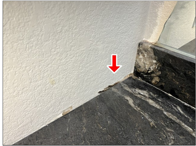
4.0 Item 12(Picture) primary bedroom bath: wall damage visible
