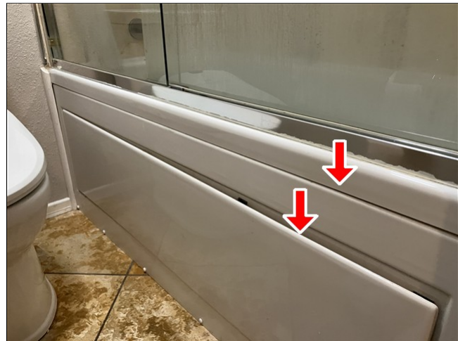
6.5 Item 2(Picture) hall bath: tub spa access cover was loose / recommend further evaluation and correction as needed
