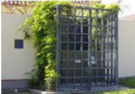
Attractive screening of mechanical equipment
