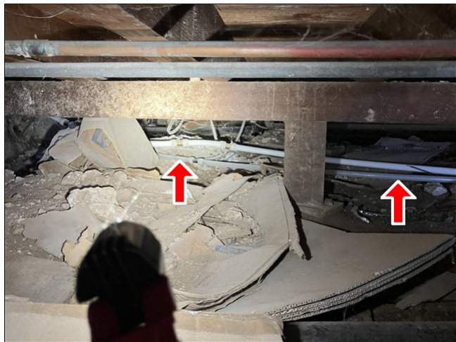
6.4 Item 1(Picture) 1819: water supply pipe was not properly strapped and supported off the ground
