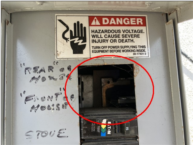
7.3 Item 1(Picture) 1819: missing breaker blank cover
