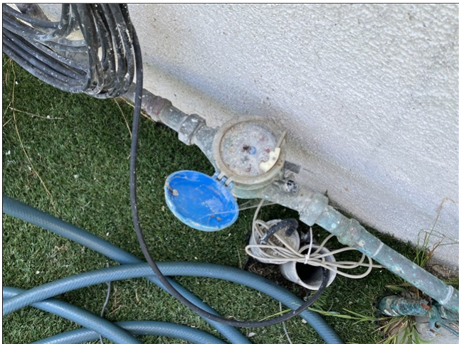
6.0 Item 3(Picture) 1817: water meter
