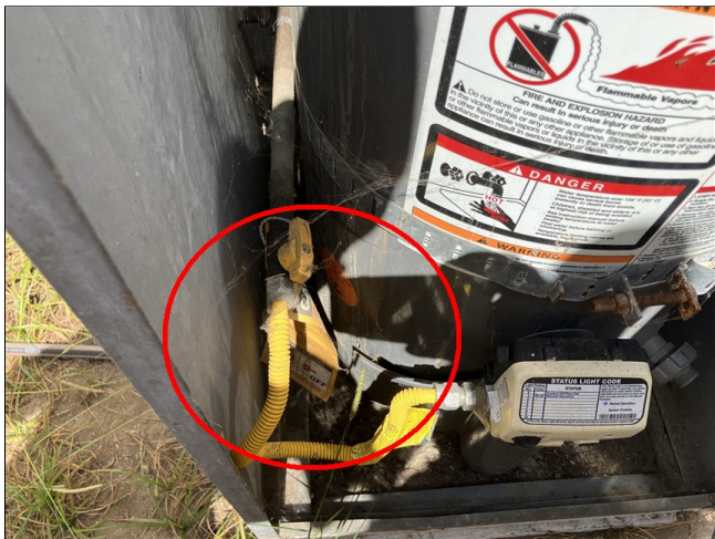
6.6 Item 5(Picture) 1819: missing sediment trap
