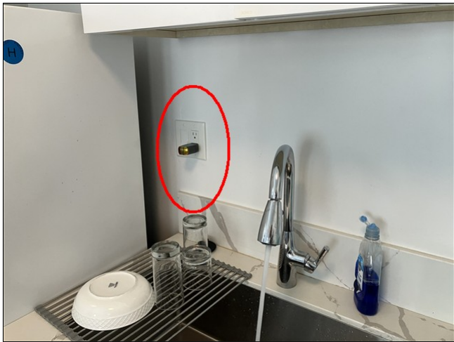
7.6 Item 2(Picture) 1819: recommend evaluation and upgrade of any non-GFCI outlets
