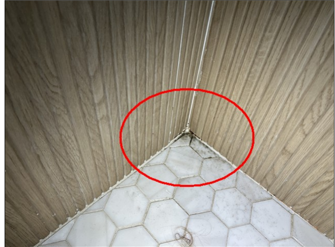
4.6 Item 2(Picture) 1819: shower surround caulking or appropriate sealant maintenance/repairs needed
