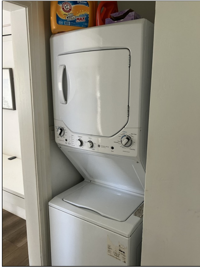
10.6 Item 1(Picture) 1819: hookups not visible for inspection
