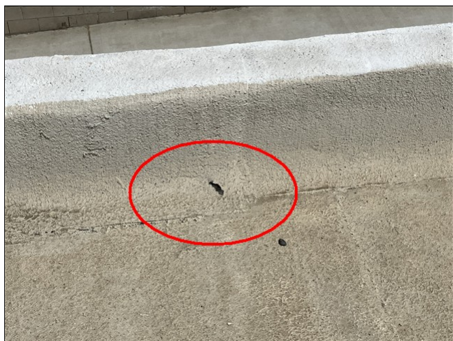
1.0 Item 3(Picture) 1819: roof covering defect/damage visible
