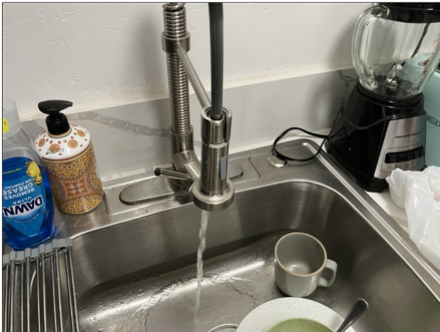
6.5 Item 1(Picture) 1817 kitchen: loose faucet / spray control button did not operate properly when tested
