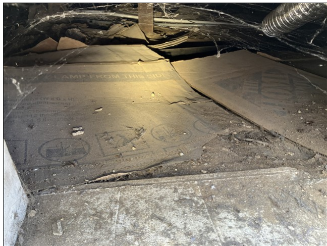
5.0 Item 4(Picture) 1819: debris visible in the subfloor area
