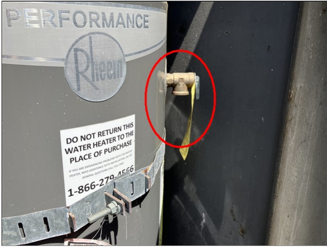
6.2 Item 4(Picture) 1819: missing TPRV drain
