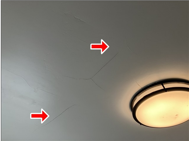
4.0 Item 1(Picture) 1819: cracks visible at ceiling
