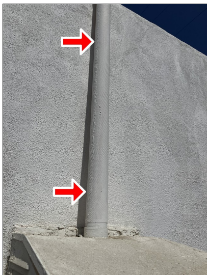
6.2 Item 6(Picture) 1819: aged vent / materials installed before 1978 may contain asbestos
