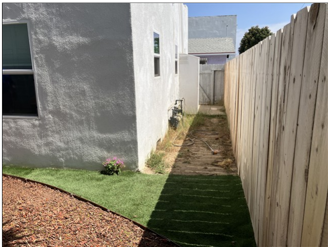
2.4 Item 2(Picture) 1819: grading or drainage improvements/corrections are recommended to achieve positive slope away from the property
