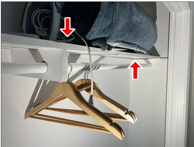
4.4 Item 1(Picture) 1819: bedroom closet shelf is leaning
