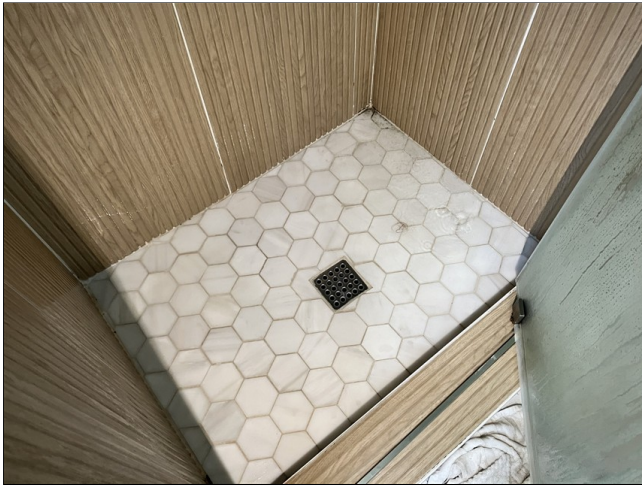
6.3 Item 4(Picture) 1819: slow drainage observed at shower / debris in drain visible
