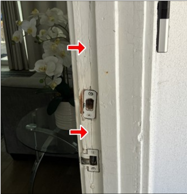
2.1 Item 1(Picture) 1819: crack visible at door jamb
