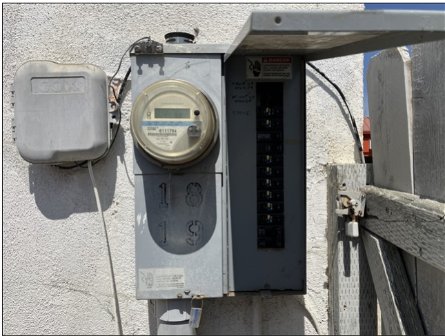
7.2 Item 1(Picture) 1819: electric meter and main disconnect
