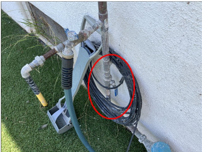
6.0 Item 4(Picture) 1817: house water shut off valve
