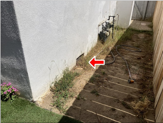
9.2 Item 4(Picture) 1819: vent appeared below grade level or was susceptible to moisture intrusion
