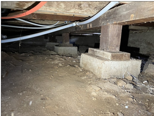
5.1 Item 2(Picture) 1817: post and pier seismic strapping/anchoring upgrades recommended
