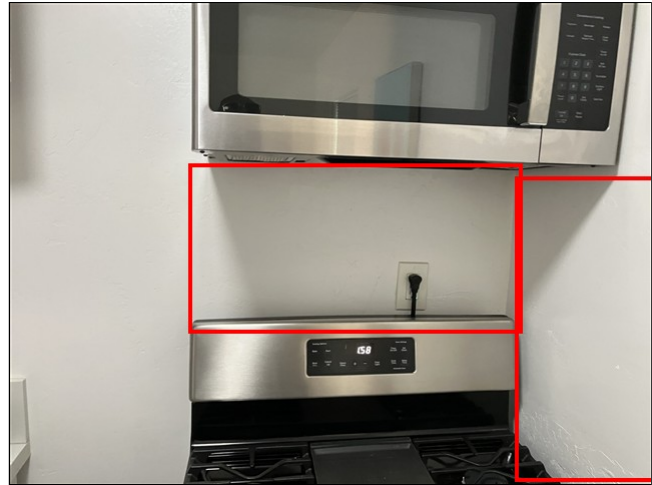
10.1 Item 4(Picture) 1817: non-combustible backsplash needed behind range ovens and stovetops
