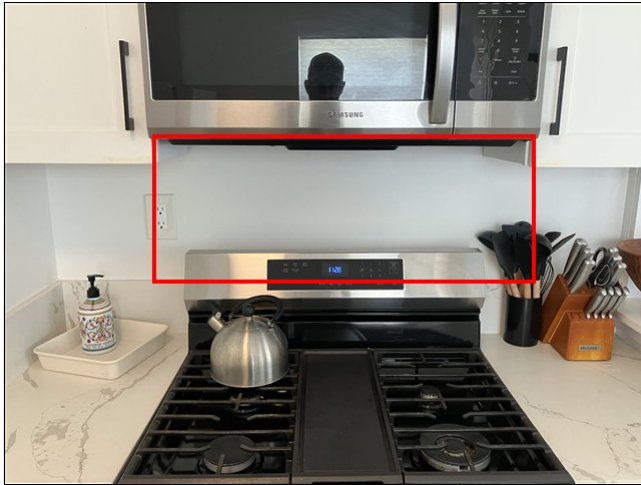
10.1 Item 3(Picture) 1819: non-combustible backsplash needed behind range ovens and stovetops
