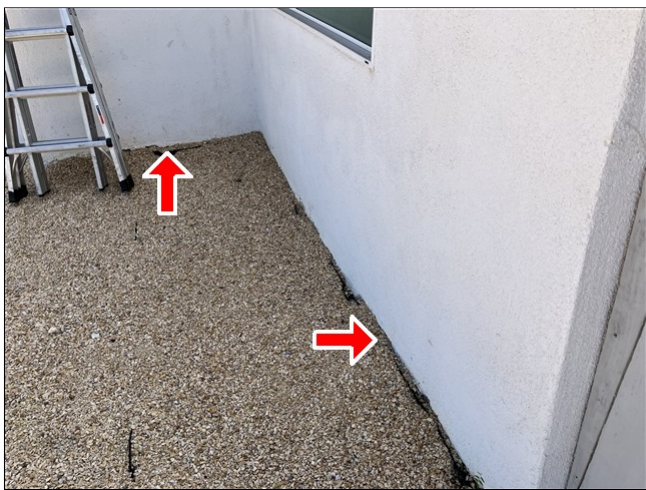
2.0 Item 2(Picture) 1819: weep screed flashing upgrades recommended
