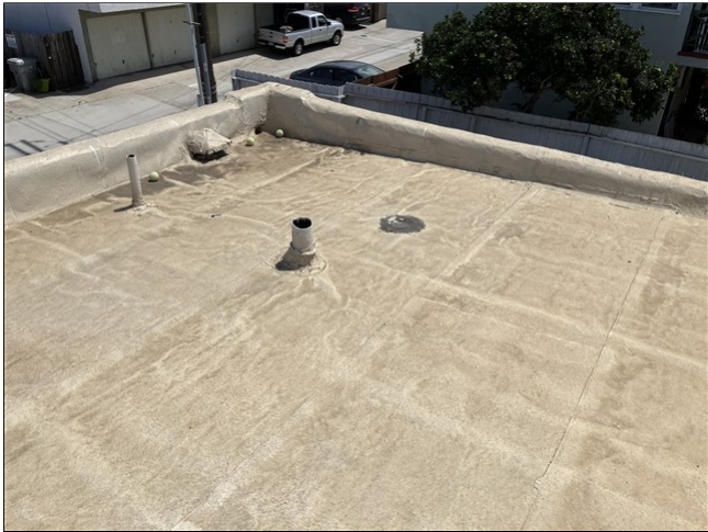
1.0 Item 5(Picture) 1817: aged roof covering / recommend further evaluation and replacement as needed
