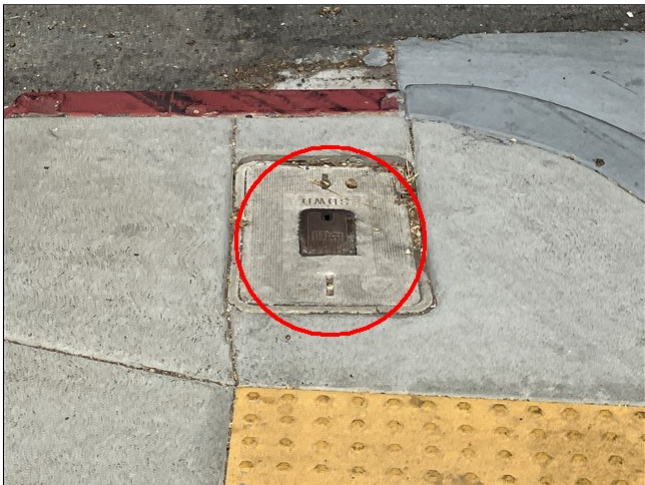
6.0 Item 2(Picture) 1817: water meter and main shut-off
