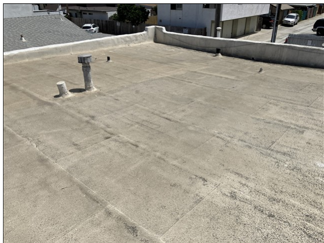
1.0 Item 1(Picture) 1819: roof covering appeared aged / recommend further evaluation
