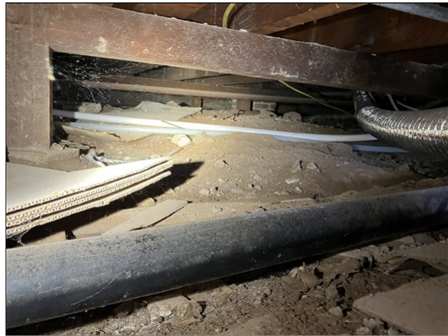
5.7 Item 1(Picture) 1819: subfloor area clearance was minimal creating limited access and/or visibility
