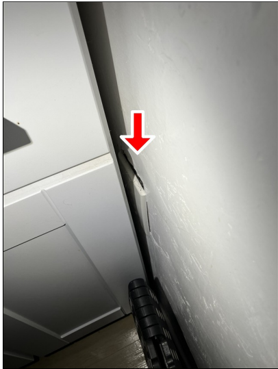
4.0 Item 4(Picture) 1817 kitchen: gap visible around outlet
