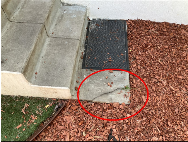
2.4 Item 4(Picture) 1817: crack visible at concrete step
