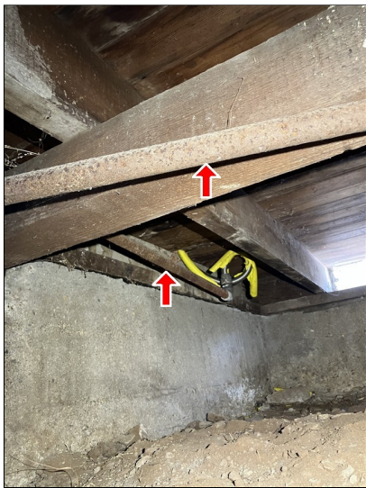
6.6 Item 2(Picture) 1817: aged gas supply pipes observed
