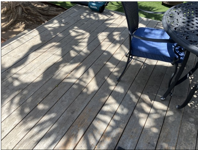
2.3 Item 3(Picture) 1819: deck boards did not appear to be protected from UV
