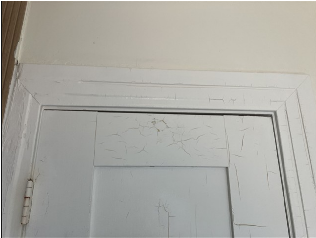
4.3 Item 1(Picture) 1819: bathroom door paint cracks/ defects visible
