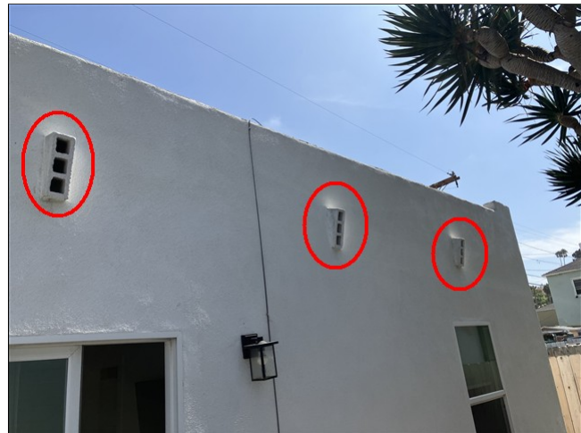
9.2 Item 2(Picture) 1819: vent screens needed at attic vents
