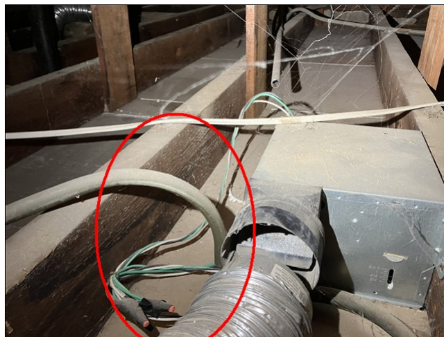
7.4 Item 4(Picture) 1817 attic: bath exhaust vent wiring was not properly installed
