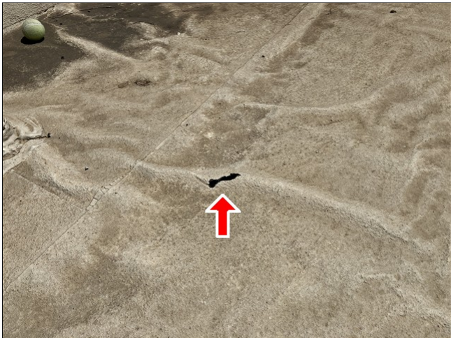
1.0 Item 7(Picture) 1817: roof covering defects visible
