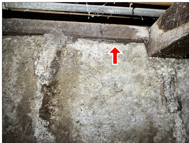
5.2 Item 2(Picture) 1819: possible WDO evidence or damage observed
