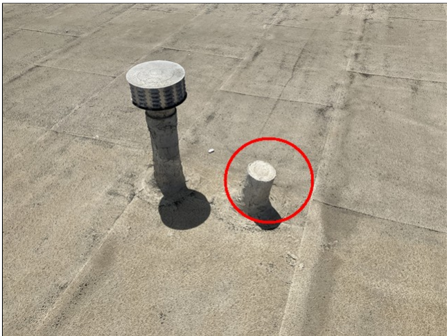
1.5 Item 2(Picture) 1819: vent termination was covered / recommend further evaluation
