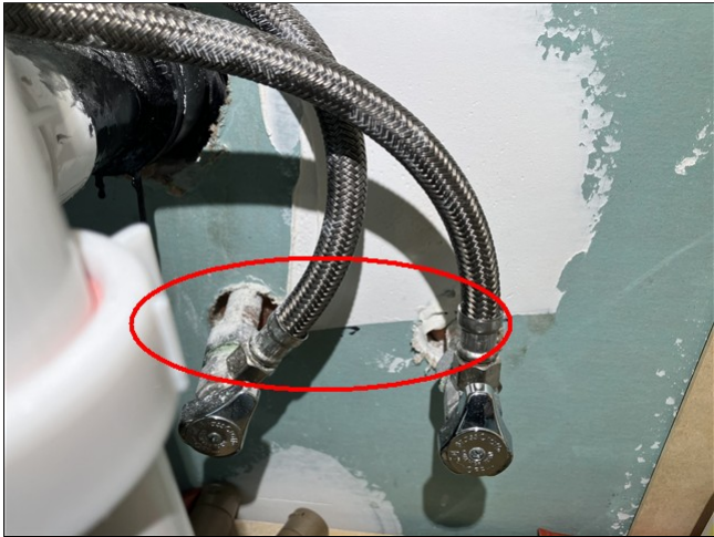
4.0 Item 3(Picture) 1819: bathroom sink wall penetrations visible
