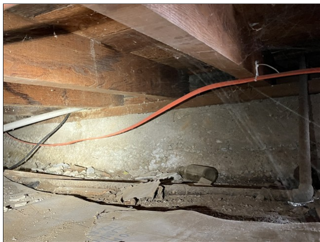
5.0 Item 3(Picture) 1819: foundation anchoring upgrades recommended
