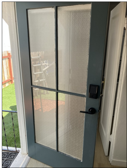
2.6 Item 2(Picture) 1817: recommend evaluation and upgrade of any non-safety glass windows at appropriate locations
