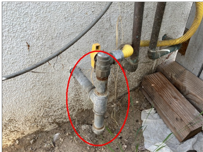
6.6 Item 6(Picture) 1817: improper sediment trap configuration
