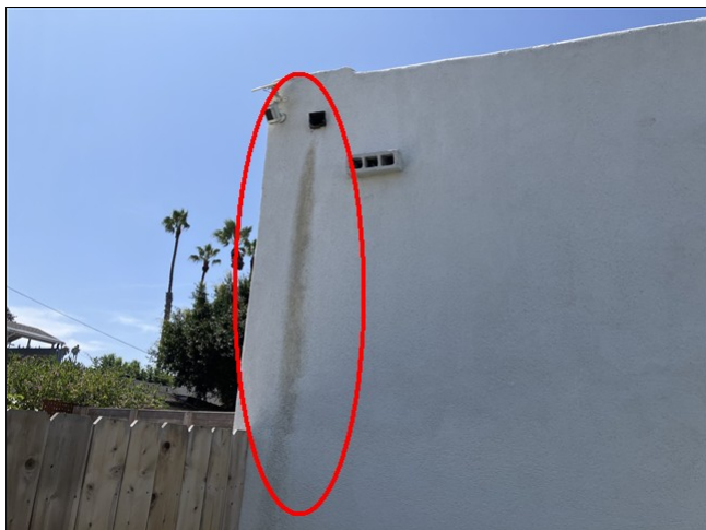
1.1 Item 1(Picture) rain gutter upgrades recommended
