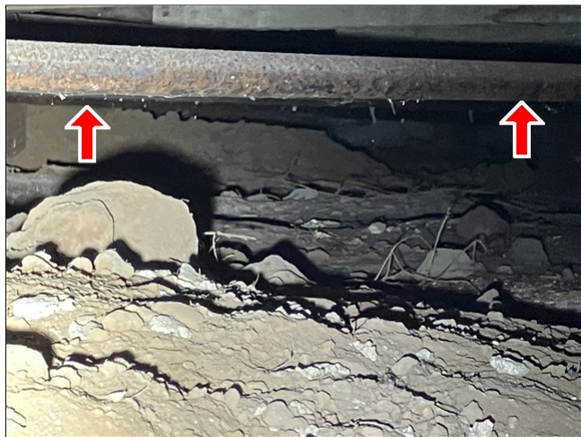
6.6 Item 3(Picture) 1819: aged gas supply pipes observed
