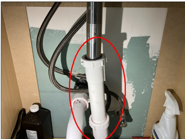
6.3 Item 6(Picture) 1819: bathroom sink drain was not installed properly
