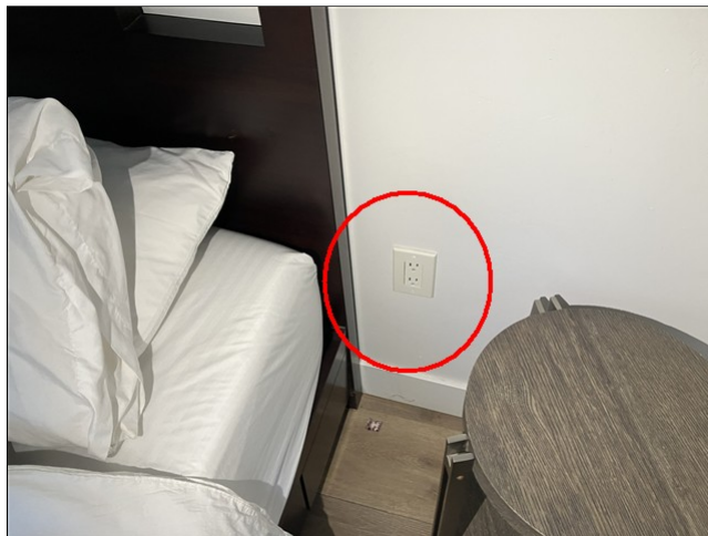
7.5 Item 2(Picture) 1819 bedroom: loose outlet
