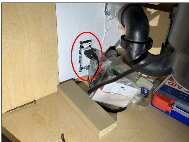
7.5 Item 5(Picture) 1817 kitchen: missing outlet cover
