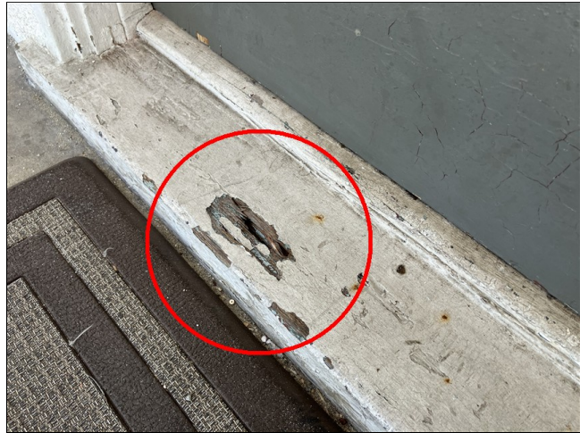
2.1 Item 2(Picture) 1819: possible WDO evidence or damage observed at door threshold
