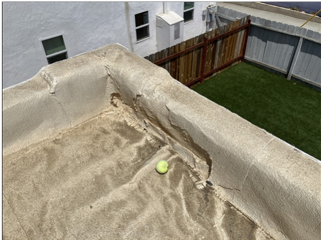
1.0 Item 8(Picture) 1817: roof covering defects visible
