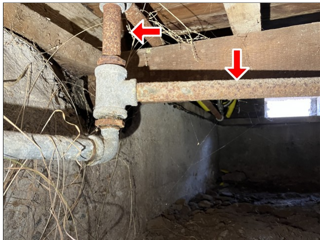
6.6 Item 1(Picture) 1817: aged gas supply pipes observed
