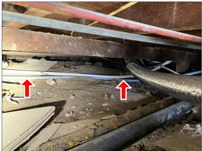
6.4 Item 2(Picture) 1819: water supply pipe was not properly strapped and supported off the ground
