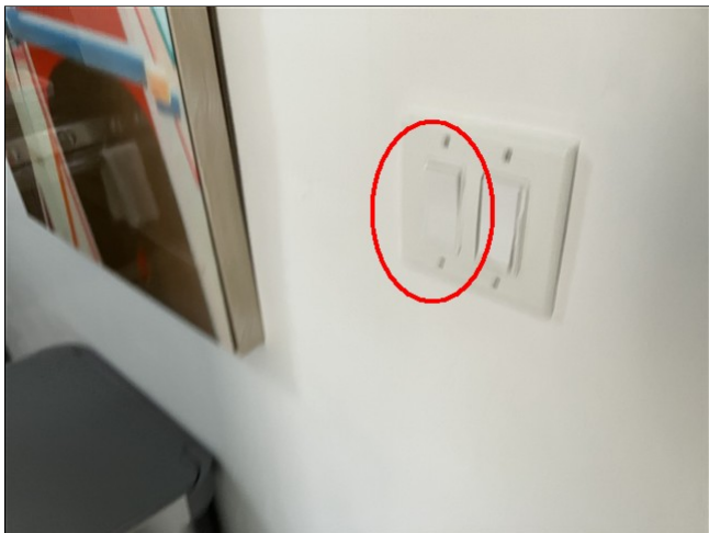
7.5 Item 7(Picture) 1817: switch and corresponding fixture or outlet were not identified
