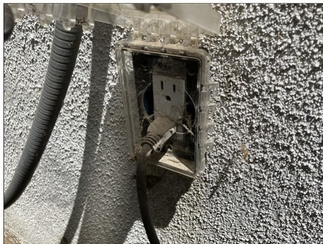
7.6 Item 4(Picture) 1817: recommend evaluation and upgrade of any non-GFCI outlets
