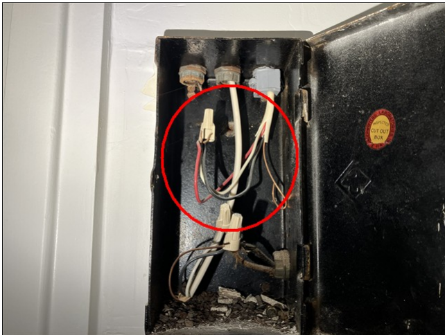
7.4 Item 1(Picture) 1819 bedroom closet: recommend further evaluation of exposed wire ends / box should be secured with a fastener
