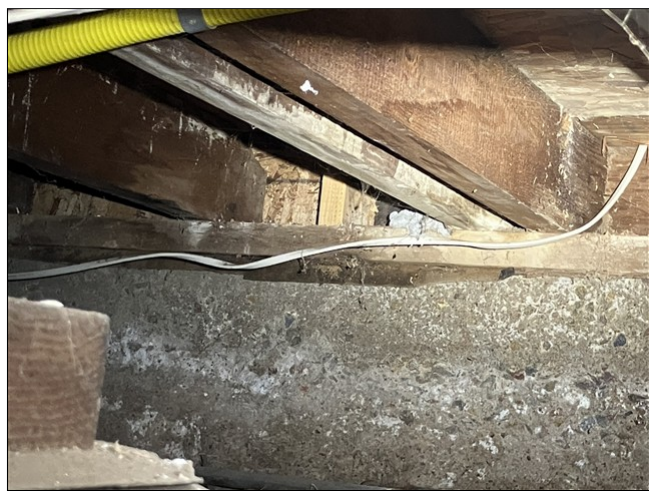
5.0 Item 2(Picture) 1817: foundation anchoring upgrades recommended
