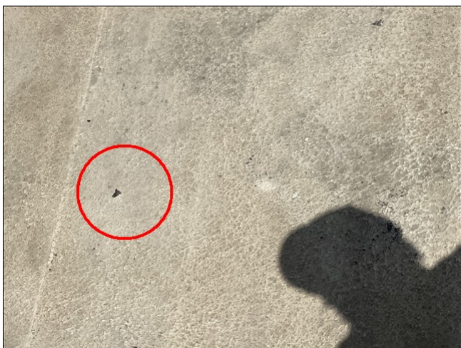
1.0 Item 4(Picture) 1819: roof covering damage/defect visible
