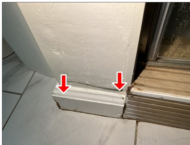
4.6 Item 5(Picture) 1819 bath: moisture stains or damage visible
