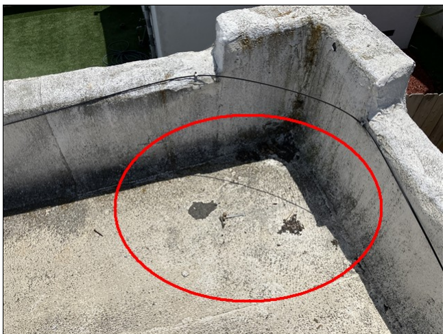
1.0 Item 2(Picture) 1819: roof covering appeared aged / recommend further evaluation
