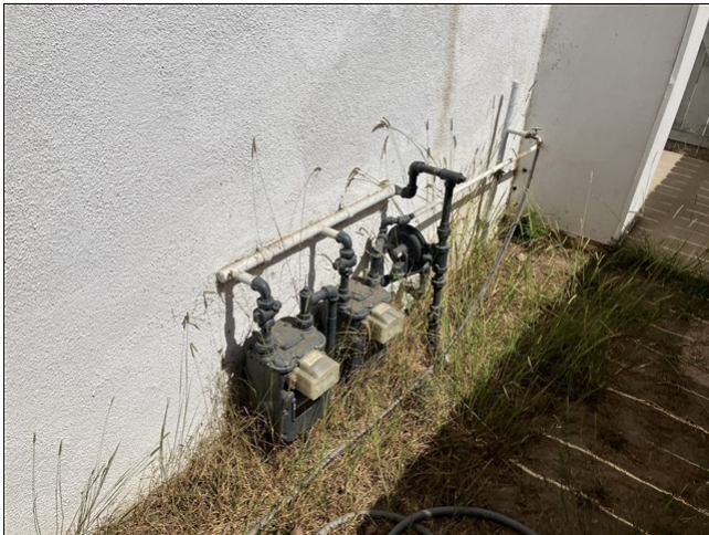
6.1 Item 1(Picture) gas meter and shut-off valve
