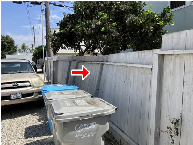
2.6 Item 1(Picture) leaning fence next to driveway
