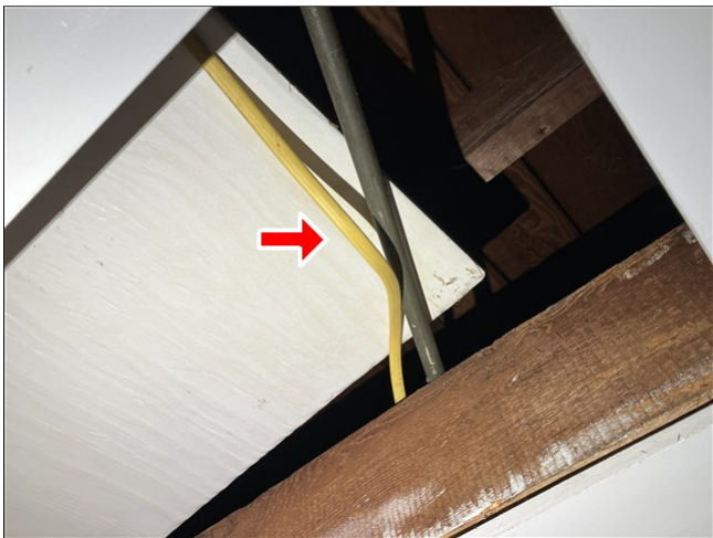
9.3 Item 1(Picture) 1817: wiring should not cross over access to attic
