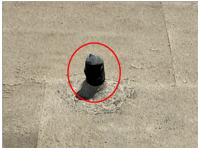
1.5 Item 1(Picture) 1819: vent termination was covered / recommend further evaluation
