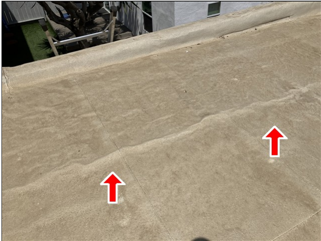
1.0 Item 9(Picture) 1817: roof covering defects visible
