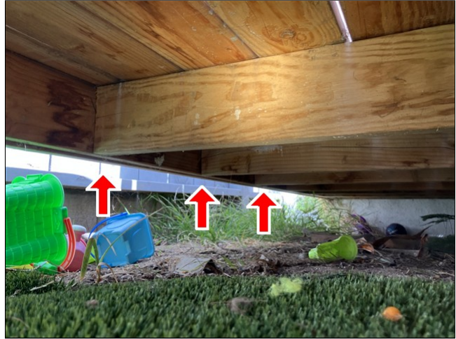
2.3 Item 2(Picture) 1819: missing deck joist hangers
