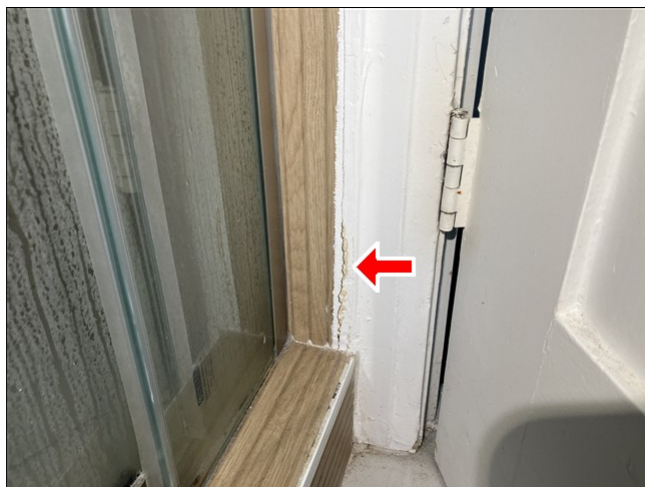
4.6 Item 4(Picture) 1819 bath: moisture stains or damage visible
