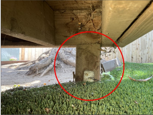
2.3 Item 1(Picture) 1819: substandard deck installation or building material was observed / recommend further evaluation
