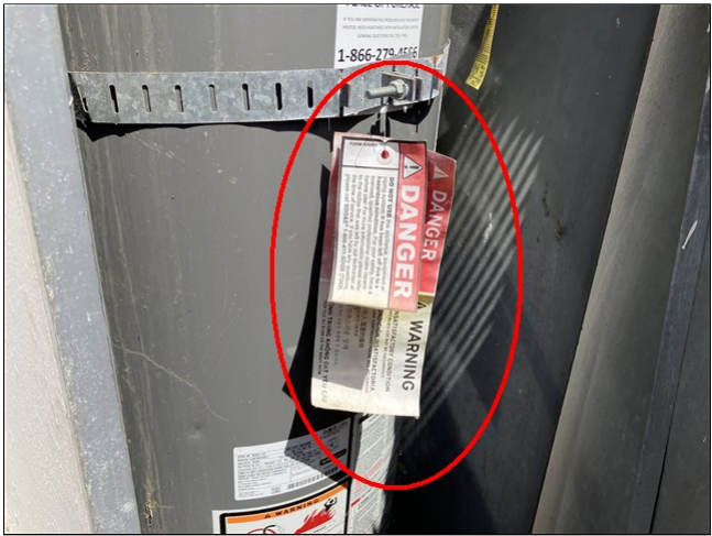
6.2 Item 2(Picture) 1819: recommend further evaluation of "danger tag"
