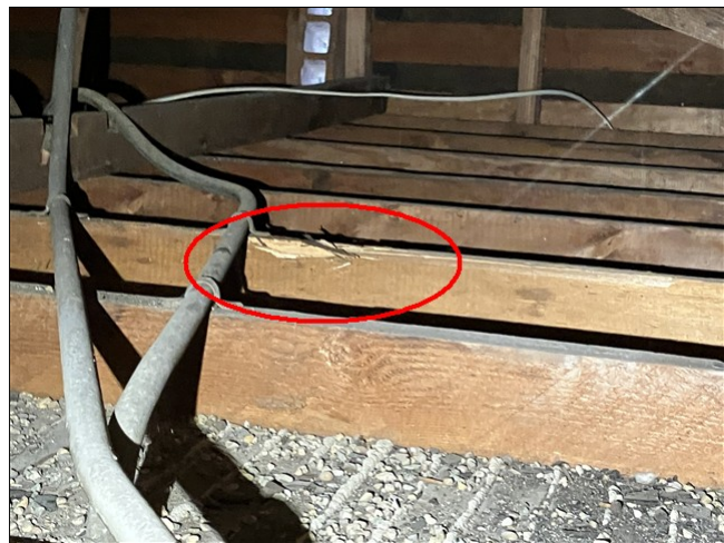
5.5 Item 1(Picture) 1819 attic: possible WDO evidence or damage observed
