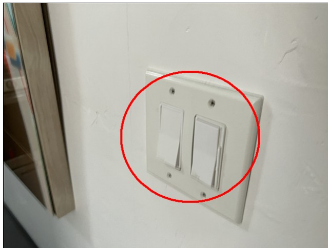
7.5 Item 4(Picture) 1817 kitchen: loose switch cover
