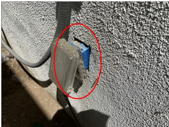
7.5 Item 3(Picture) 1817: loose exterior outlet
