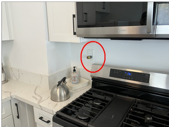
7.6 Item 3(Picture) 1819: recommend evaluation and upgrade of any non-GFCI outlets
