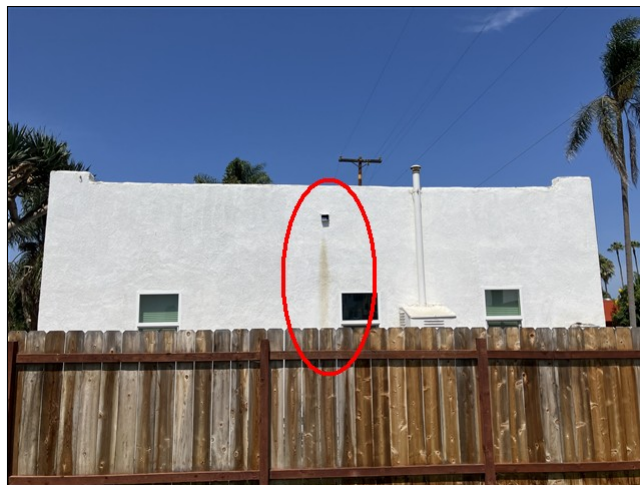
1.1 Item 2(Picture) rain gutter upgrades recommended
