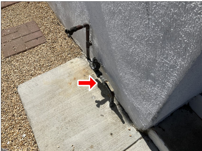
6.0 Item 1(Picture) 1819: house water shut off valve
