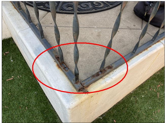
2.3 Item 4(Picture) 1817: oxidation visible at railing
