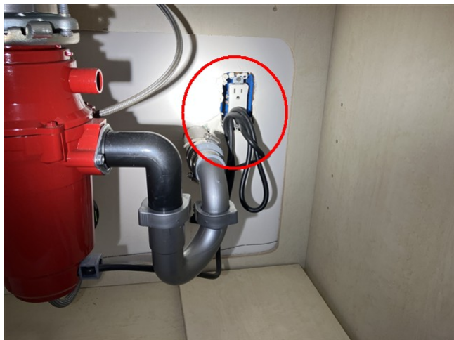
7.5 Item 1(Picture) 1819 kitchen: missing outlet cover
