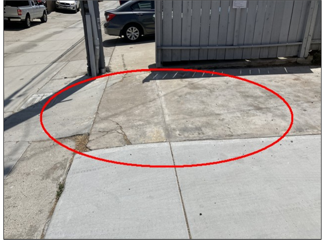
2.4 Item 5(Picture) cracks visible at driveway
