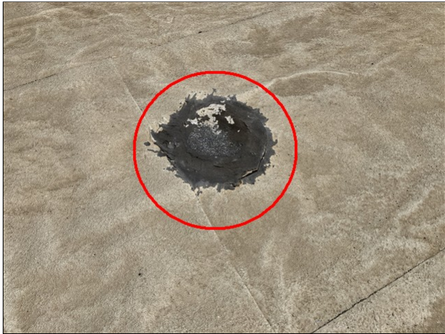
1.0 Item 6(Picture) 1817: roof covering defects visible
