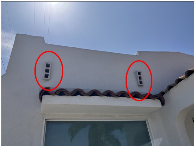
9.2 Item 1(Picture) 1819: vent screens needed at attic vents
