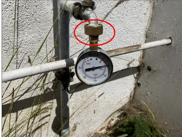
6.4 Item 5(Picture) 1819: missing vacuum breaker
