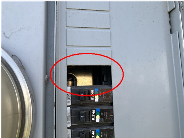
7.3 Item 2(Picture) 1817: missing breaker blank cover
