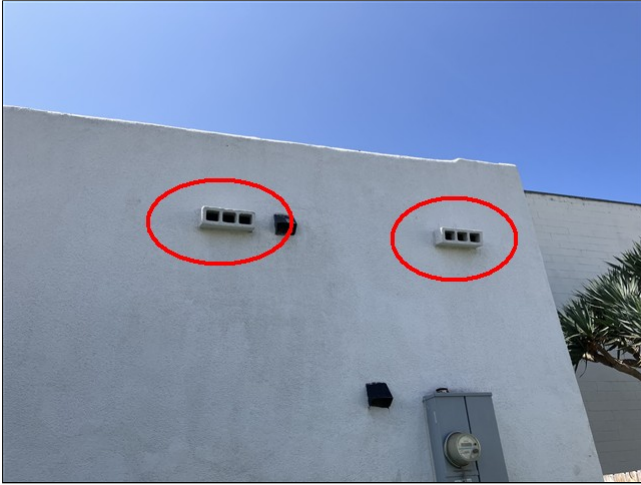
9.2 Item 3(Picture) 1817: vent screens needed at attic vents
