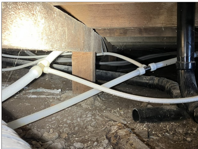
5.1 Item 3(Picture) 1819: post and pier seismic strapping/anchoring upgrades recommended
