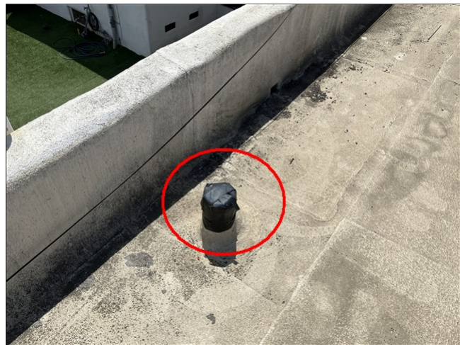
1.5 Item 3(Picture) 1819: vent termination was covered / recommend further evaluation and correction as needed
