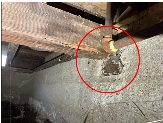
5.2 Item 1(Picture) 1817: possible WDO evidence or damage observed floor beam
