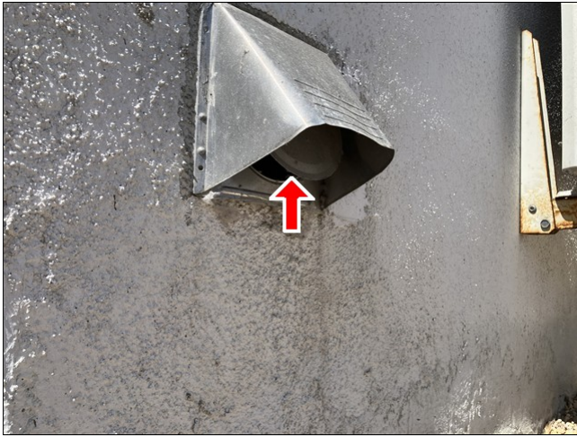
9.1 Item 1(Picture) 1819: lint debris removal for damper to fully close
