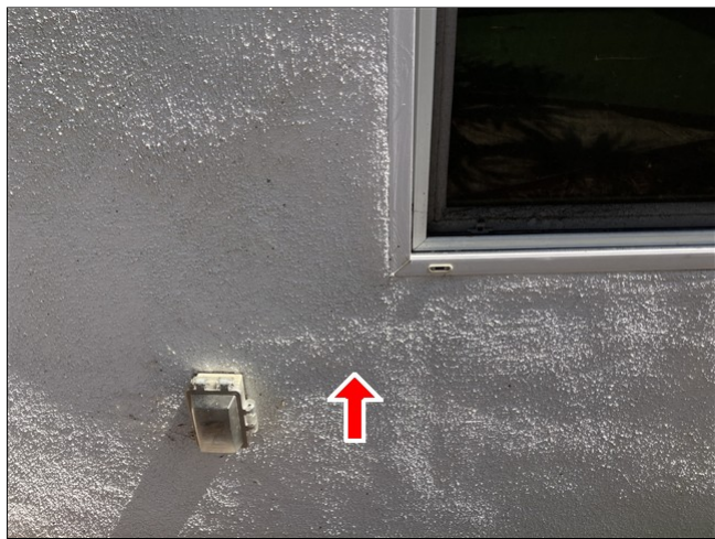
2.0 Item 3(Picture) 1819: crack visible at stucco
