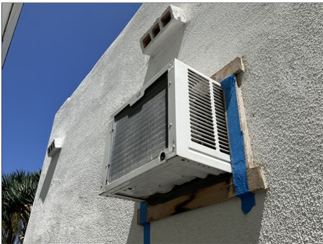
8.4 Item 3(Picture) 1817: wall a/c unit
