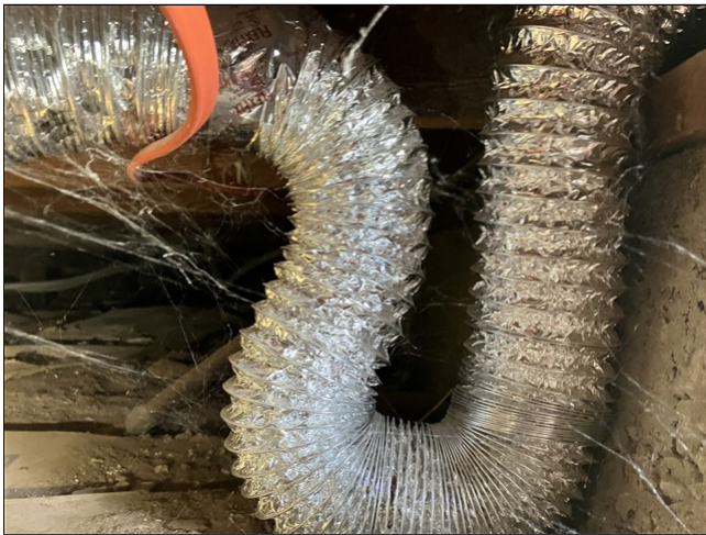
9.1 Item 2(Picture) 1819: dryer ducting material upgrade recommended
