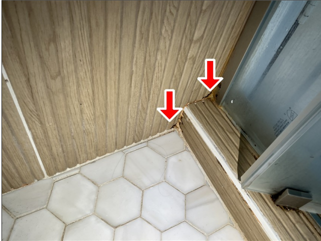
4.6 Item 1(Picture) 1819: shower surround caulking or appropriate sealant maintenance/repairs needed
