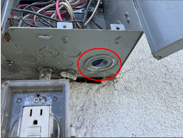
7.3 Item 3(Picture) 1817: missing knockout plug
