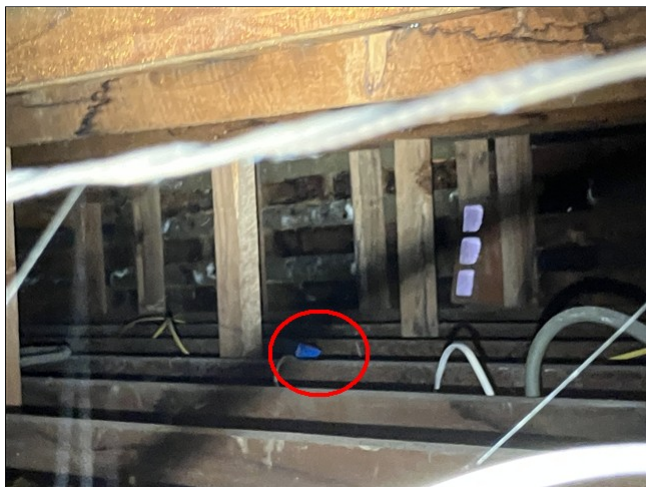
7.4 Item 3(Picture) 1819 attic: missing junction box cover
