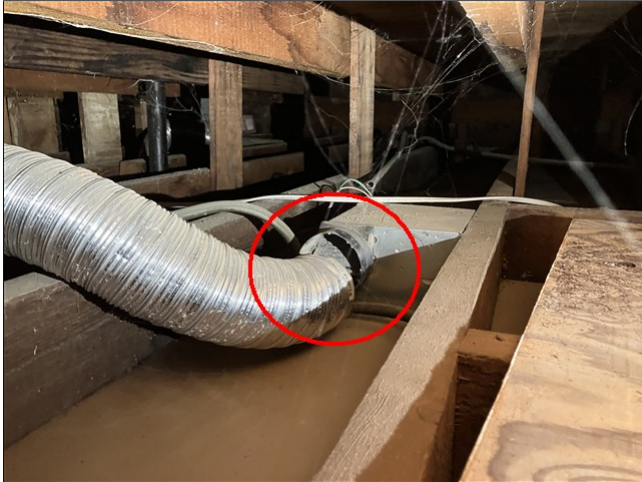
9.1 Item 3(Picture) 1817 attic: bath exhaust vent duct disconnected
