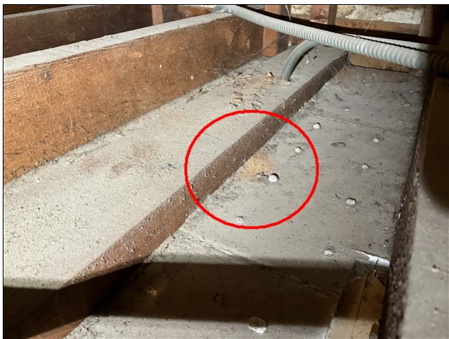
5.5 Item 2(Picture) 1817 attic: possible WDO evidence or damage observed
