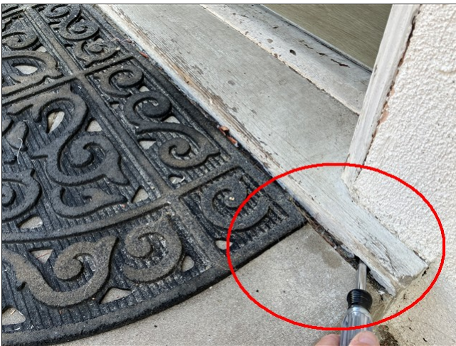
2.1 Item 3(Picture) 1817: possible WDO evidence or damage observed
