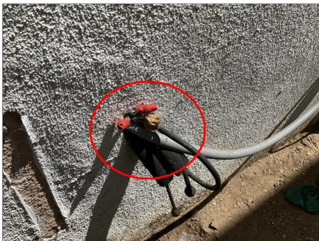
7.4 Item 5(Picture) 1817: recommend further evaluation abandoned materials
