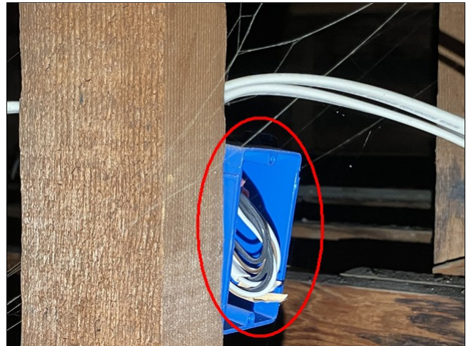
7.4 Item 2(Picture) 1819 attic: missing junction box cover
