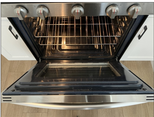
10.1 Item 2(Picture) 1819: missing anti-tip bracket
