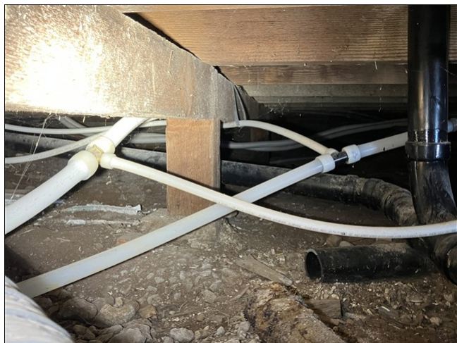
6.4 Item 3(Picture) 1819: water supply pipe was not properly strapped and supported
