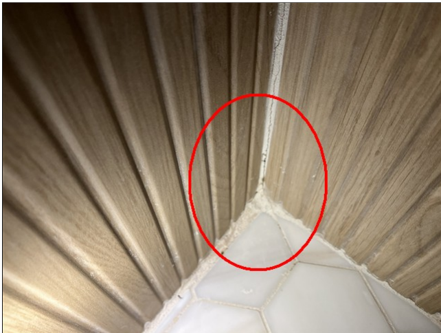
4.6 Item 3(Picture) 1819: shower surround caulking or appropriate sealant maintenance/repairs needed
