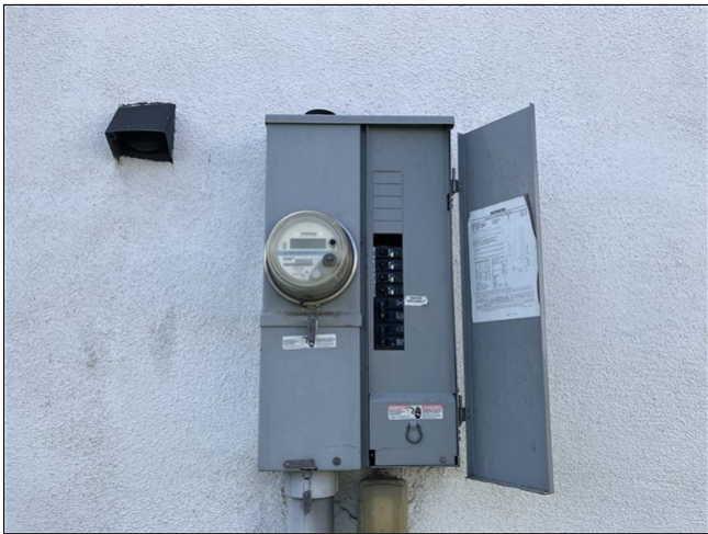
7.2 Item 2(Picture) 1817: electric meter and main disconnect
