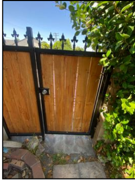
Gate not latching properly - recommend servicing
