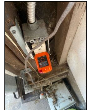
Outlet cover missing - needs to be serviced
