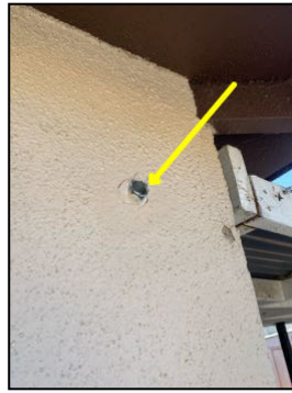
Cracking/chipping/holes - needs to be serviced
