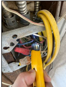
Exposed live wires - needs to be serviced/evaluated by a licensed electrician immediately
