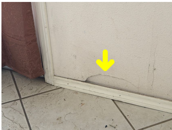
The walls or ceiling have cosmetic damage, which you may wish to view for yourself.
