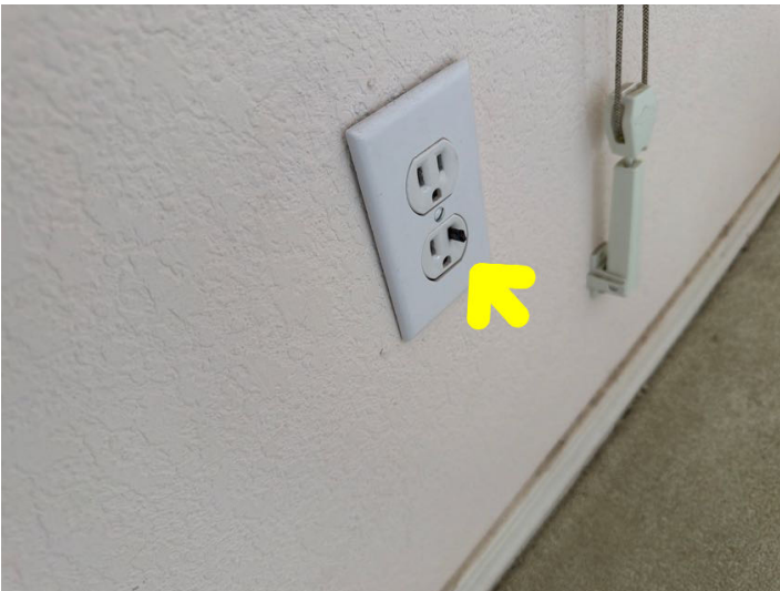
One or more outlets have an obstruction within, and should be evaluated and serviced by a licensed electrical contractor.
