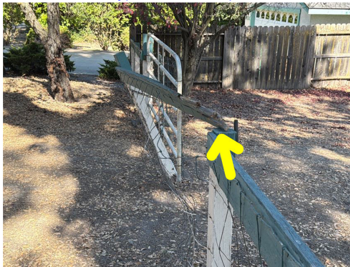
The fences have damage that you may wish to have repaired.
