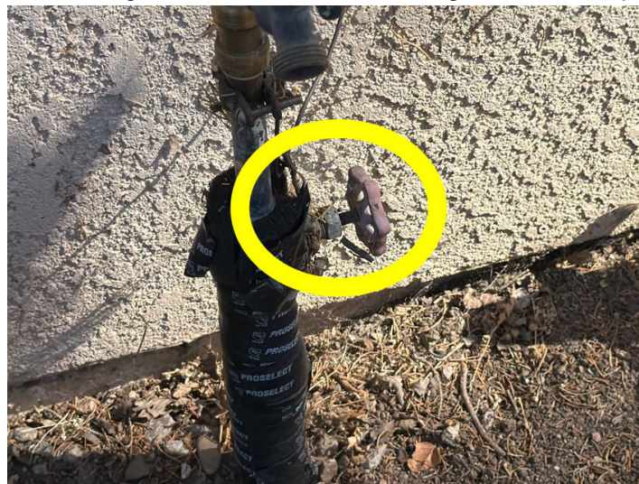
The main water shutoff valve is an older 'Gate' style valve. This older valve may no longer properly function. We recommend it be upgraded to a newer 'Ball' valve.
