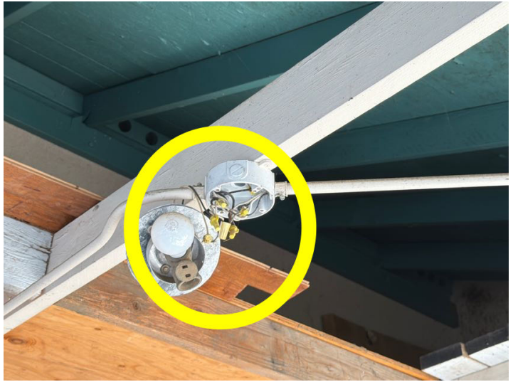
An exterior light is not properly secured or is loosely installed and should be serviced.
