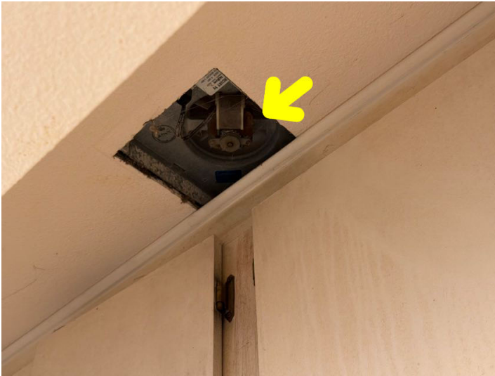
An exhaust fan is missing its cover and should be serviced.
