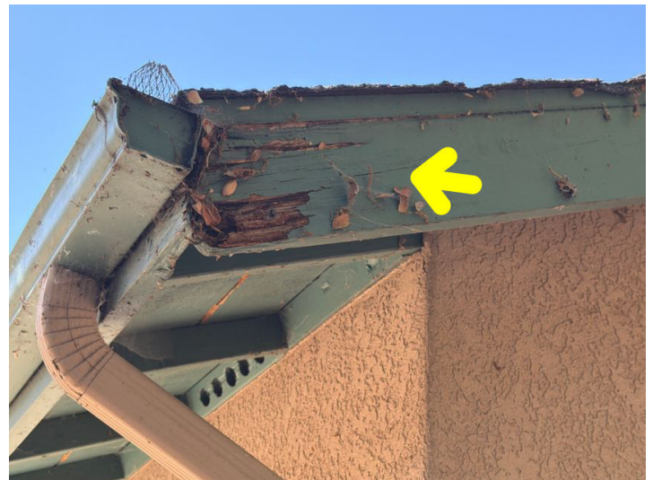
There is damage to the wood trim, fascia, and/or eaves that should be evaluated by a pest inspector.
