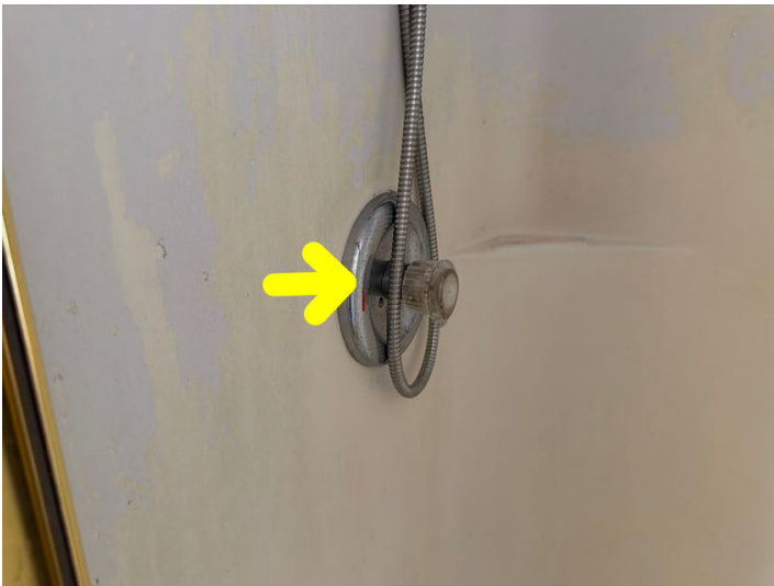
The shower valve handle is loose and should be serviced.
