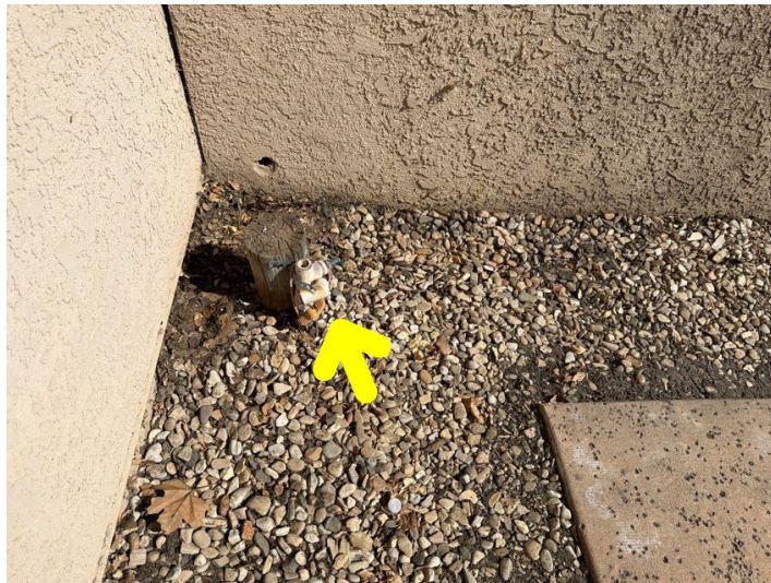
A hose bib on the rear is not functional or has been abandoned.
