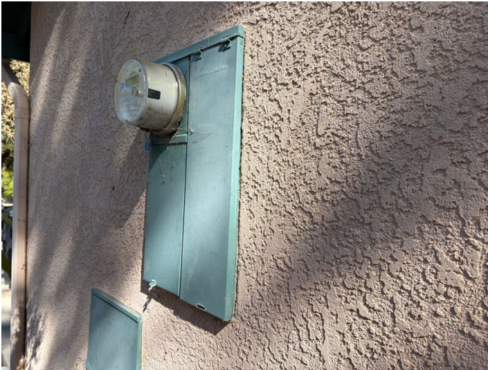
The residence is served by a 100 amp main electrical panel, located at the right side of the home or unit.
