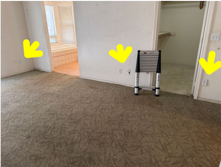
One or more outlets have an open-neutral, and should be evaluated and serviced by a licensed electrical contractor.
