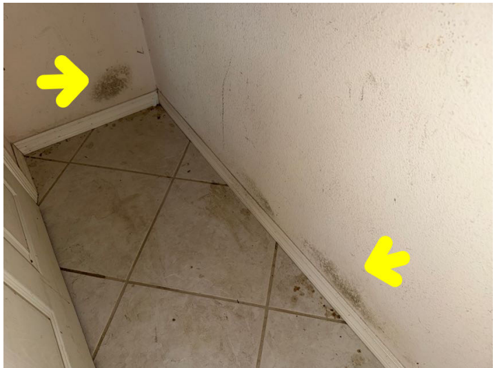
There is a mold-like substance present, which should be evaluated by a specialist and serviced as necessary. All molds flourish in a damp environment and many are commonplace, but some are toxic and may represent a health threat.
