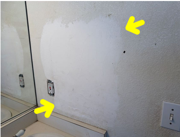
There has been a drywall repair that should be explained by the seller.
