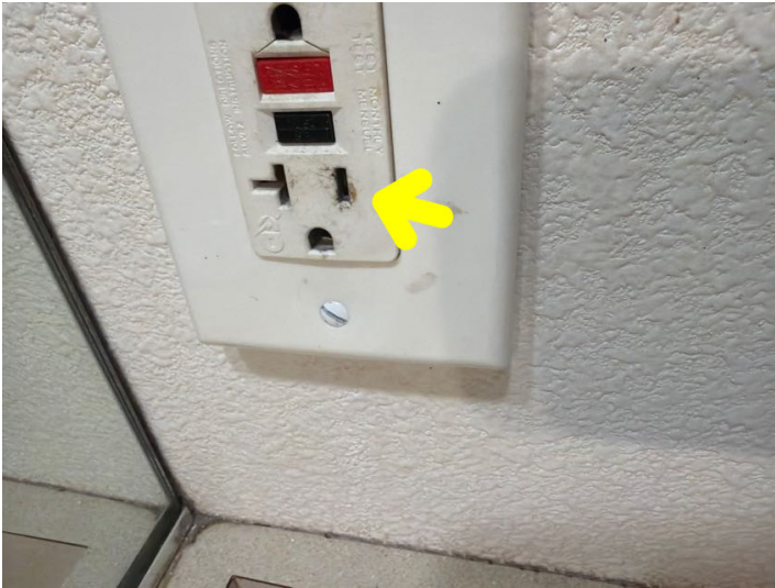
One or more bathroom sink outlets are damaged, and should be evaluated and serviced by a licensed electrical contractor.
