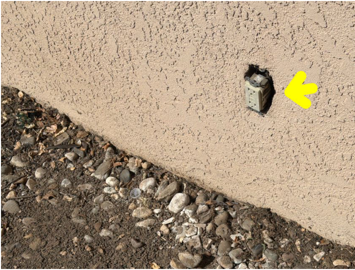
One or more outlets at the rear are not secure and should be evaluated and serviced by a licensed electrical contractor.
