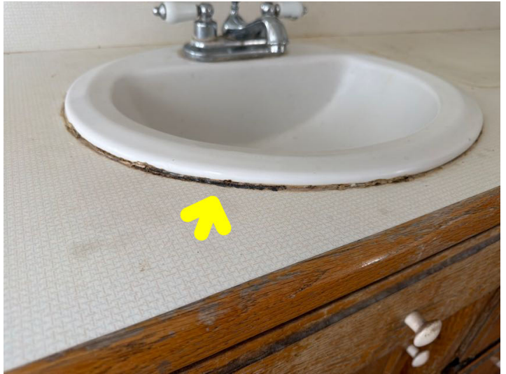
There is a separation between the sink and the countertop, which should be sealed to forestall moisture intrusion.
