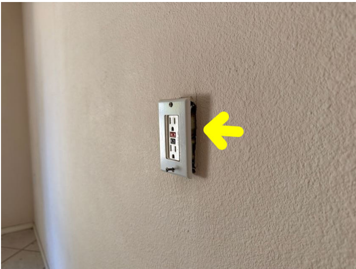
A GFCI outlet did not trip when activated and should be repaired or replaced by a licensed electrical contractor.
