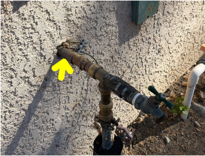
A hose bib on the right side is not fully secured and should be serviced by a qualified plumbing contractor.
