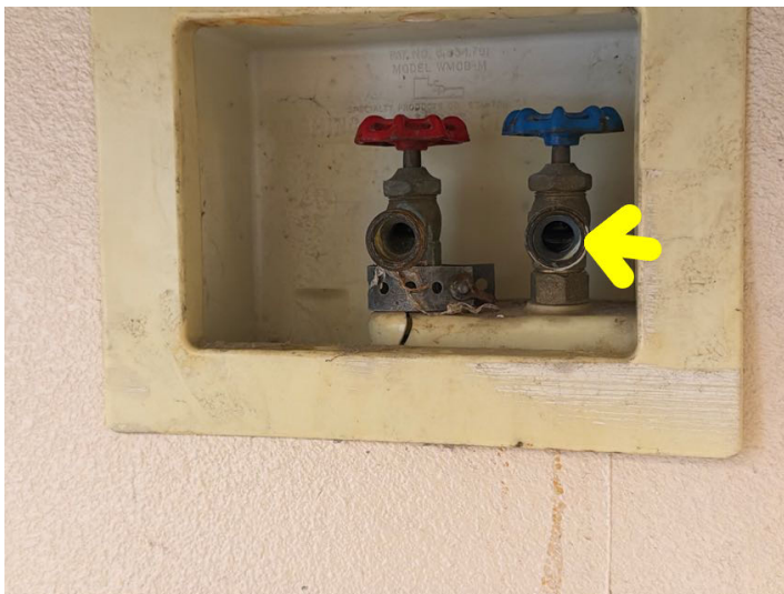
A water supply pipe or fitting is leaking and should be evaluated and serviced by a qualified plumbing contractor.
