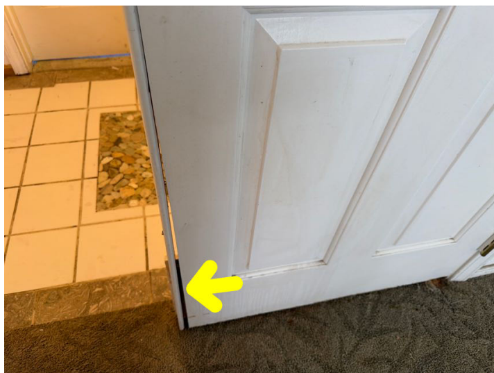
The entry door is damaged and should be serviced.
