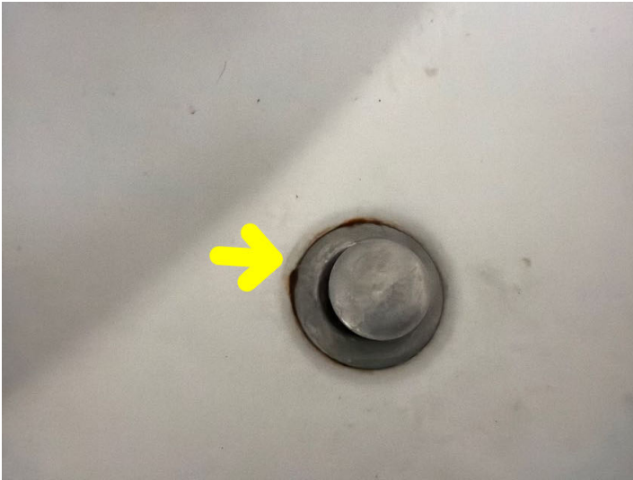
The bathroom sink has rusted at the drain or overflow inlet. It is not leaking, but will obviously be susceptible to leaks.
