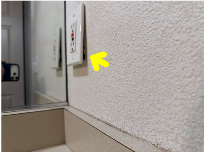
One or more bathroom sink outlets are not secure, and should be evaluated and serviced by a licensed electrical contractor.
