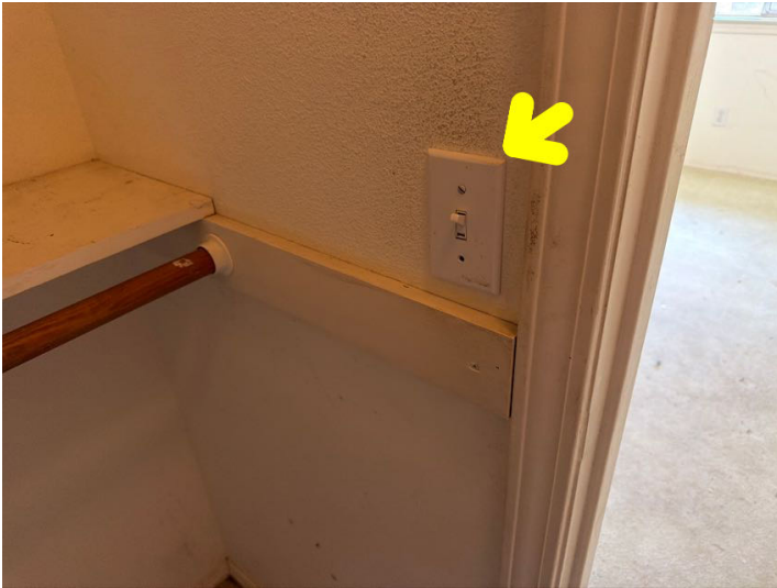
One or more light switches are not secure, and should be evaluated and serviced by a licensed electrical contractor.
