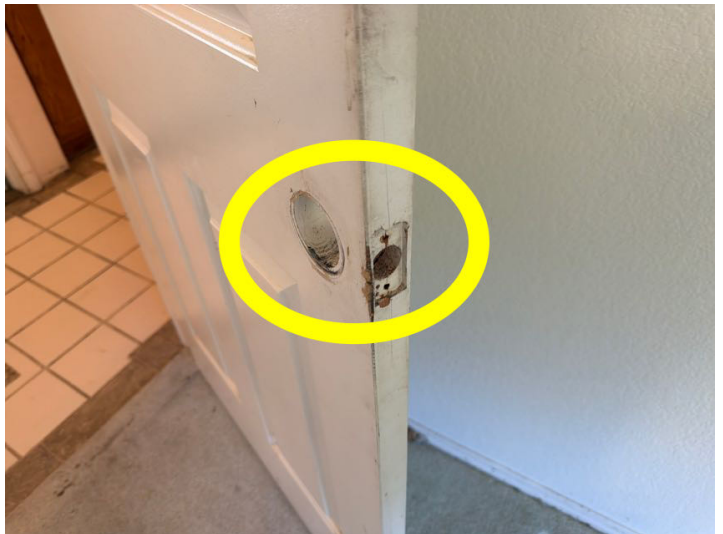
The entry door handle and hardware are missing and should be serviced.
