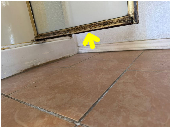
The shower door seal is missing or damaged, and should be serviced.
