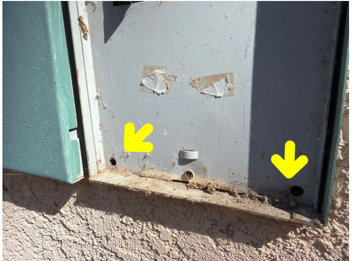
The interior panel cover is missing one or more of its fasteners or screws and should be serviced.
