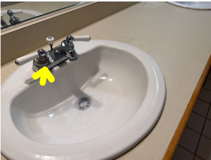
The sink faucets leak around the stem while in use, and should be repaired.
