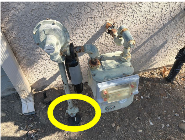
The gas main shut-off is located on the right side of the home, unit or building.
