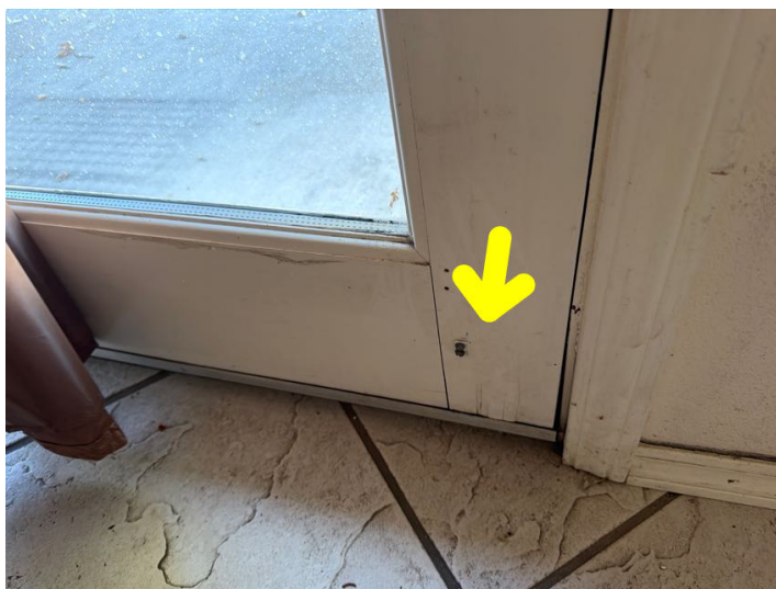
An exterior door has moisture damage, and should be evaluated by a pest inspector.
