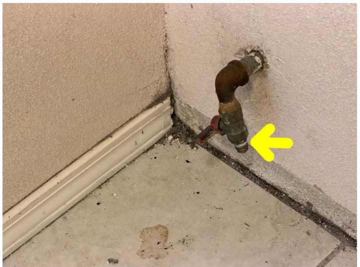
There is no cap on the gas valve. The gas valve should be capped when not in use.
