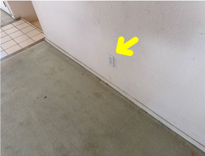
One or more outlets have an open-neutral, and should be evaluated and serviced by a licensed electrical contractor.
