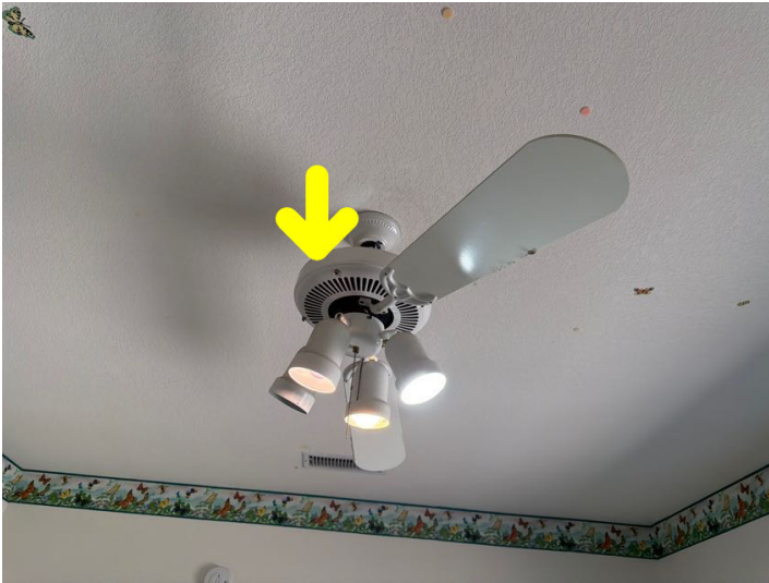
The ceiling fan is damaged and should be serviced.
