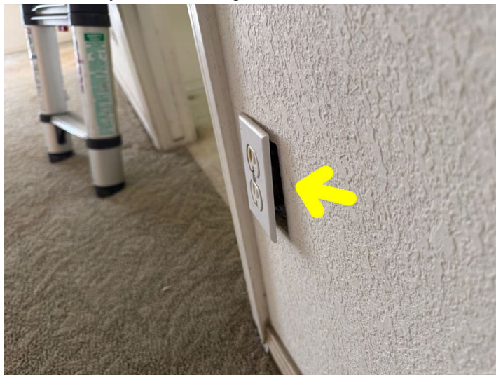
One or more outlets are not secure, and should be evaluated and serviced by a licensed electrical contractor.
