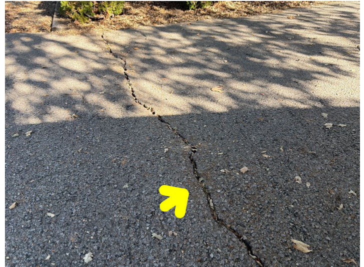
The driveway is damaged or has deteriorated and should be repaired.
