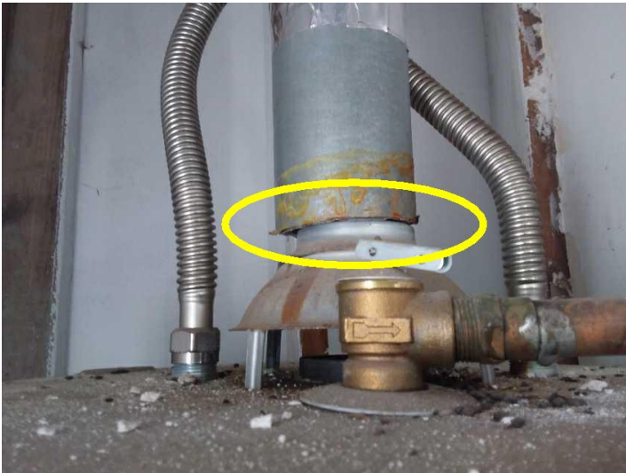
The vent pipe is disconnected and will not effectively draft the bi-products of combustion beyond the residence, and should be serviced.
