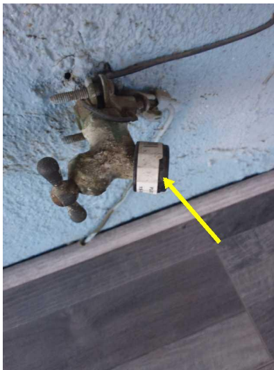
A hose bib has been capped which implies it might be dripping, which you may want to have evaluated.
