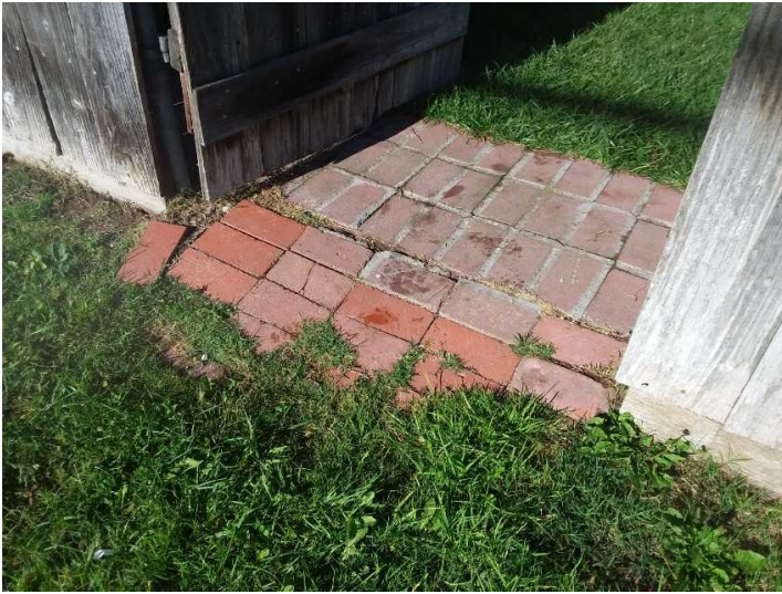
The paver patio or walkway has multiple offsets. This may be due to unsuitable soil below the pavers.
