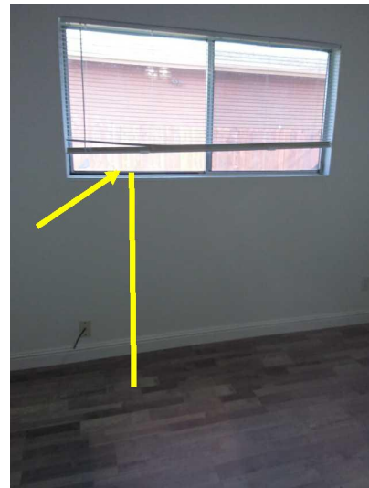
A window is too high or too small to facilitate an emergency exit or egress. Bedroom windows should measure 24" high by 20" wide, with an optimum sill height of 44", to facilitate an emergency exit by the occupant and an emergency egress for a fire person wearing breathing apparatus.
