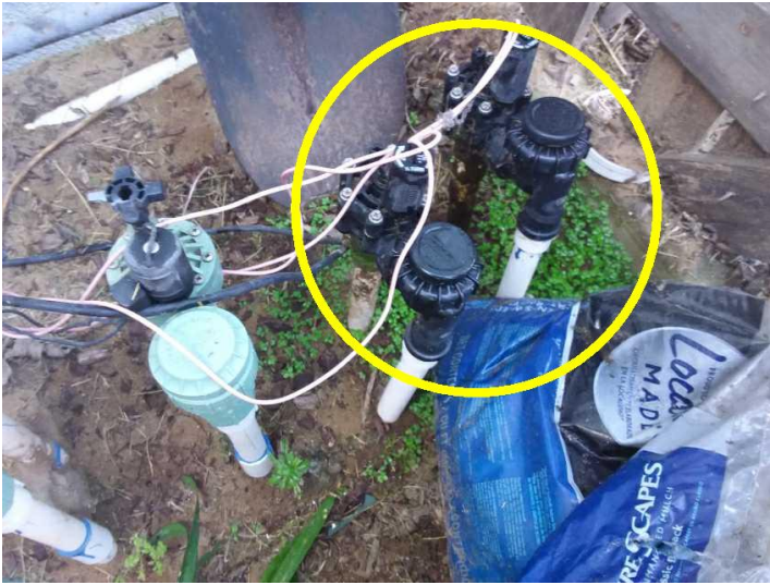
A sprinkler valve located at the right side is leaking and should be repaired.
