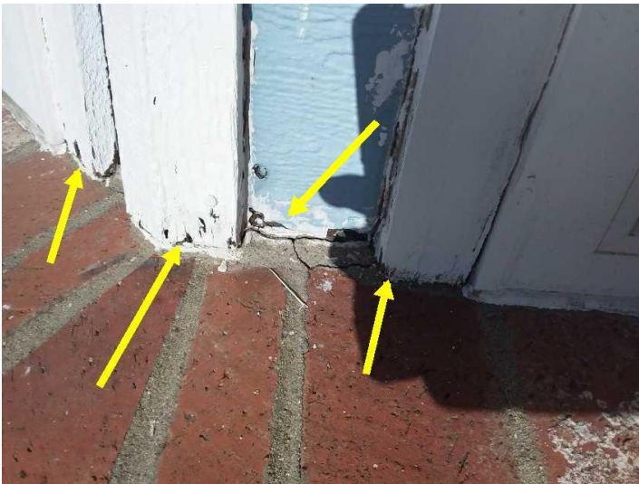
Portions of the wood siding are dry rot or moisture damaged, and should be evaluated by a termite inspector.
