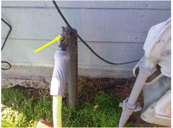
A hose bib at the right side leaks when activated and should be serviced.
