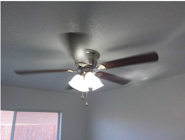
The ceiling fan is functional but rocks at high speeds and should be serviced so the fan operates smoothly.
