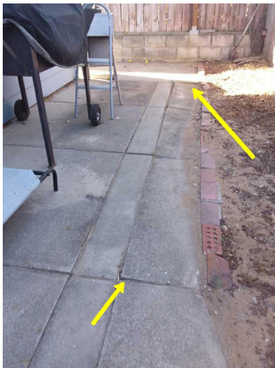
There is one or more offsets in the walkways that could prove to be trip-hazards.
