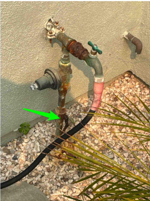
Main water shut off valve
