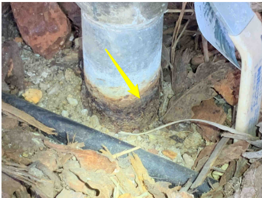
Some rust and deterioration noted at areas of the unprotected gas pipe at dirt level
