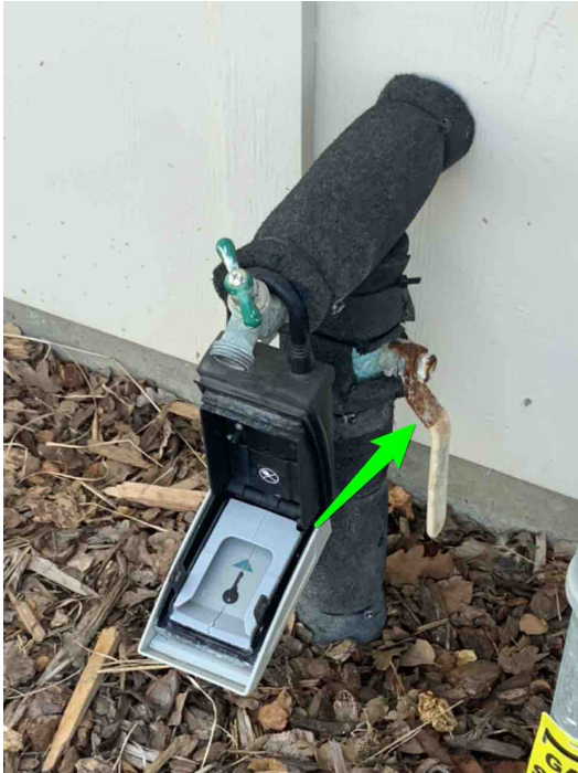
Main water shut off valve
