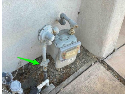
Main gas shut off valve
