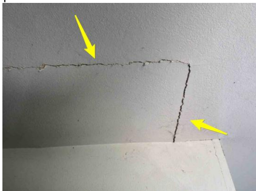
Example. In the garage over the water heater
