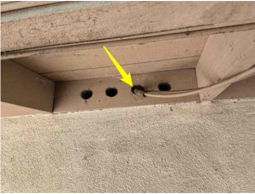
Unprotected openings can lead to bird or bat intrusion
