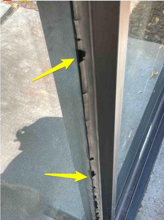
152: Damaged weatherstripping at the exterior sliding glass doors.
