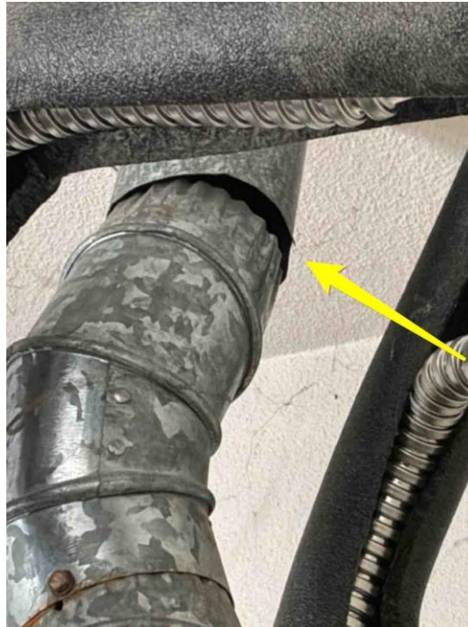
Connector pipe found disconnected
