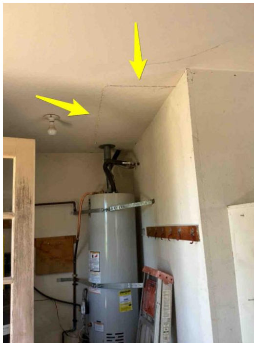
Example. In the garage over the water heater
