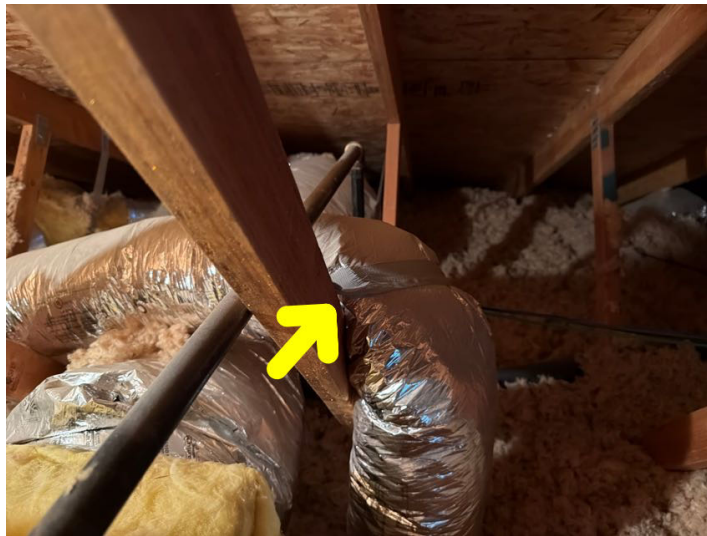
One or more of the flexible ducts are crushed and should be serviced by a licensed HVAC contractor.
