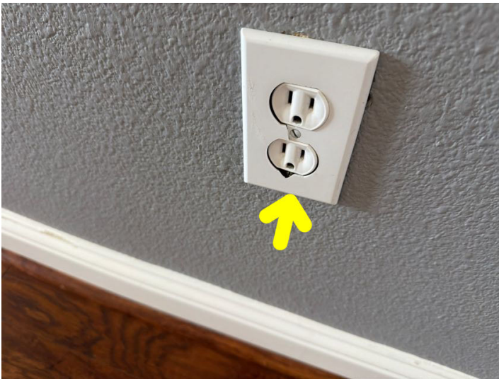
One or more outlet covers are cracked or broken and should be serviced.
