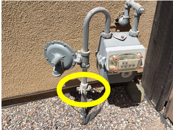
The gas main shut-off is located on the right side of the home, unit or building.
