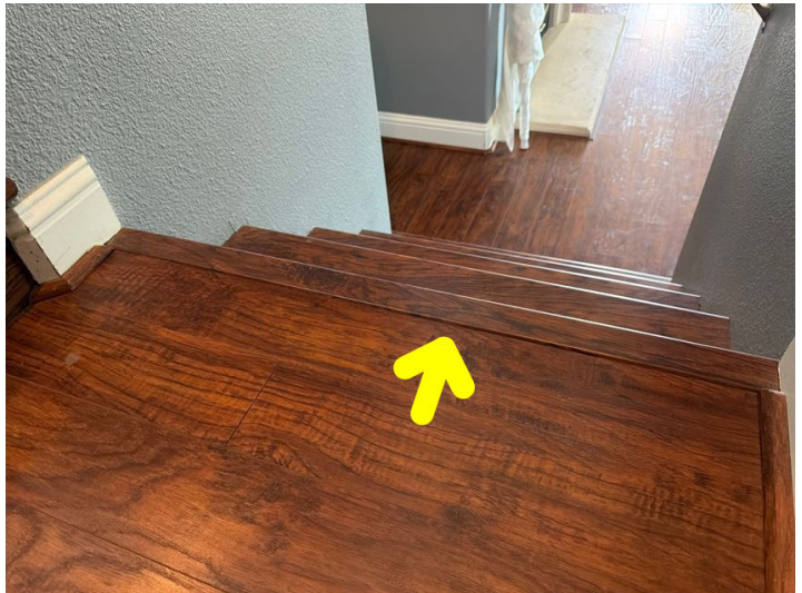
There is an offset in the floor that could prove to be a trip hazard.
