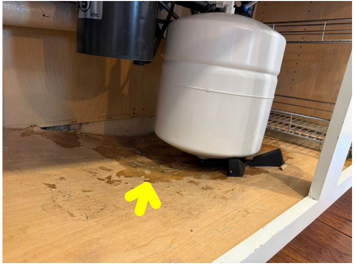
The floor of the kitchen sink cabinet is damaged, and should be replaced.
