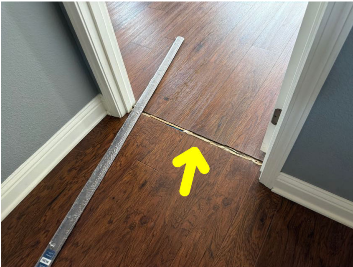
The entry door floor trim is missing or damaged and should be replaced.
