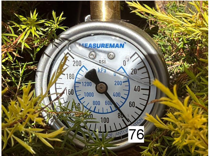
The pressure inside the residence is nearing 80 PSI and will stress components of the system. A qualified tradesperson should reduce the pressure at the regulator to sixty pounds per square inch. However, the regulator may have failed and would need to be replaced.
