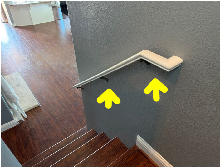
A handrail is loose and should be secured for optimal safety.
