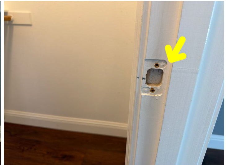
The closet door striker plate is missing and should be adjusted for the striker pin to engage.
