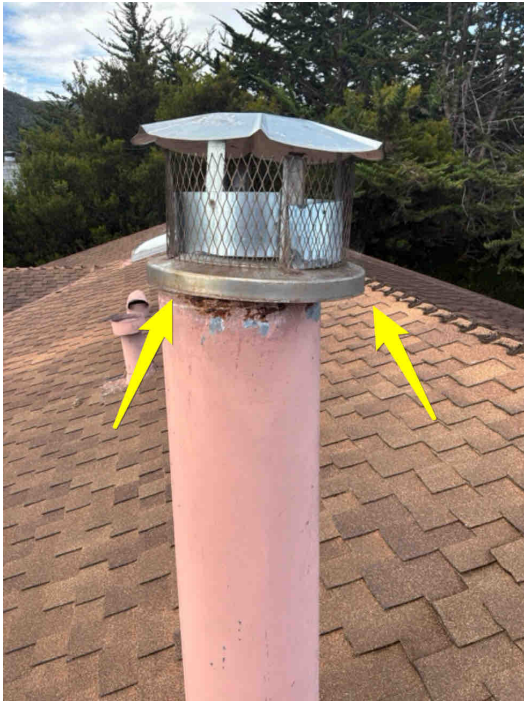
The chimney pipe appears to be loose and or disconnected
