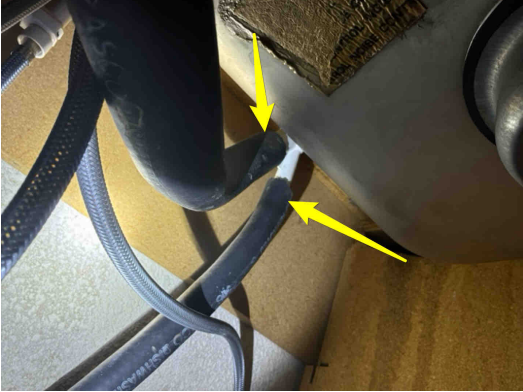
The air gap under the kitchen sink
