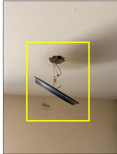
An interior light fixture in the garage was damaged at the time of the inspection.
