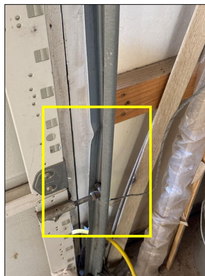
The track was damaged and needed repair.
