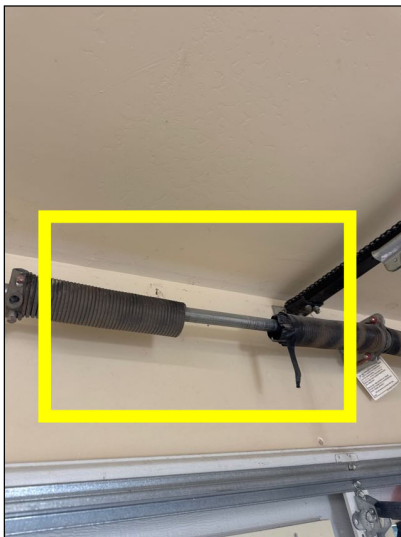
Springs supporting an overhead garage door were broken and needed replacement.
