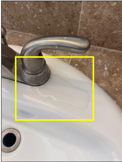
The faucet at this bathroom sink leaked when the water was turned on. (right side)
