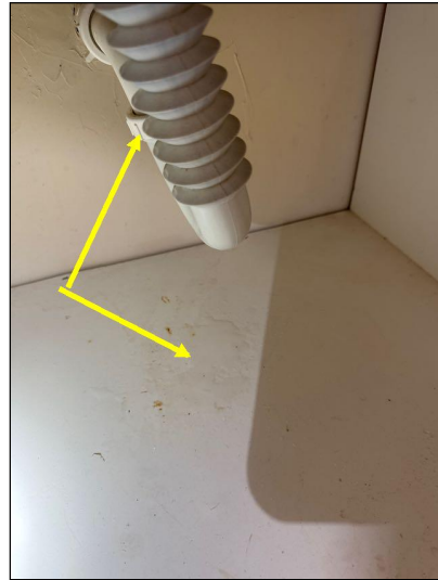
Leaking connections at the trap assembly beneath the bathroom sink (right side)
