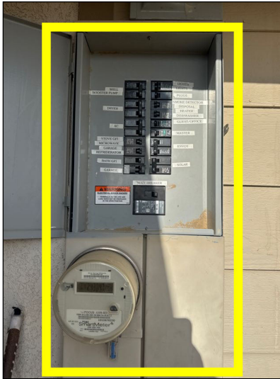
Main electrical service panel to the home.
