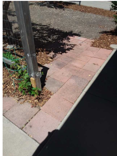
The paver patio or walkway has multiple offsets. This may be due to unsuitable soil below the pavers.
