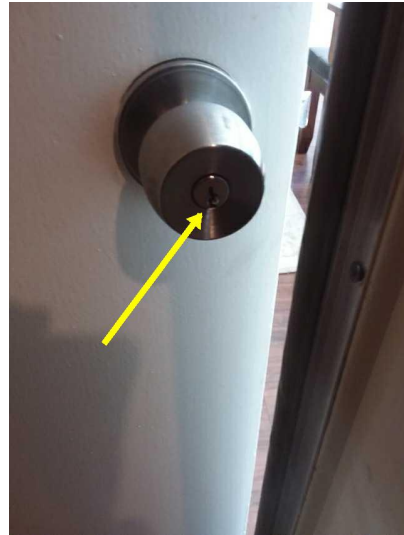
The keyed deadbolt could prevent or impede an emergency exit, and should be replaced with a safer latch type.
