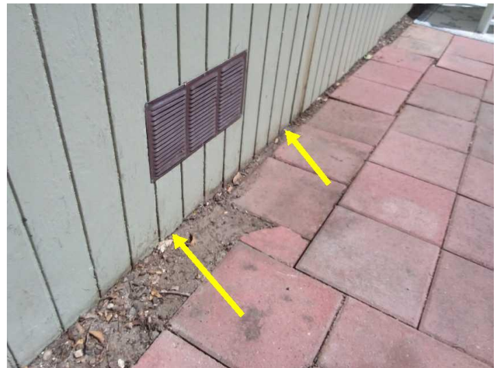
There are areas where the wooden siding is close to or touching the ground and is subject to moisture damage. These areas should be monitored closely and sealed frequently to prevent moisture damage. Wooden siding should be a minimum of 4 inches from soil and 2 inches from hard surfaces.
