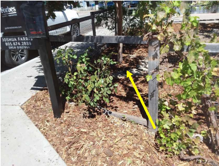
The fences have damage that you may wish to have repaired.
