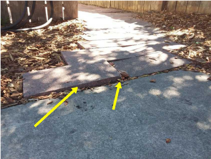
There is one or more offsets in the walkways that could prove to be trip-hazards.
