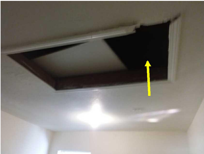
The hatch cover to the attic area should be sheathed with metal or drywall, and made to self-close and latch, in order to provide a firewall separation between the garage and the residence.
