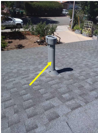
A rain collar is missing on a heat vent and should be installed.
