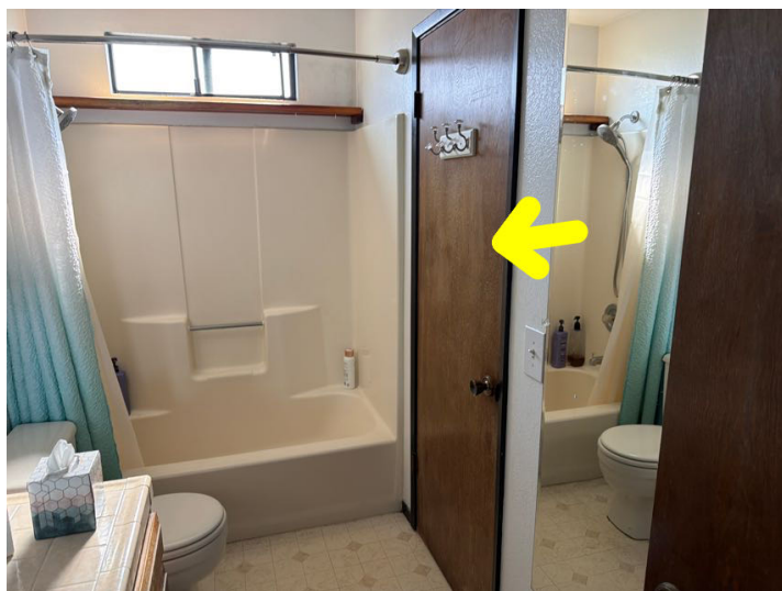
A door is blocked or locked and could not be tested, and should be demonstrated as functional.
