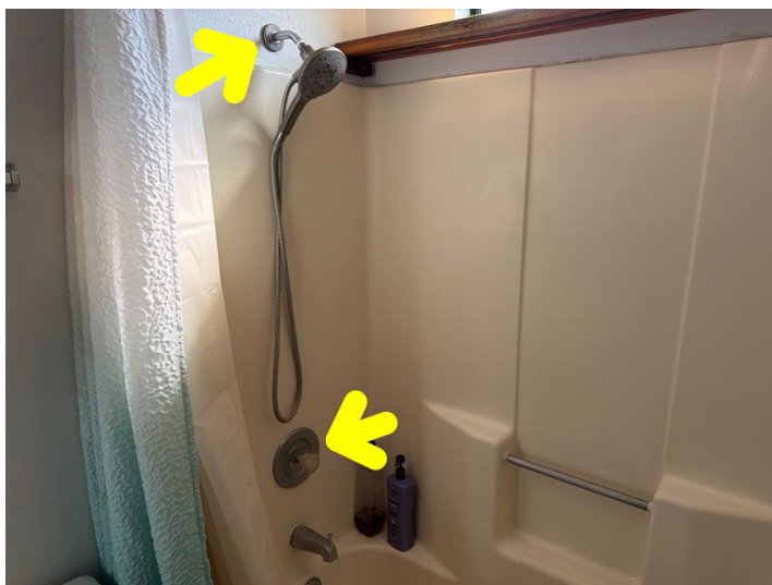
The tub/shower water supply pipe is loose and should be serviced.
