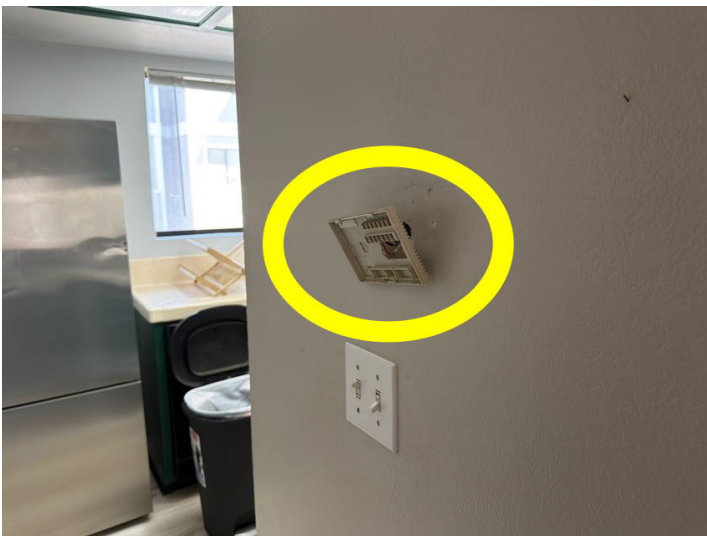
The thermostat is missing and should be replaced.
