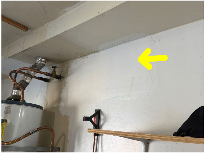
There had been a drywall/plaster repair that should be explained by the seller.
