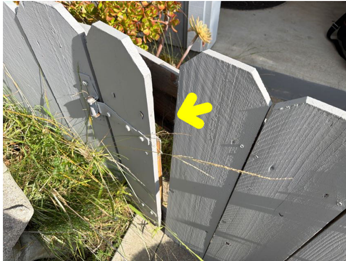
The gate at the front needs to be serviced to be functional.
