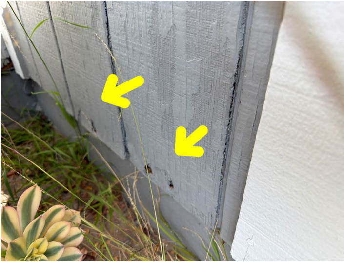
Portions of the siding have dry rot or are moisture damaged, and should be evaluated by a pest inspector.
