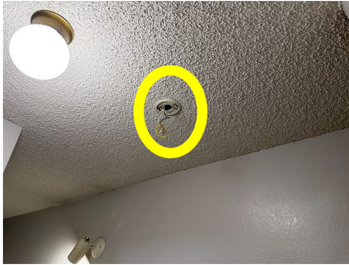
A pre-wired smoke detector is missing and should be replaced.
