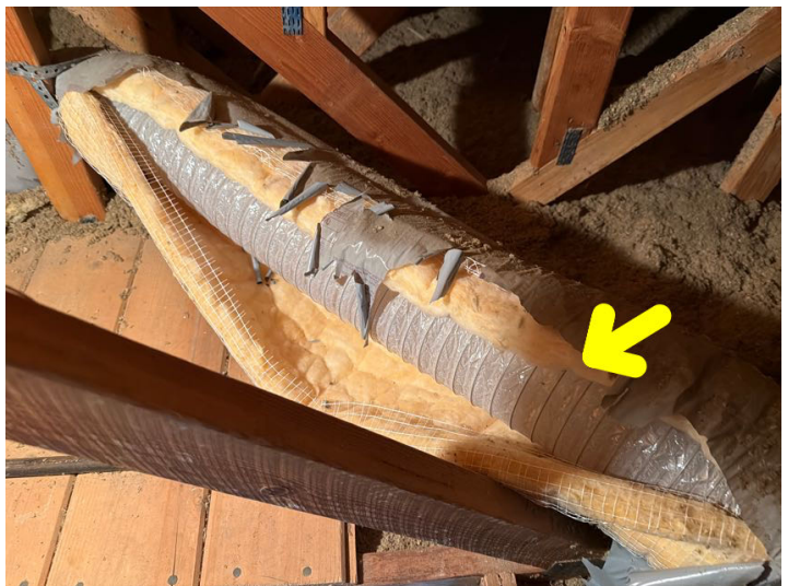
Sections of outer shell of the flexible ducting have been damaged by ultra-violet contamination, which has caused the outer shell to deteriorate, and therefore should be evaluated by a licensed HVAC contractor with a view toward replacement.
