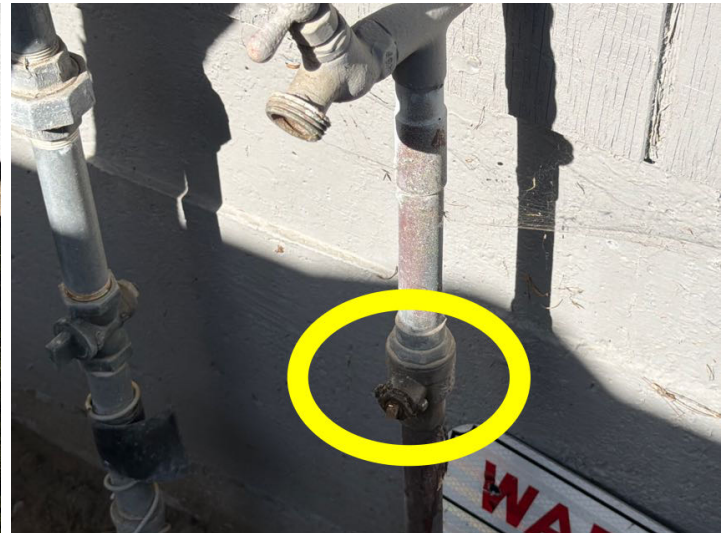
The main water shut off valve handle is missing and it should be replaced.
