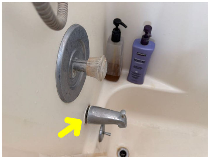
The tub spout should be sealed to the wall.
