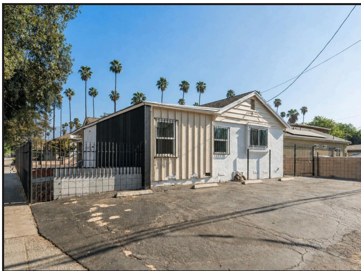
SIDE YARD — SEPARATE GAS AND ELECTRIC METERS
