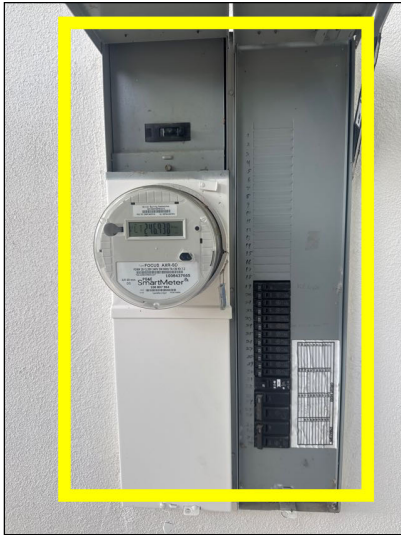
Main electrical service panel to the home.
