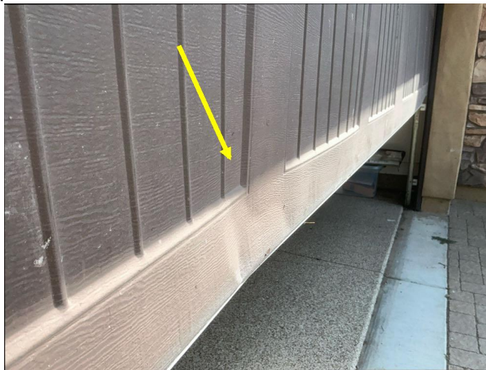
The garage door has damage that you should view for yourself.
