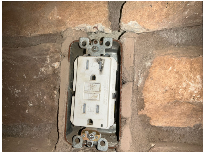
An outlet at the rear is damaged or has a scorch mark on it and should be evaluated and serviced by a licensed electrical contractor.
