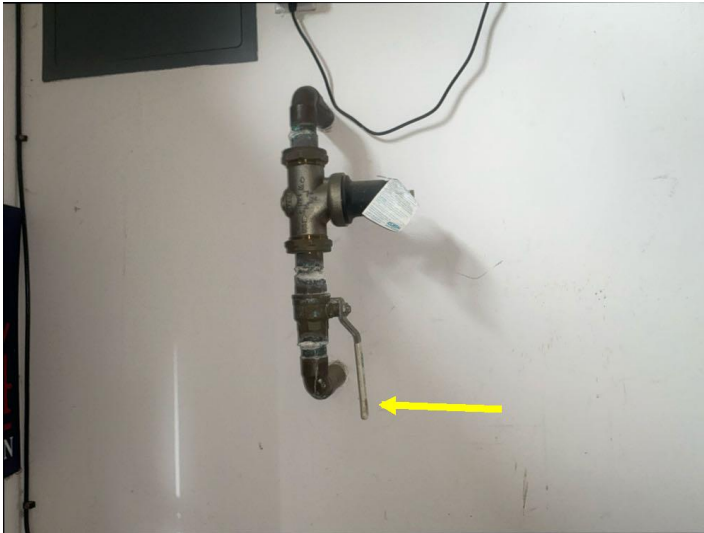
Main water shutoff
