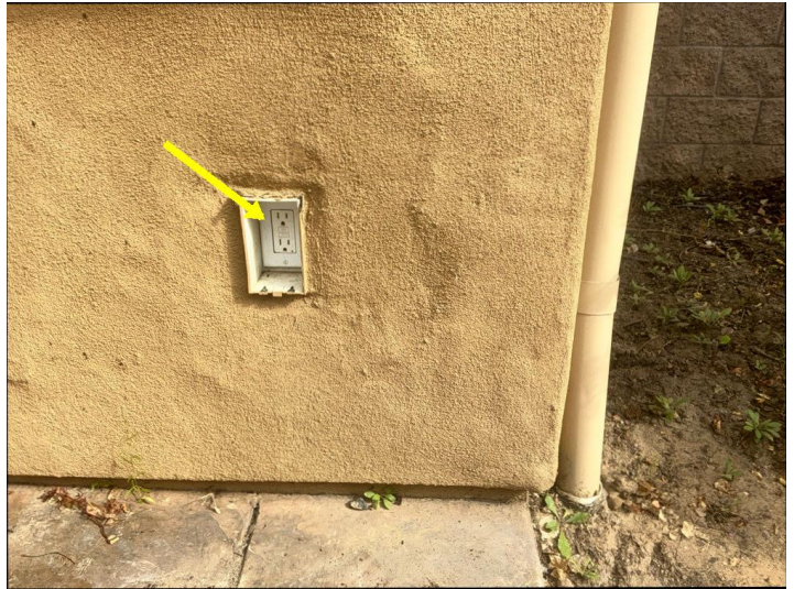
A ground-fault protected outlet on the front does not reset and should be serviced.
