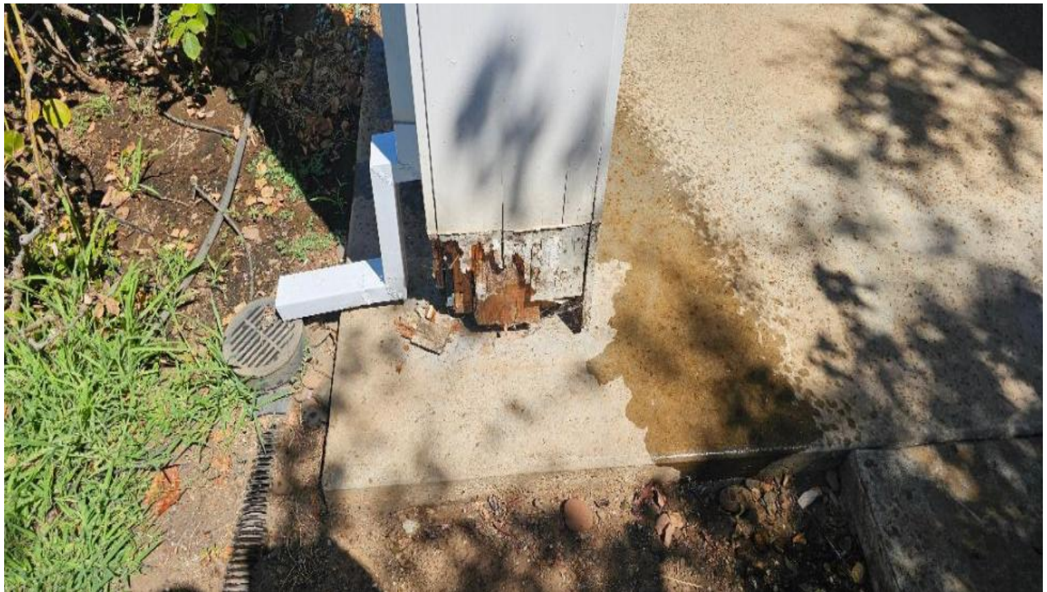
3A - Damaged wood trim with possible hidden damage to the support post.
