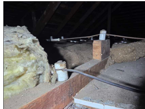
Wiring method: knob and tube present in areas of the structure - considered obsolete - recommend complete inspection by electrical contractor @ attic
