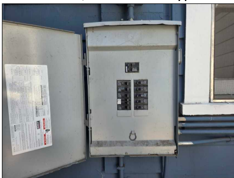
General view - main panel
