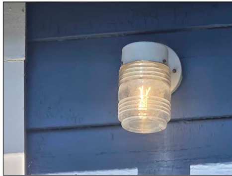
Exterior light(s) tested and operated
