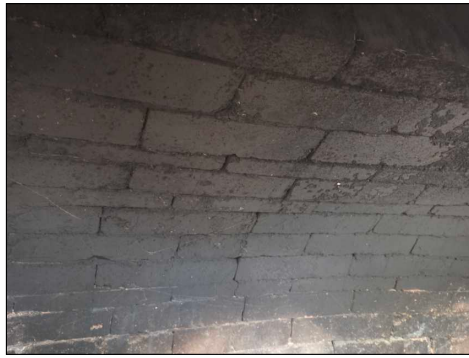
Small cracks/worn areas present at firebox - typical for age
