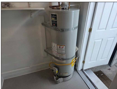
Water heater tested and operated
