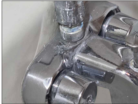
Leak at shower line connection - needs to be serviced @ 207
