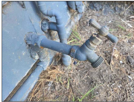
Bibb(s) not functional at one or more locations - needs to be serviced ( galvanized )
