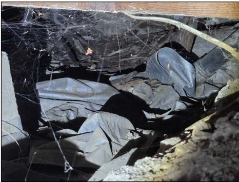
Debris/soil obstructing access in areas - confined areas in crawl space - very limited access
