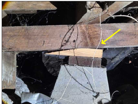
Irregularly shimmed posts - needs to be serviced
