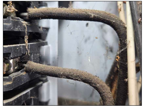
Wiring method: Cloth wiring observed at various locations throughout the property - we recommend a licensed electrician for upgrade of all older materials
