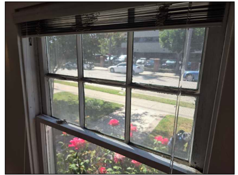
Missing sash/cables - needs to be serviced
