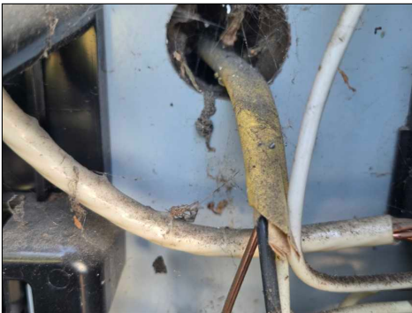
Wiring method: non-metallic sheathed cable (romex)
