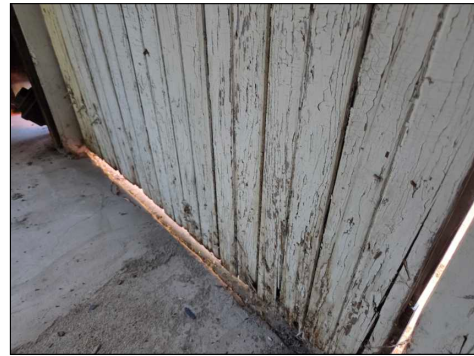
Deteriorated wood present - needs to be serviced
