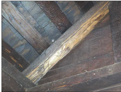
Deteriorated wood members - needs to be serviced
