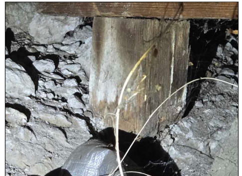
Wood post are worn/older - recommend upgrade
