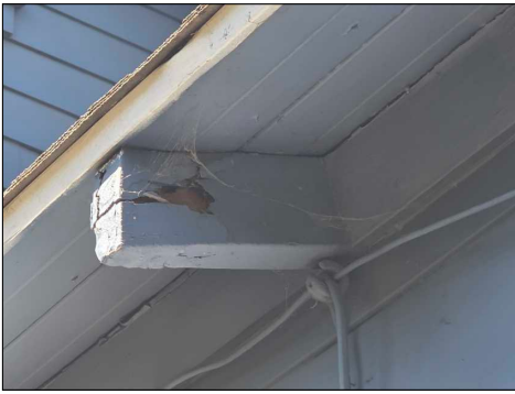
Deteriorated wood - recommend evaluation by termite inspector
