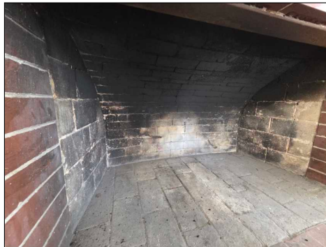
No gas present/visible
