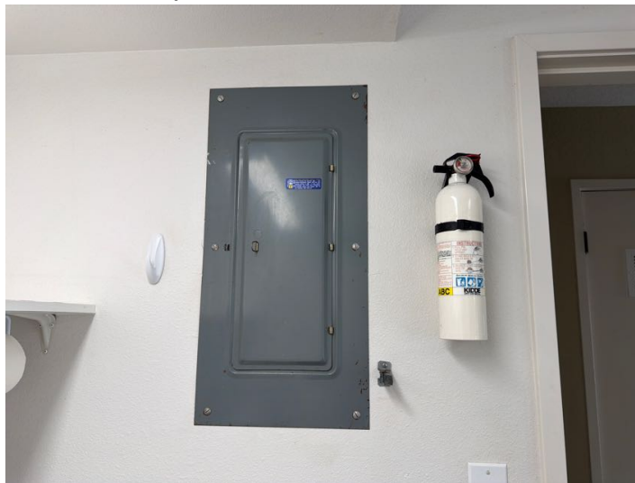
The sub panel is located in the garage.
