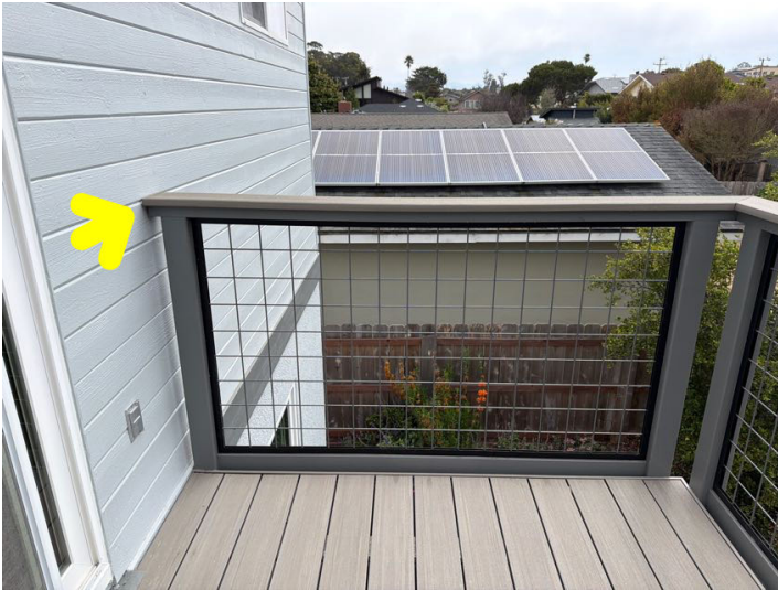
Sections of the guardrail are not secure, and should be serviced.
