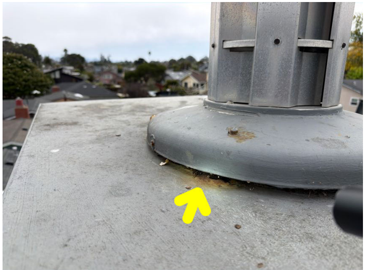
The sheet metal chase cover, which is designed to seal the chimney wall and shed rainwater, is damaged, deteriorated, or rusted and should be serviced by a certified fireplace specialist.
