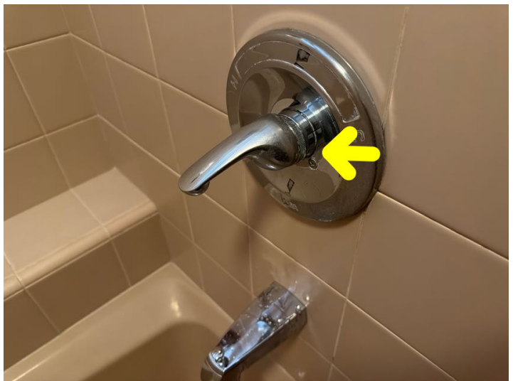
The shower faucet leaks around the stem while in use, and should be repaired by a qualified tradesperson.
