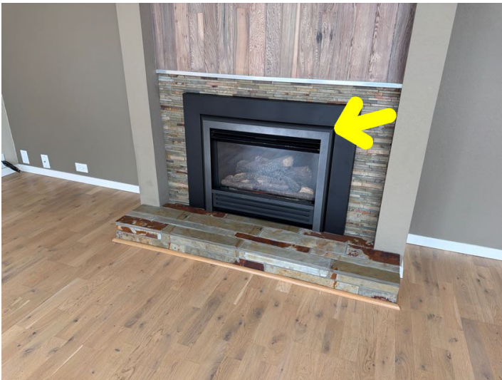
The ornamental gas log fire is functional.
