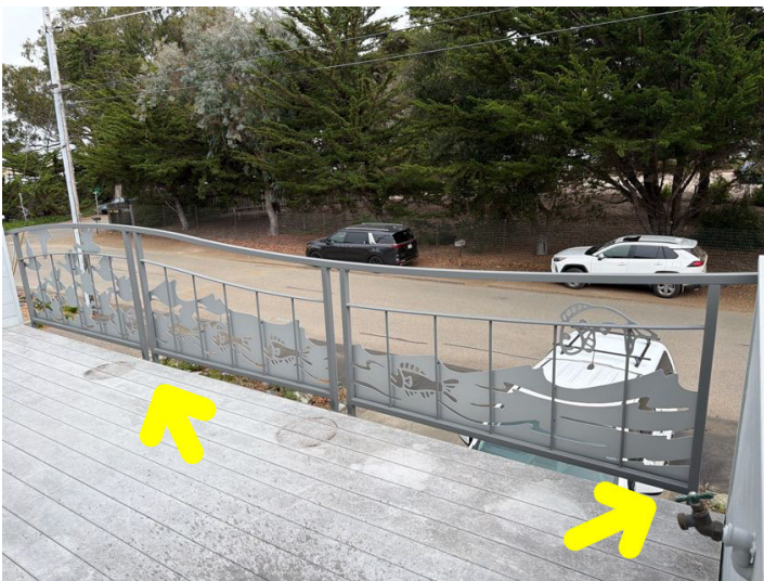
Sections of the guardrail are not secure, and should be serviced.
