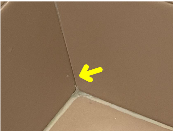
One or more open seams in the tub/shower area need to be caulked or re-grouted to forestall moisture intrusion.
