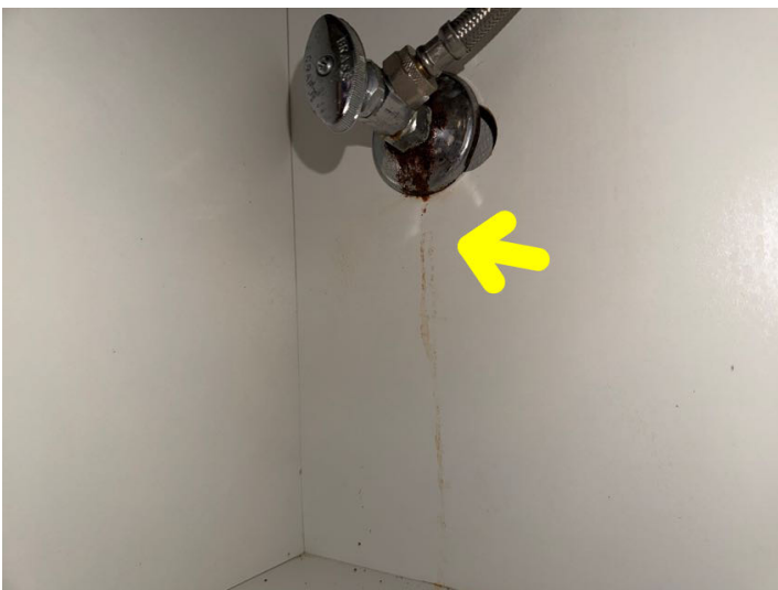
The wall of the sink cabinet below a water valve is functional but moisture damaged, which could indicate a leak, and should be evaluated by a qualified tradesperson.
