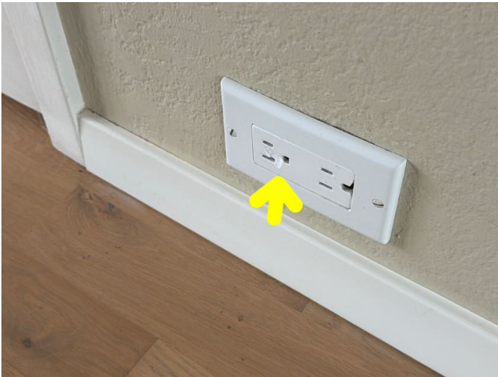
One or more outlets are damaged, and should be evaluated and serviced by a licensed electrical contractor.
