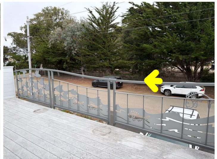
The balcony guardrail does not conform to common safety standards. Common safety standards require them to be a minimum of 42 inches high when the standing surface is thirty inches or more above grade. Also, guardrail pickets should be no more than four inches apart for child safety.
