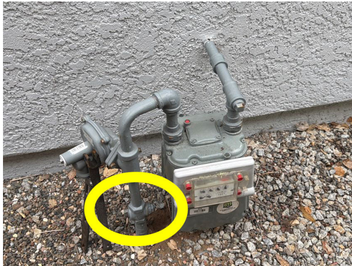
The gas main shut-off is located on the left side of the home, unit or building.
