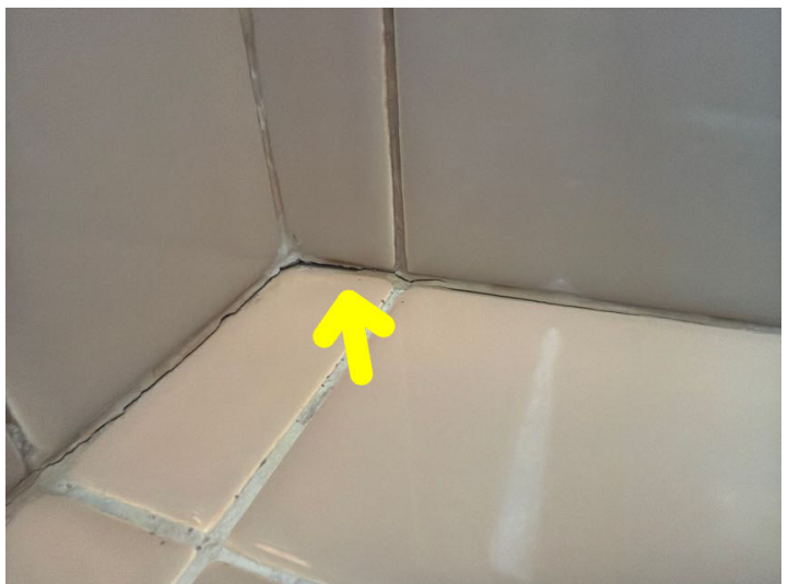
There is a separation between the sink countertop and the back-splash, which should be sealed to forestall moisture intrusion between the cabinet and the wall.
