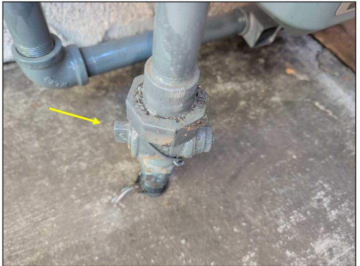
Gas supply shut off.
