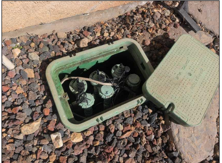
Rear irrigation control valves.
