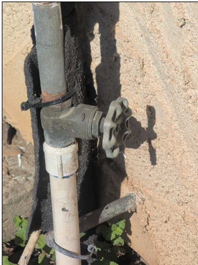
Irrigation isolation valve.
