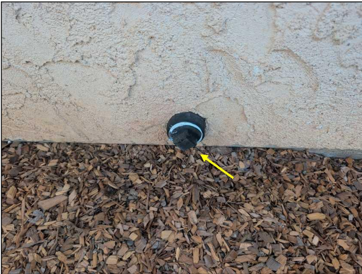
Plumbing drain clean out.
