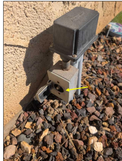
Switch for pool light.
