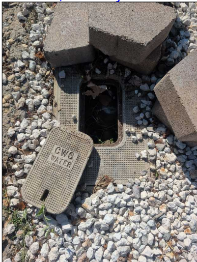
Water meter/utility shut off.
