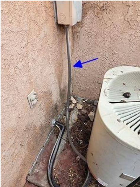
Photo 36-1 At the A/C unit
