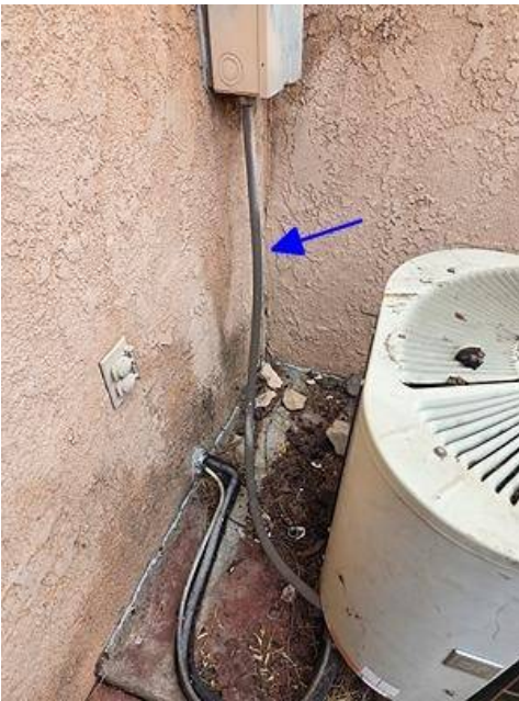
Photo 36-1 At the A/C unit
