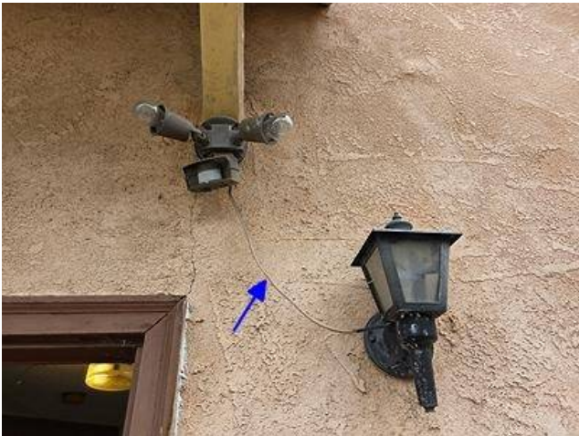
Photo 35-1 Front of unit
