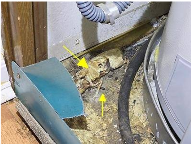
Photo 1-3 Water heater closet
