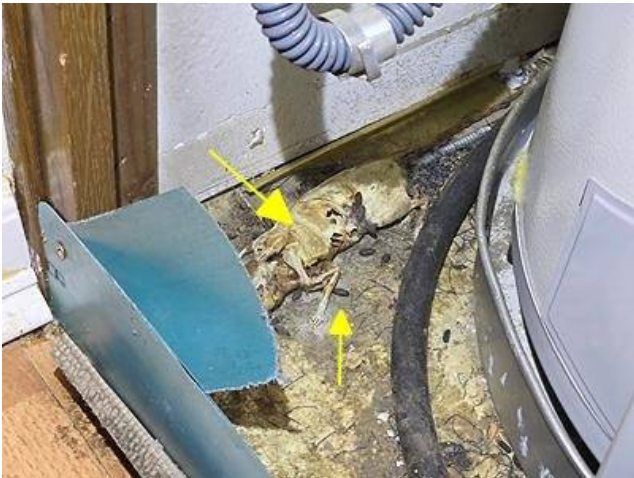
Photo 1-3 Water heater closet
