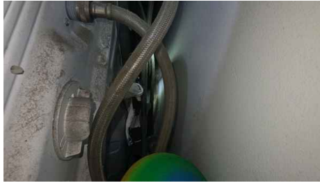
Dryer Hook Up: Fuel Gas
