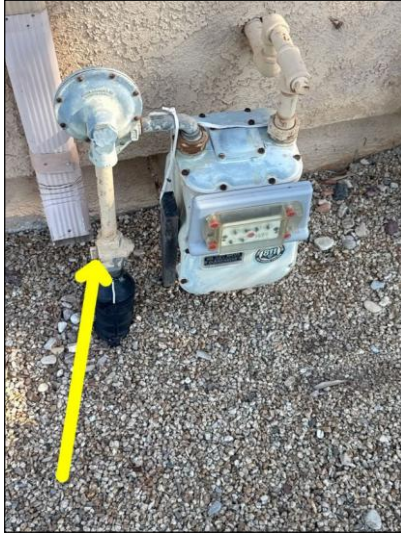
Main gas shut off to the home.
