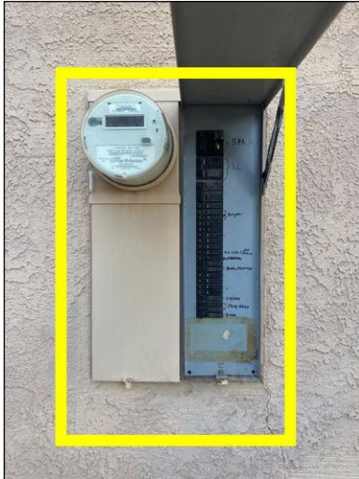
Main electrical service panel to the home.
