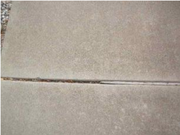
Damaged wood spacer in the driveway.
