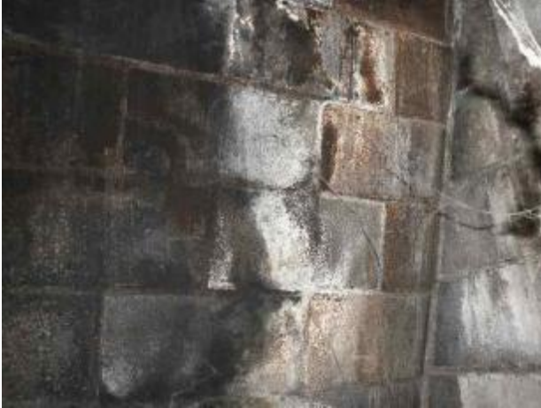
Evidence of water intrusion inside the fireplace.
