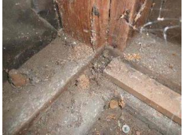
Evidence of termite infestation in the garage.
