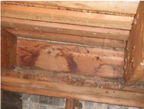
Water stain below the chimney flashing.
