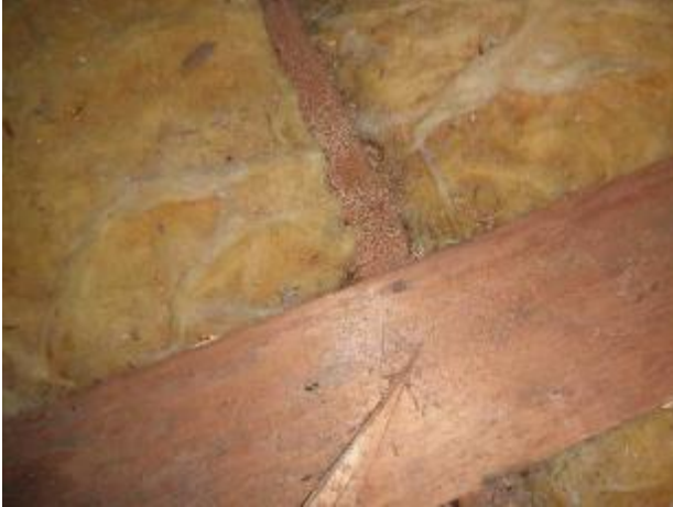
Evidence of termites in the attic space.
