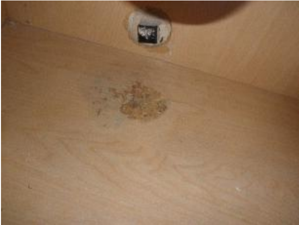
Moisture damage to the base of the master bathroom sink cabinet.
