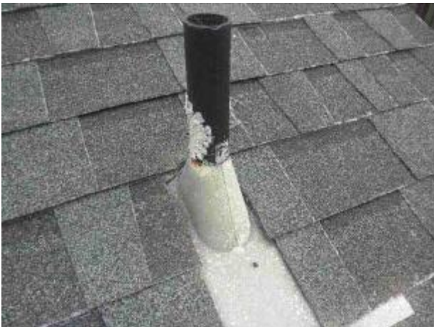
Reseal all of the flashings.
