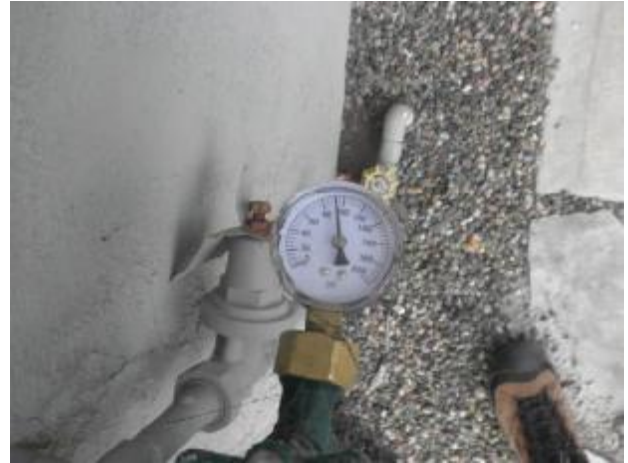
Water pressure was greater than the maximum allowable of 80 psi.
