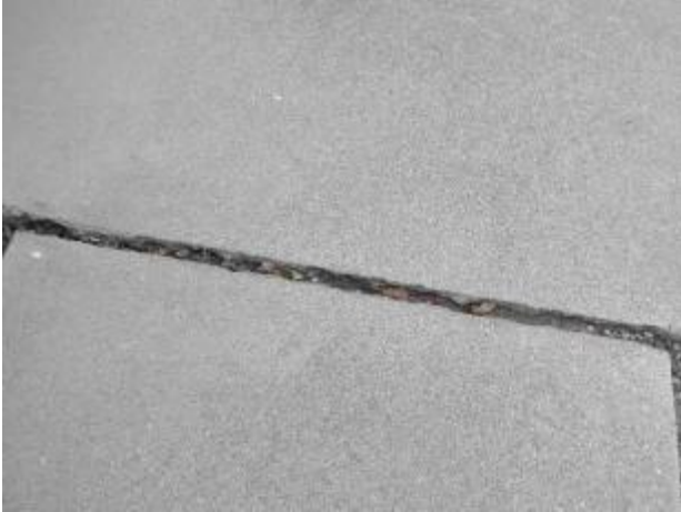
Uplifting at the concrete walkway.
