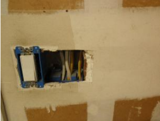
Opening in the firewall between the garage and the home.
