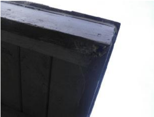
Moisture damage to the SW fascia.
