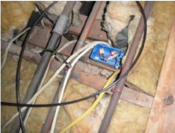
Example of missing cover plates at junction boxes in the attic.
