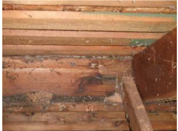
Water stain below the chimney flashing.
