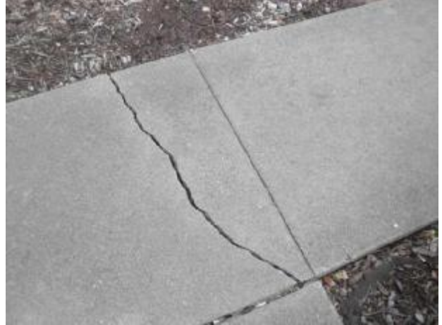
Example of general cracks in the concrete walkways.
