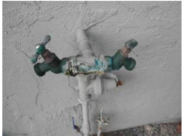
Leak at the hose bib on the SW wall.
