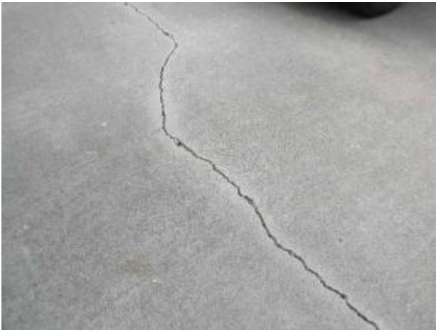
General cracks in the concrete driveway.
