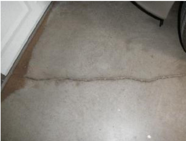
Settlement crack in the garage slab.
