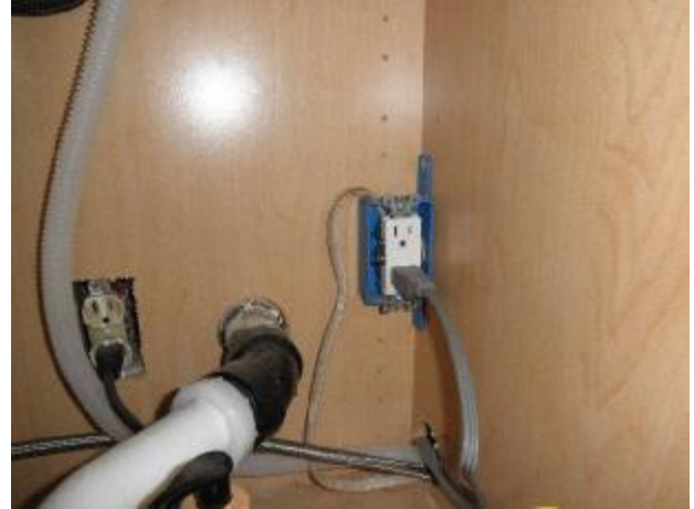
Exposed Romex wiring and missing cover plates below the kitchen sink.
