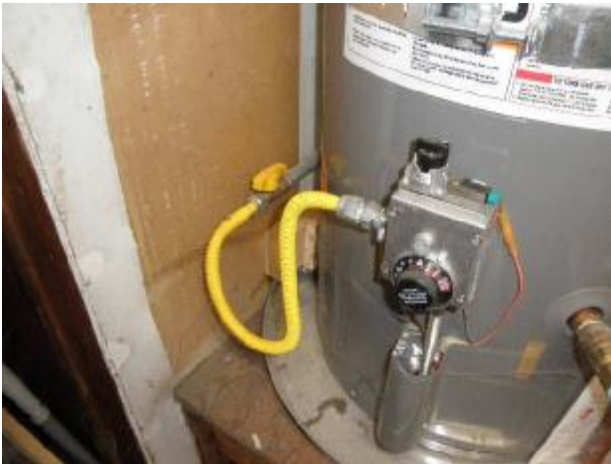
Missing sediment trap at the water heater gas line.
