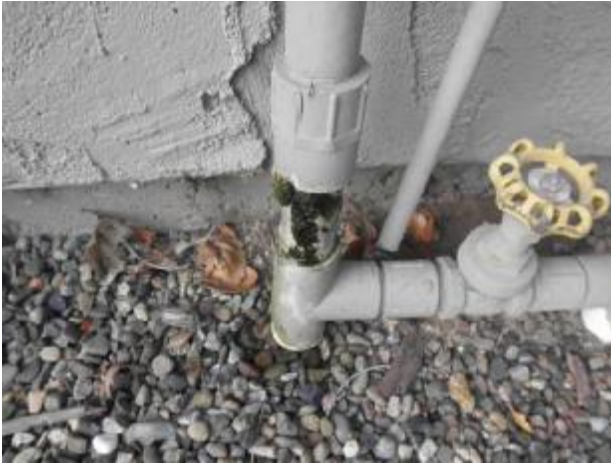
Leak at the main water riser.
