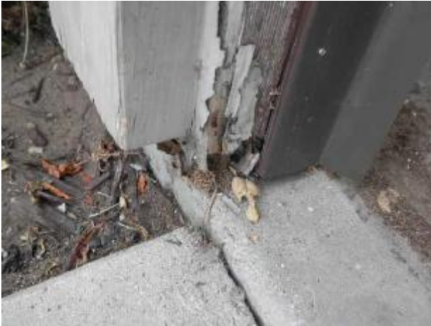
Termite damage to the garage vehicle door jamb.
