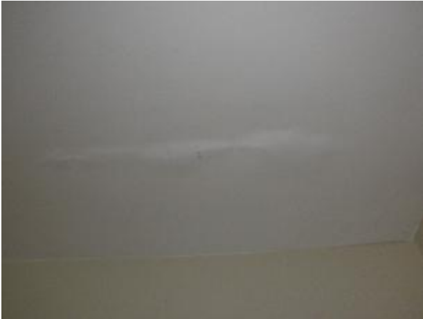
Water stain and bubbling paint above the front entry door.
