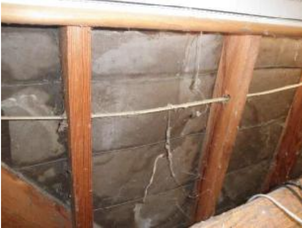
Horizontal Romex wiring less than seven feet off the ground in the garage.
