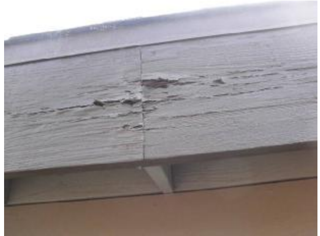
Moisture damage to the south fascia.
