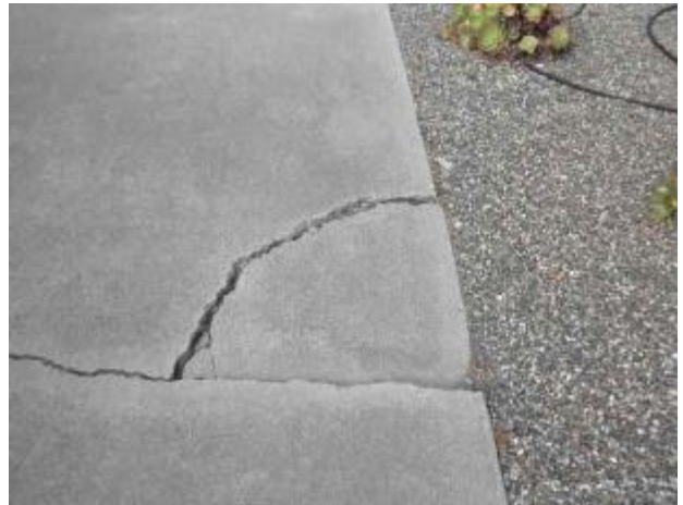
General cracks in the concrete driveway.
