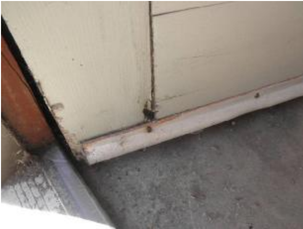
Moisture damage to the base of the garage side door.
