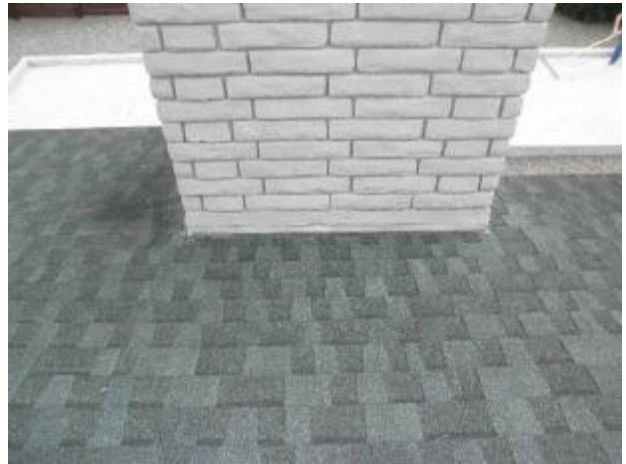
Missing cricket flashing behind the chimney.
