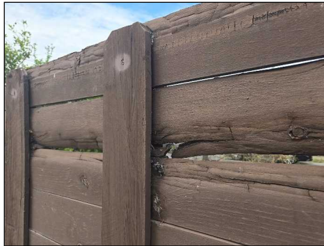
Damaged fencing/walls - needs to be serviced
