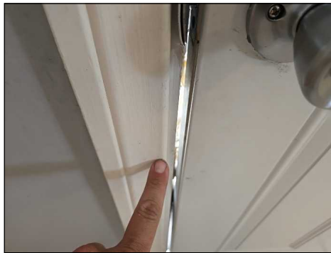
Gap at sides - needs to be serviced
