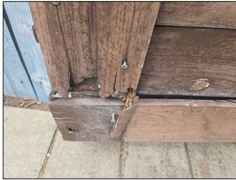
Damaged - needs to be serviced
