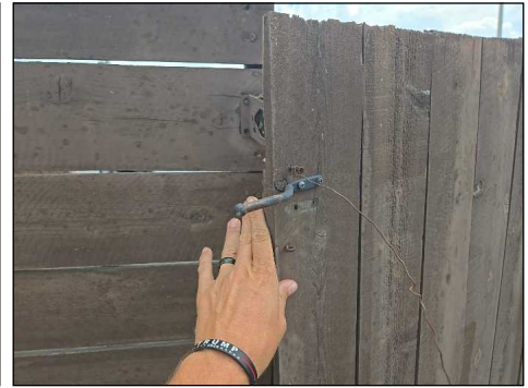
Damaged - needs to be serviced
