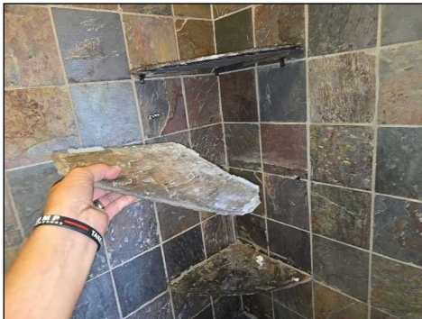
Soap dish loose/damaged - needs to be serviced - possible hidden defects
