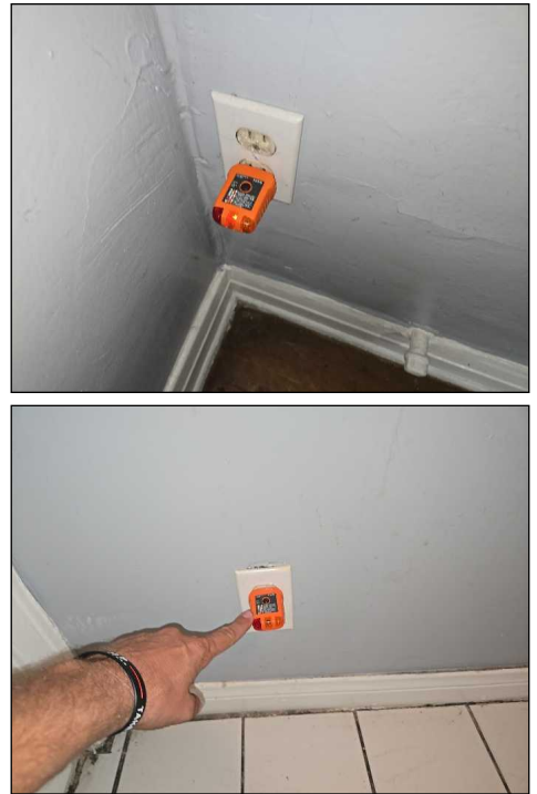
Non-energized (dead) outlet(s) - needs to be serviced
