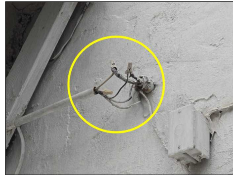
Older style wiring connections to the structure - it is recommended that you upgrade these areas
