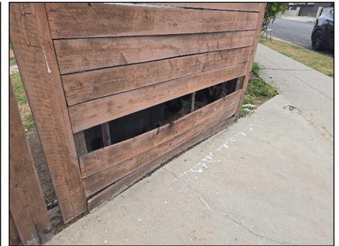
Damaged fencing/walls - needs to be serviced
