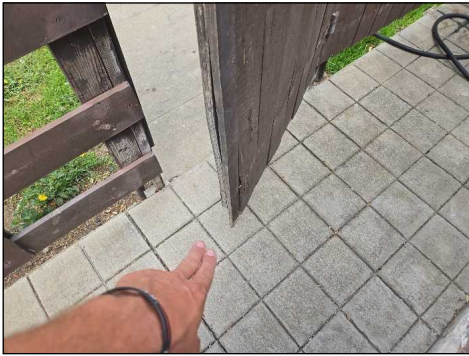
Gate is sagging - recommend servicing
