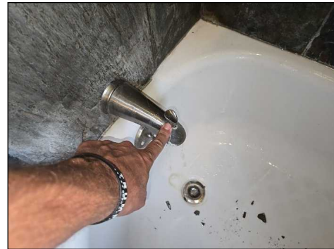
Tub fixture is seized/stuck in position - needs to be serviced
