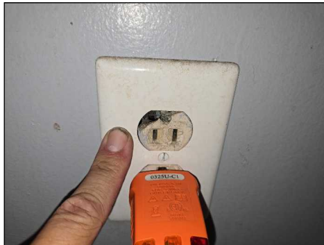
Broken outlet(s) - potential hazard - needs to be serviced
