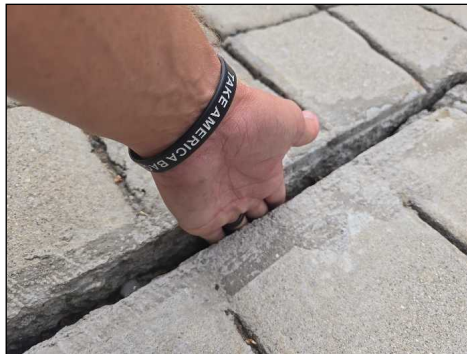
Cracking/chipping large - recommend servicing
