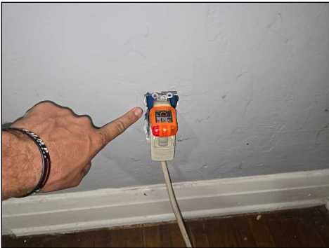
Outlet cover missing - needs to be serviced
