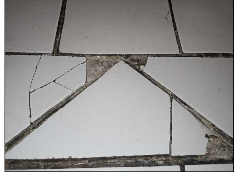
Damaged- needs to be serviced
