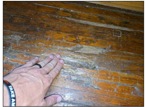
Damaged flooring – service needed
