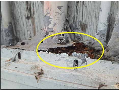
Gaps on top of panel- needs to be serviced
