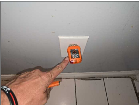
Non-energized (dead) outlet(s) - needs to be serviced
