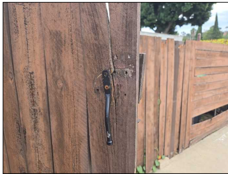
Damaged - needs to be serviced
