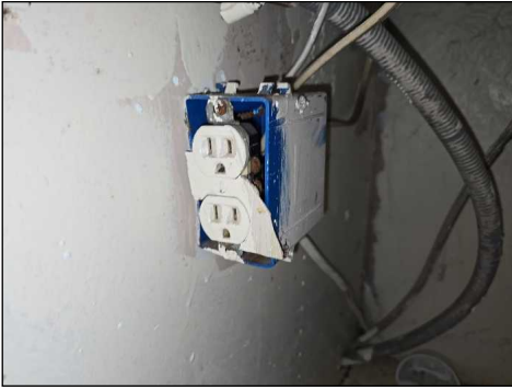
Outlet cover missing - needs to be serviced
