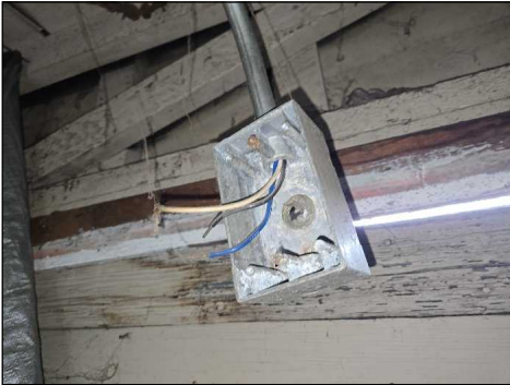
Irregular installation/workmanship- not to accepted building practices - needs to be serviced
