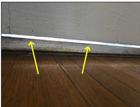
Gap at bottom - larger than normal for air flow, needs to be serviced
