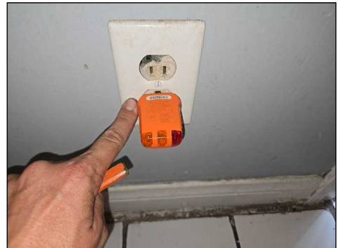
Non-energized (dead) outlet(s) - needs to be serviced
