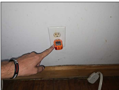
Non-energized (dead) outlet(s) - needs to be serviced
