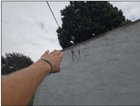
Cable clearance to the garage is low (12 feet high is recommended) - needs to be serviced
