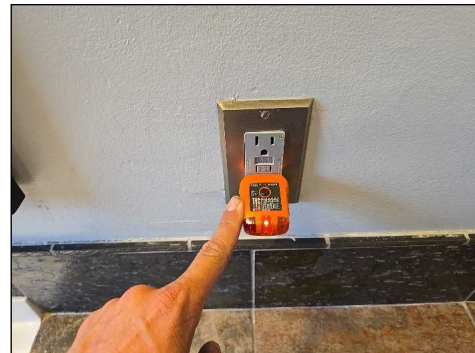
GFCI not grounded- needs to be serviced
