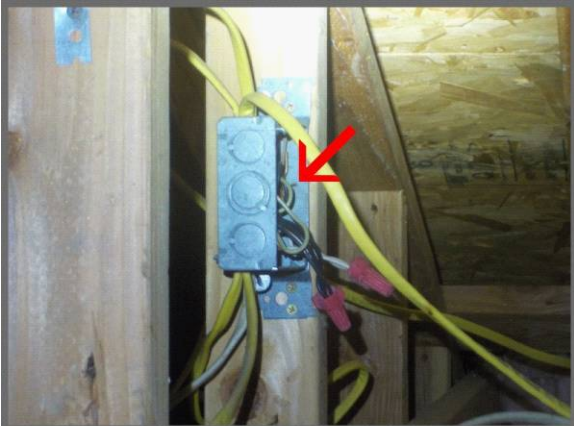
opened junction box
