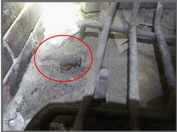
gas line is not capped
