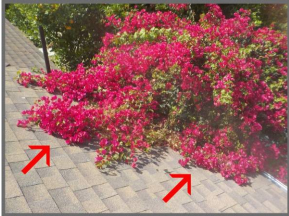
branches on the roof
