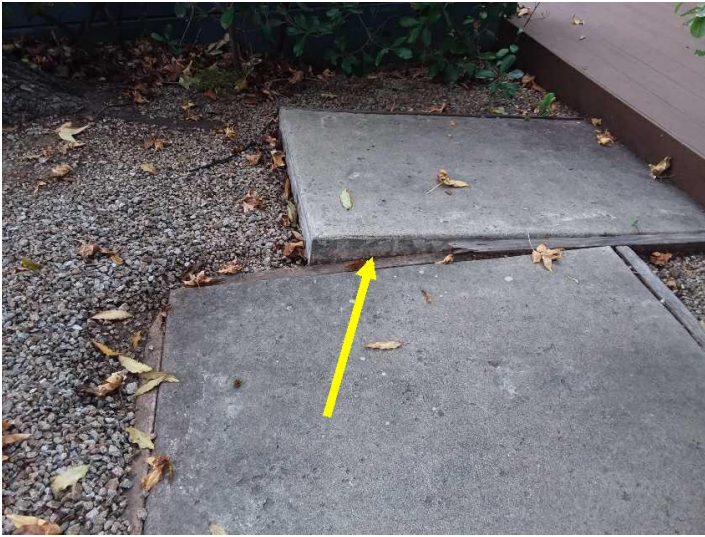
A walkway has been displaced by root movement and could present a trip-hazard.
