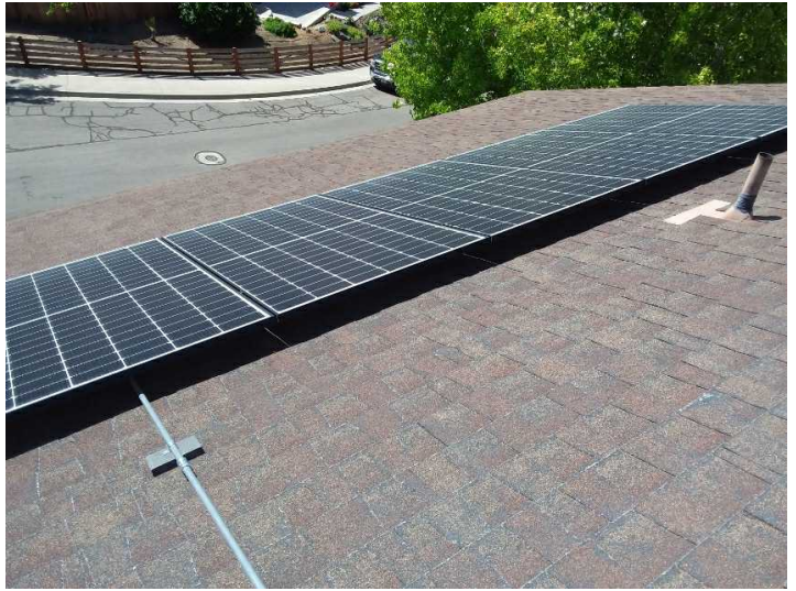
5 panels on front roof
