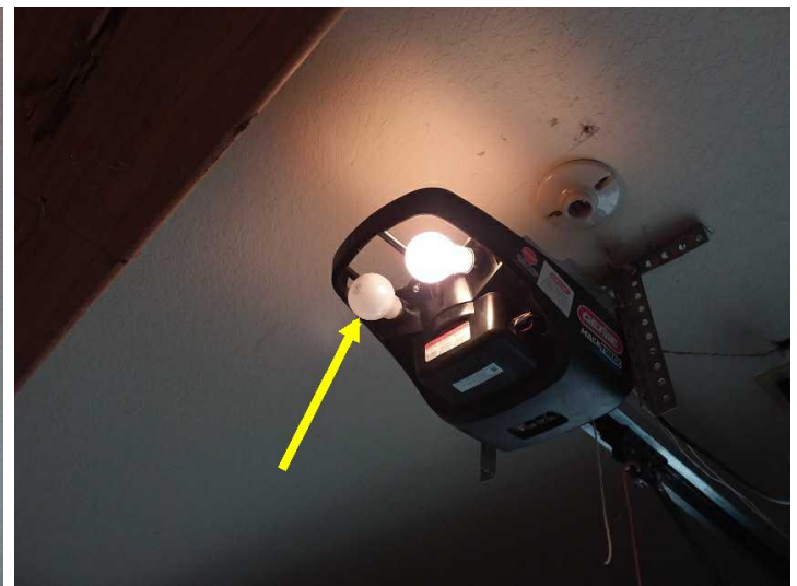
The garage door opener light bulb did not respond when the auto-reverse mechanism was activated, which should be serviced. This is important because it typically is the only light on when pulling into the garage at night.
