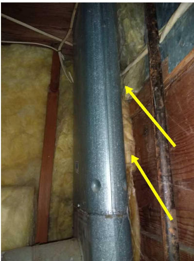
Insulation is in contact with the vent pipe and should be removed to a minimum of three inches away.
