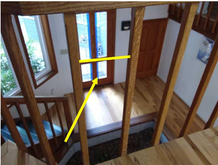
The balusters in the stair or guardrails are more than four-inches apart and are not child safe. Therefore, you may wish to add a protective barrier.
