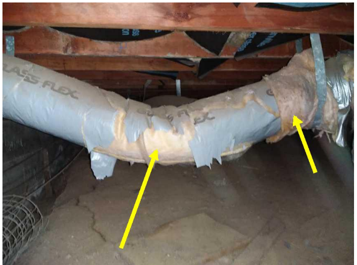
Sections of outer shell of the flexible ducting has been damaged by ultra-violet contamination, which has caused the outer shell to deteriorate and, therefore should be evaluated by a licensed HVAC contractor with a view toward replacement.
