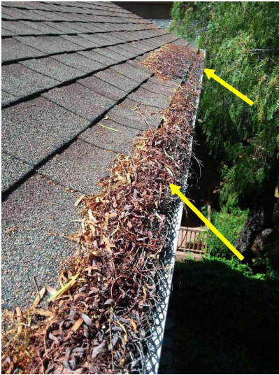
Some of the gutters need to be cleaned to drain properly.
