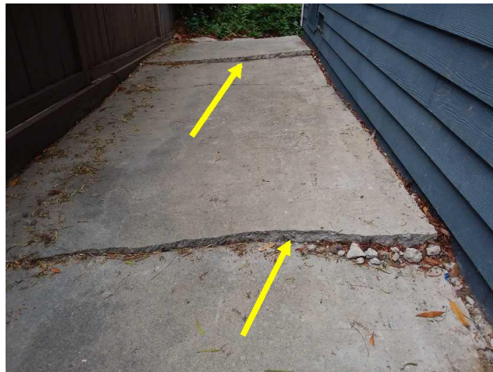
The walkways are variously damaged and should be repaired or replaced.
