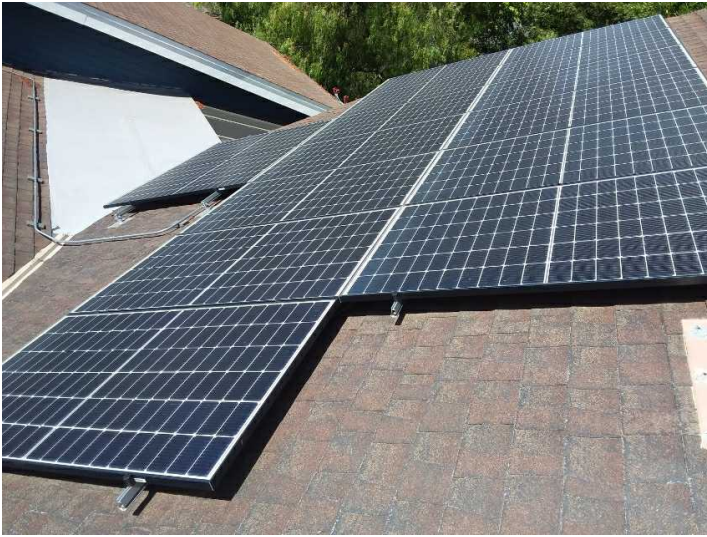
15 panels on middle roof
