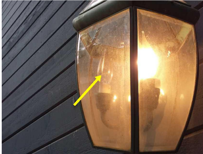
A wall light did not respond and should be serviced.
