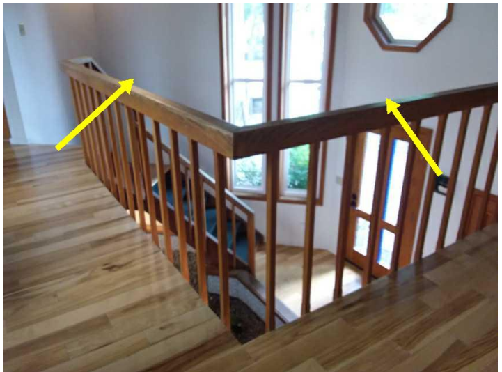
The Guardrail at the top of the stairs is not the recommended 42 inches high when the standing surface is more than 30 inches below.
