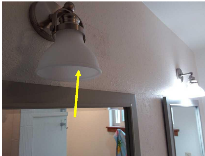
The wall light does not respond and should be serviced.
