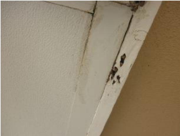
Evidence of possible termite infestation/damage to the fascia board on the west side of the garage,
