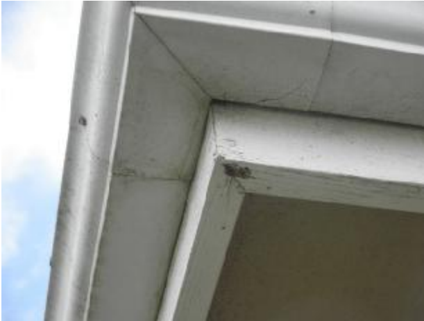
Example of the moisture damage to the fascia boards at the outside corners of the roof.
