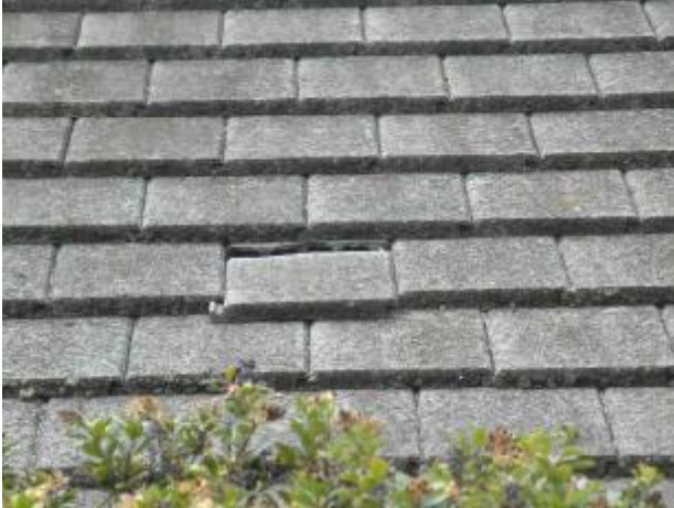
Cracked and displaced roof tile on the north facing slope.
