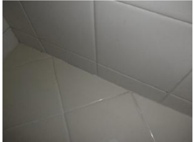
Minor grout work needed at the hall bathroom shower.
