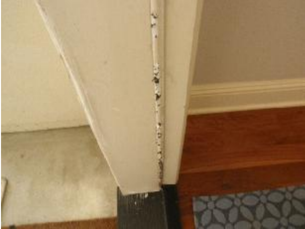
Damaged weather stripping at the garage fire door.
