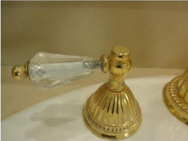
Damaged faucet handle in the master bathroom.
