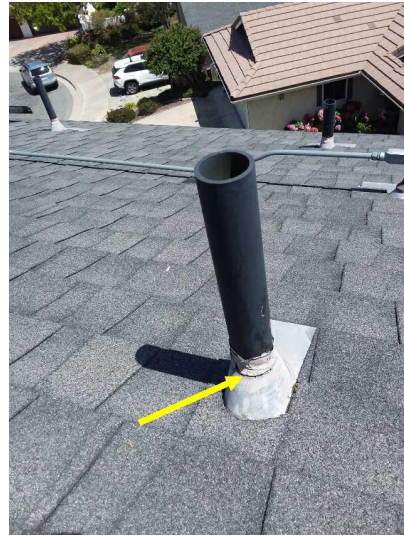
Some of the roof flashing need to be sealed or serviced. They are comprised of metal that seals valleys and vents and other roof penetrations, and are the most common point of leaks. This is particularly true of the flashing on a layered roof, which are covered by the roofing material and which are even more susceptible to leaks.
