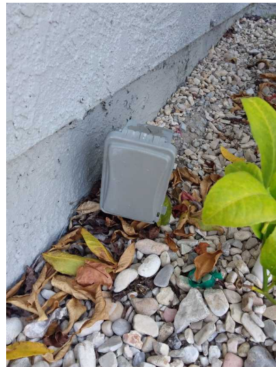
The exterior outlets are functional, but should be upgraded to have ground fault protection.
