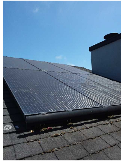
6 panels on lower front roof
