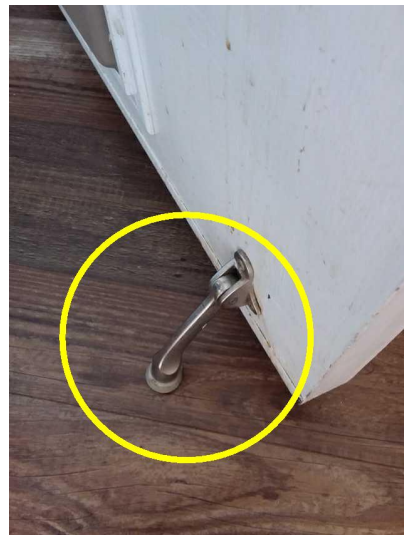
The fire rating of the house entry door has been nullified by the addition of a foot operated door stop.
