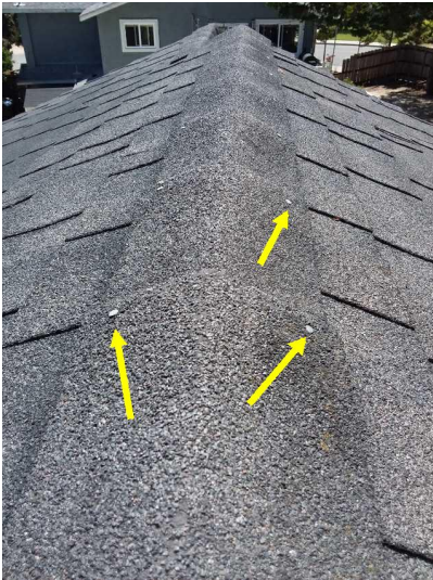
The roofing material has been improperly installed with exposed fasteners and should be monitored closely for leaks.
