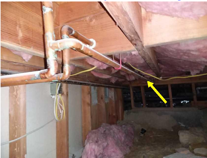
Some of the water supply lines are insufficiently supported and should be serviced.
