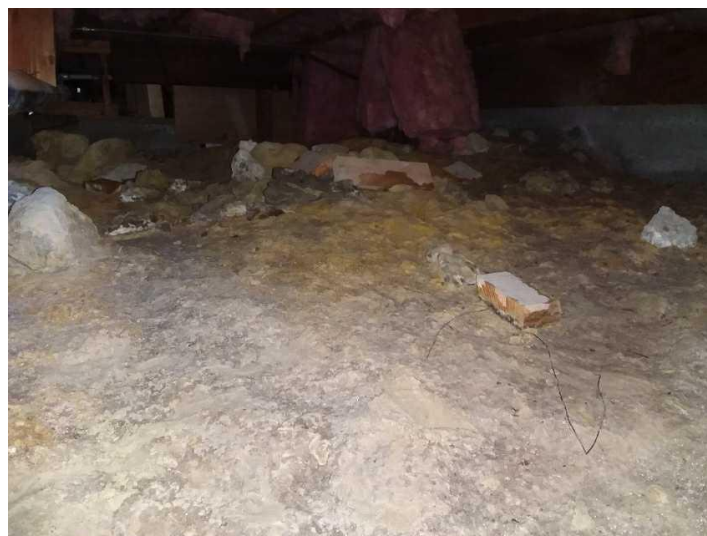
The soils in the crawlspace are moist or desiccated, which could indicate a chronic drainage problem that should be evaluated by a specialist.
