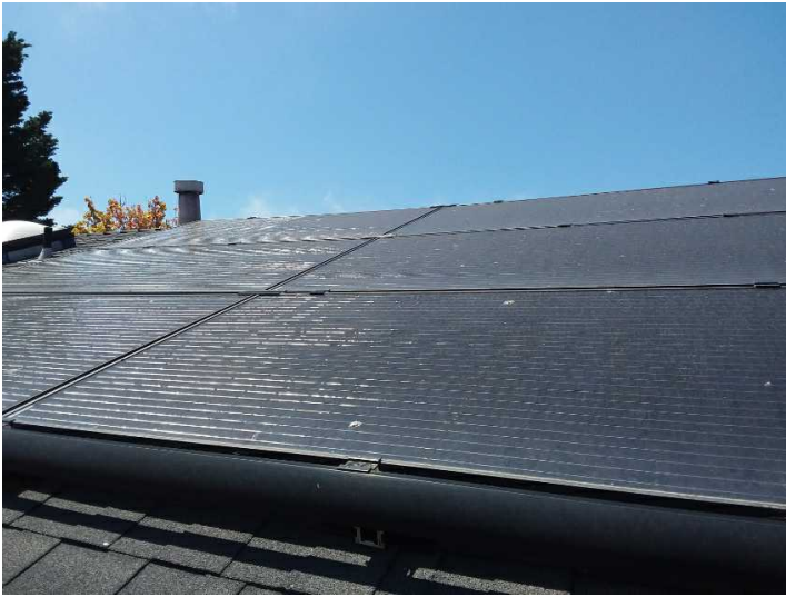
6 panels on upper rear roof
