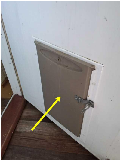
A pet door has been added that violates the firewall and the door should be replaced.
