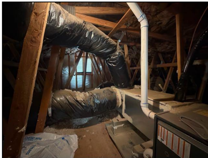
28. Ducts and registers
