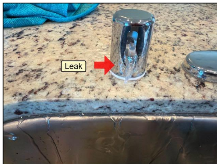
58. Air-Gap Device Leaks
