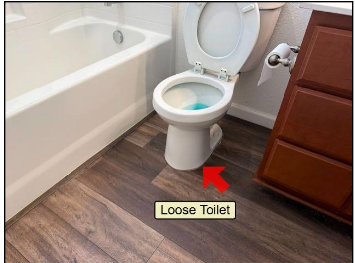
47. Toilet is loose on floor.
