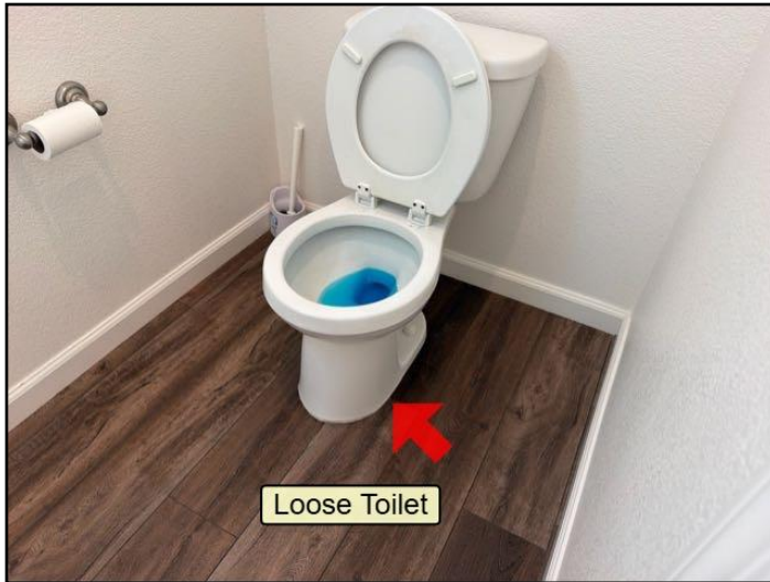
46. Toilet is loose on floor.
