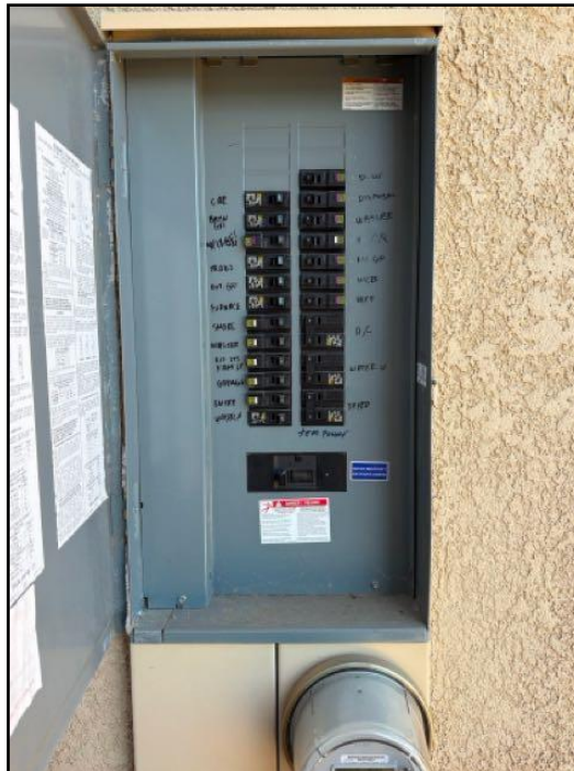
25. Breakers - exterior wall
