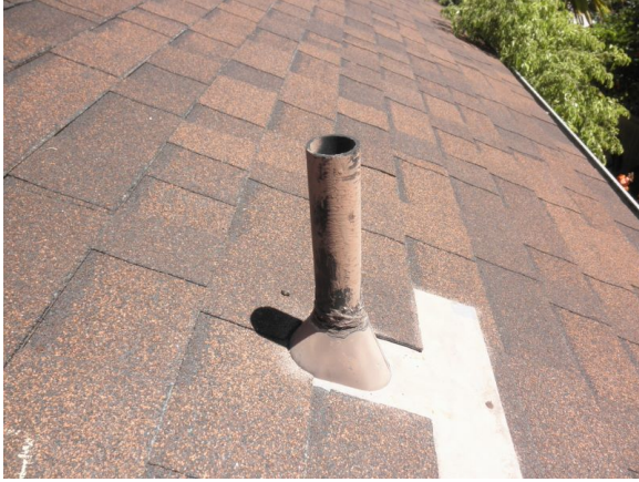
Deteriorated sealant at the vent flashings.
