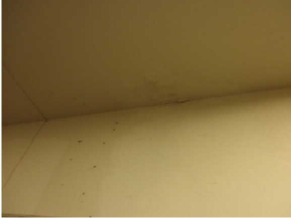
Evidence of a possible leak at the water proof deck as seen from inside the garage.
