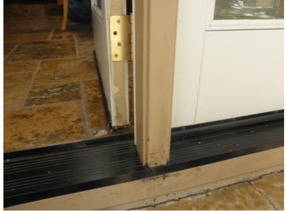
Moisture damage to the base of the door frame in the kitchen nook.
