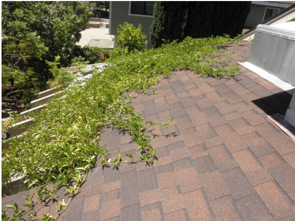
The foliage needs to be cut back off the roof.
