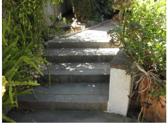
Missing railing at the concrete stairs in the backyard.
