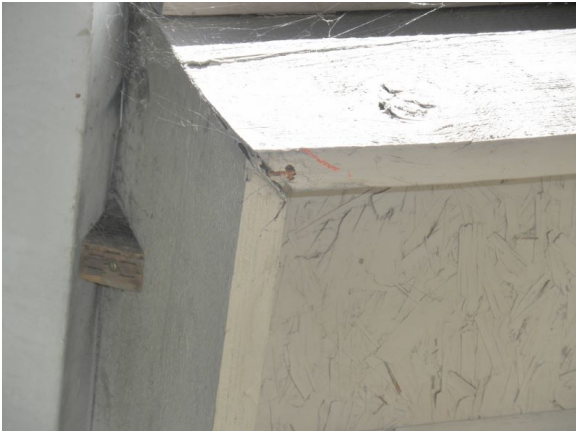
Moisture damage at the fascia board.
