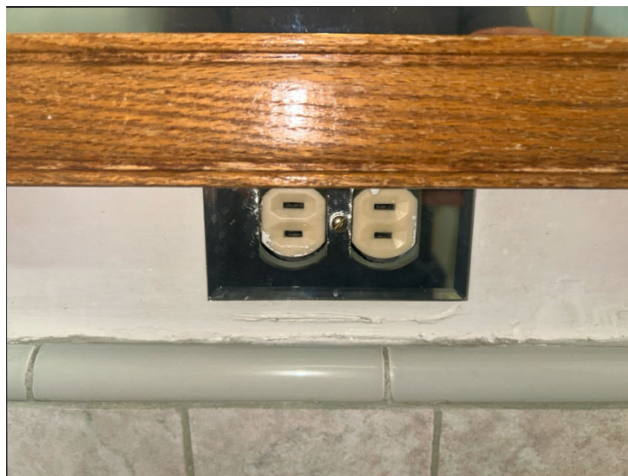
recommend all bathroom outlets be -GFCI outlets
