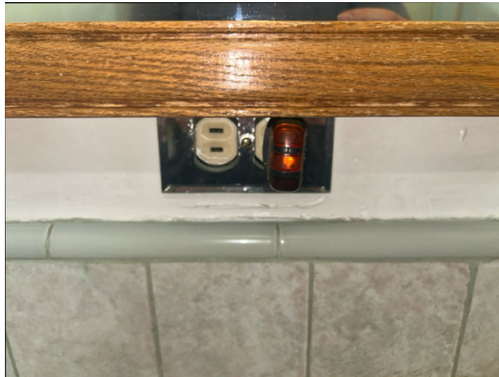
2 prong outlets present
