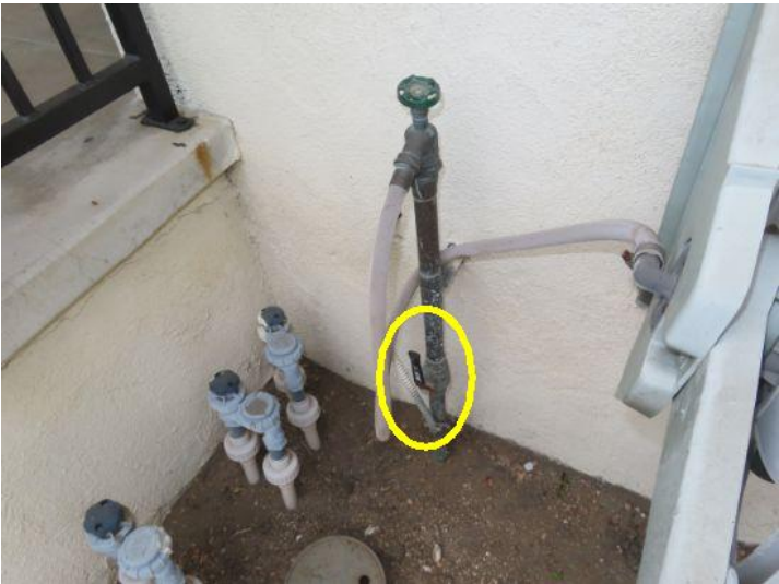
main water shut off
