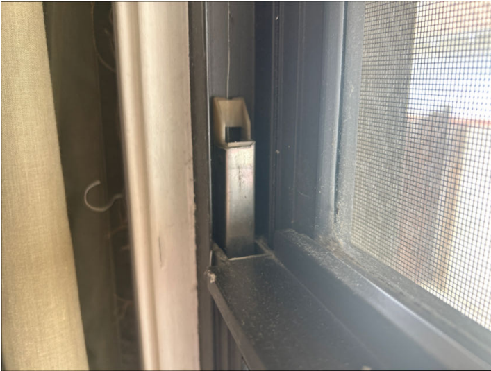
broken balance spring at the window
