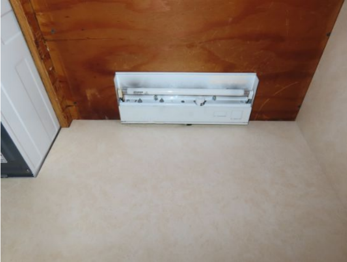
under cabinet light did not operate
