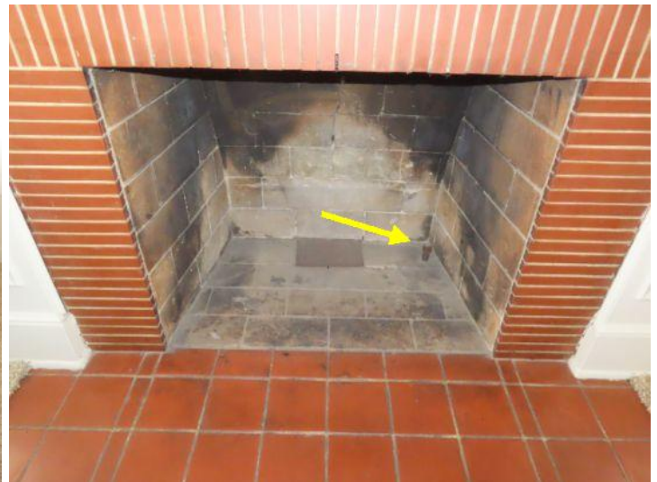
gas line is capped
