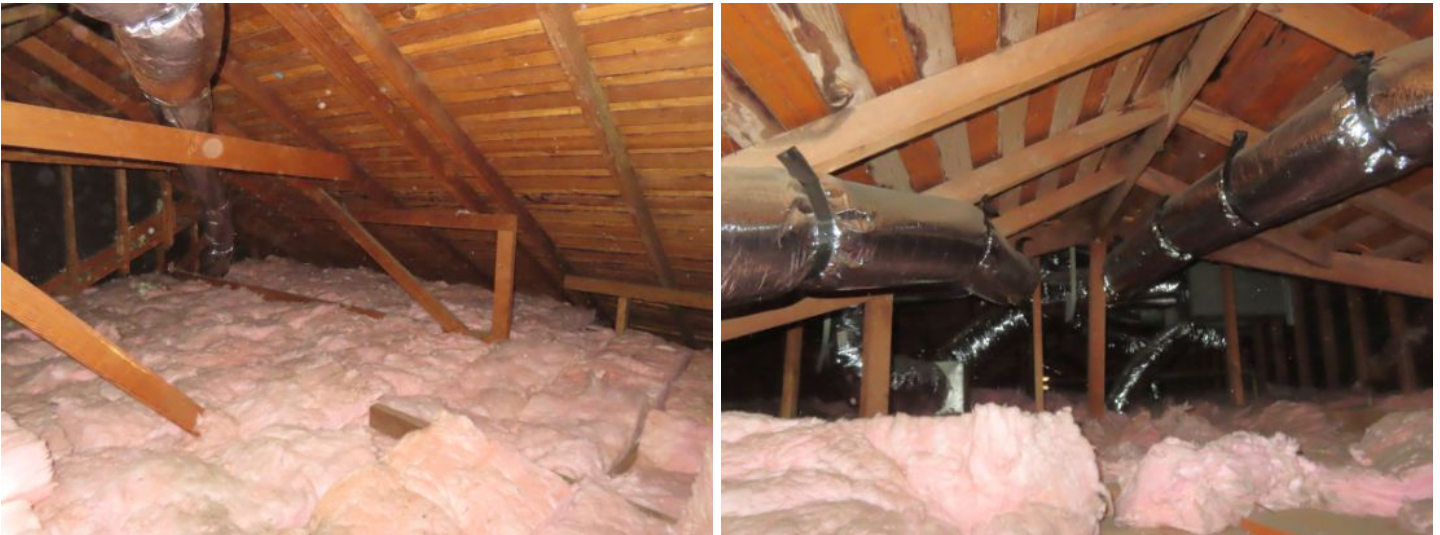
stains in areas, evidence of past leaking
