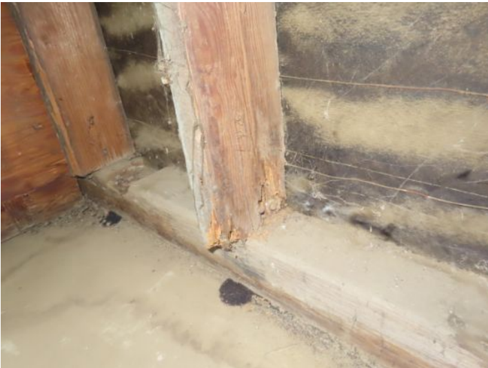
deteriorated wood, consult termite report
