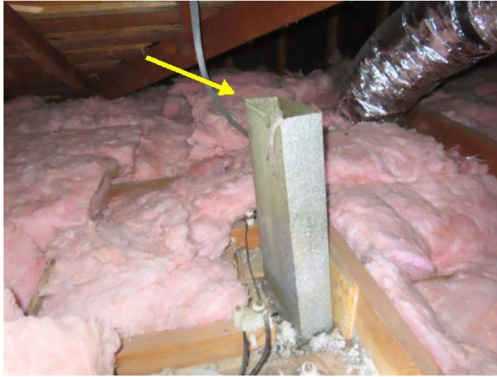
kitchen exhaust vent terminates in the attic
