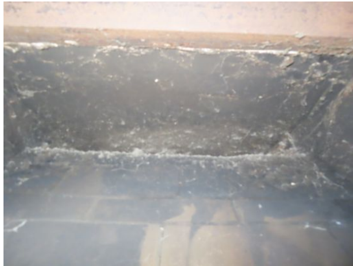
damper door missing
