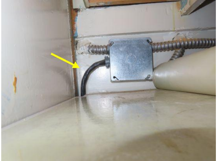
exposed romex wires inside the cabinets
