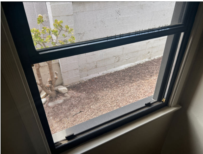
broken balance spring at the window
