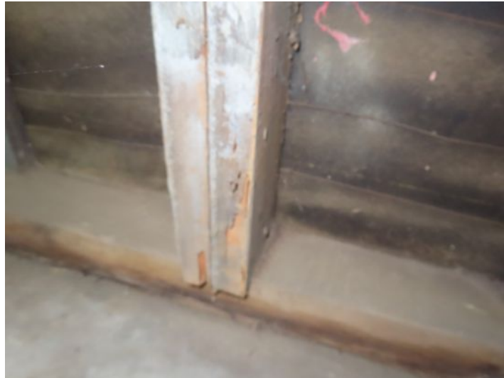
deteriorated wood, consult termite report
