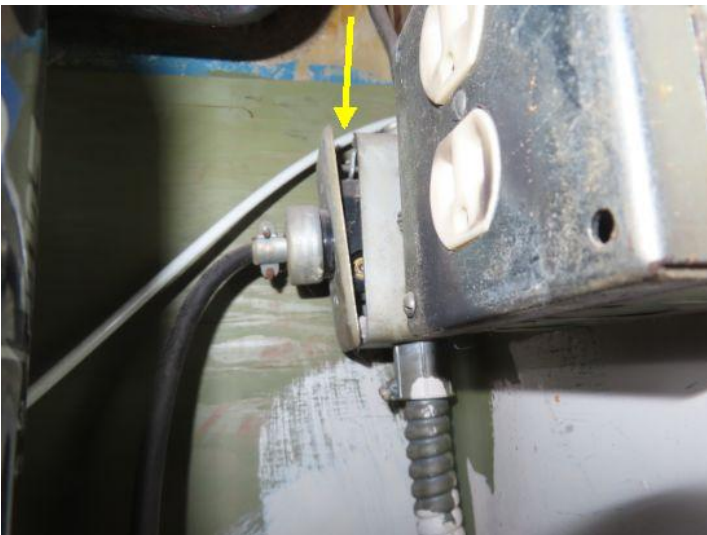
loose outlet under the sink
