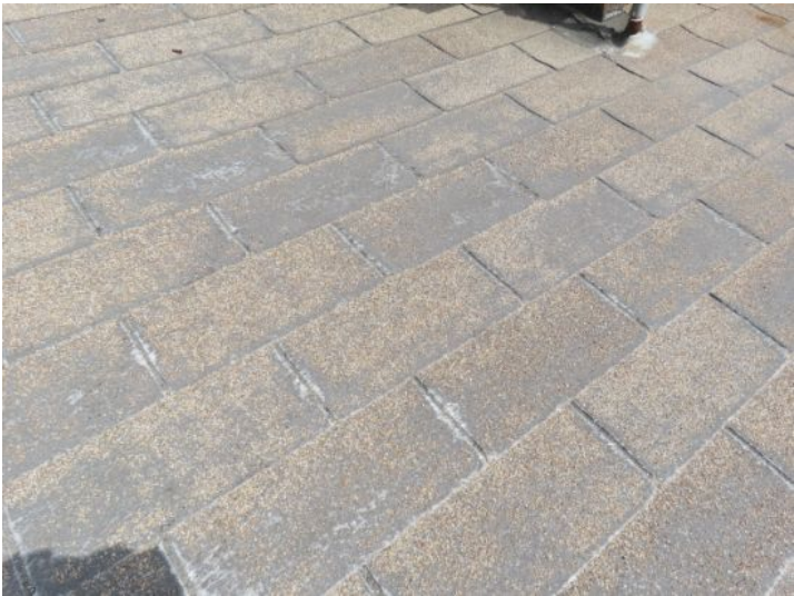
deteriorated roofing material
