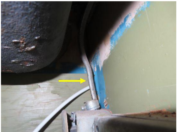
exposed romex wires inside the cabinets
