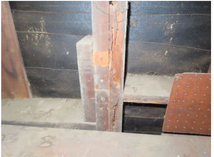
deteriorated wood, consult termite report
