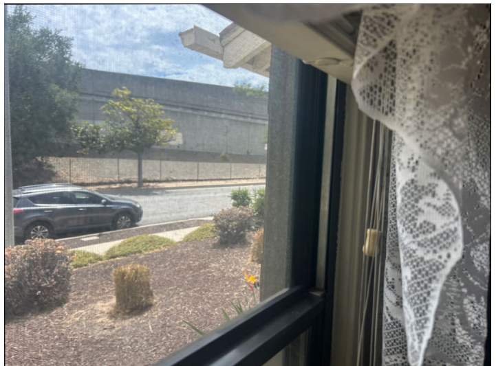
broken balance spring at the window
