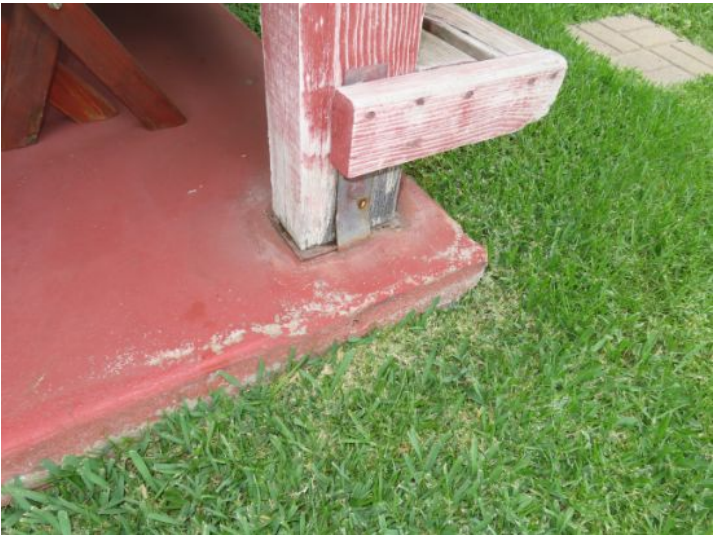
earth to wood contact
