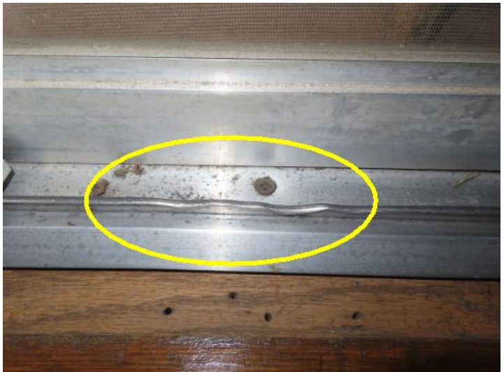
worn track, sliding door bounces
