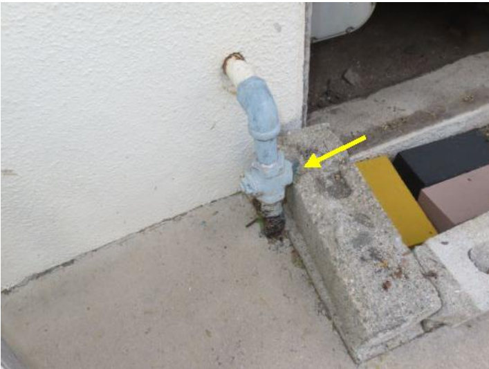
main gas shut off
