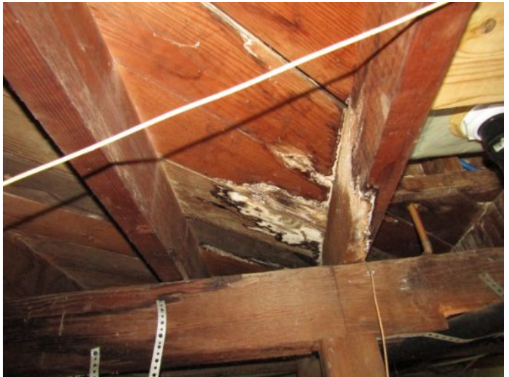
deteriorated wood in areas
