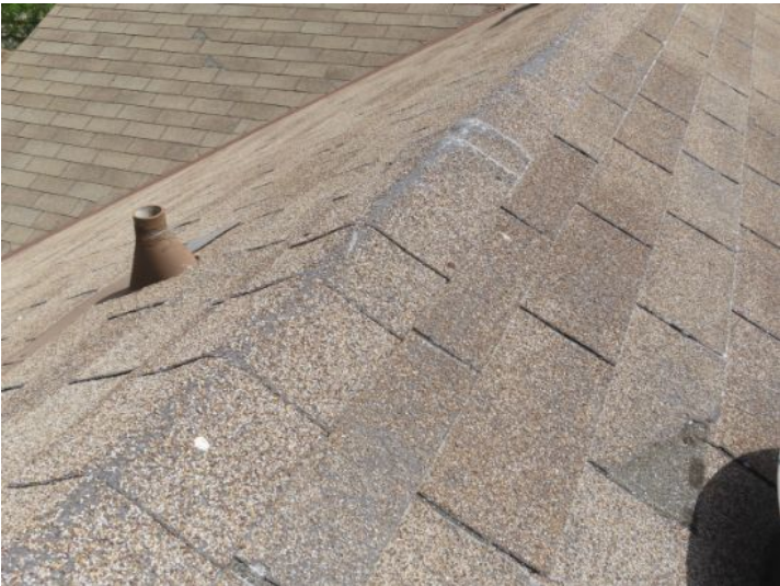
deteriorated roofing material
