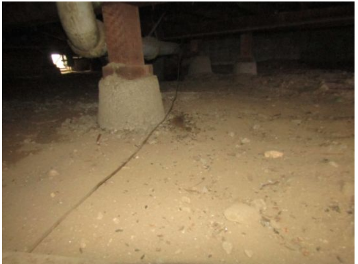
rodents droppings present
