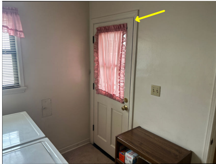
laundry door sticks at the jamb
