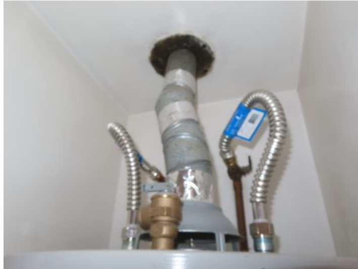
metal vent pipe vents into an old asbestos transit vent pipe
