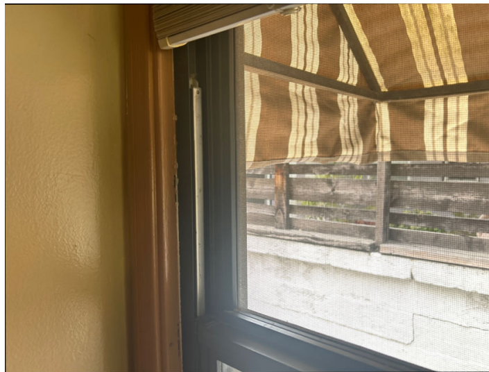
broken balance spring at the window
