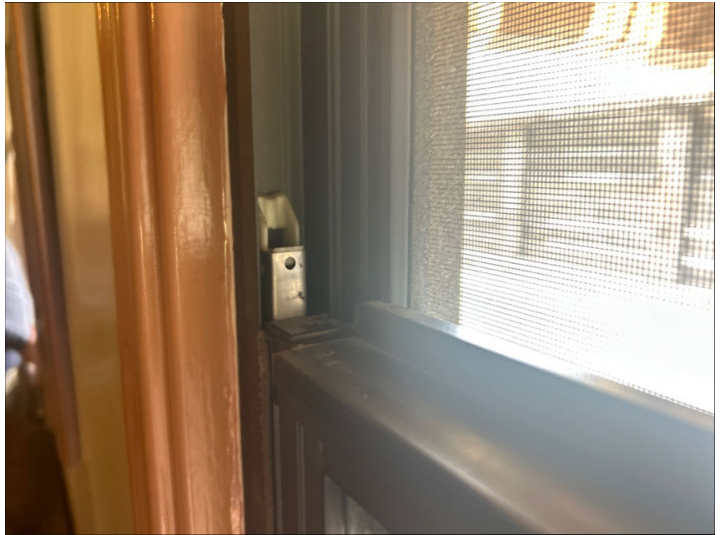
broken balance spring at the window
