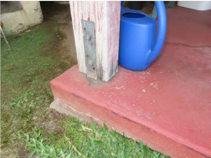
earth to wood contact
