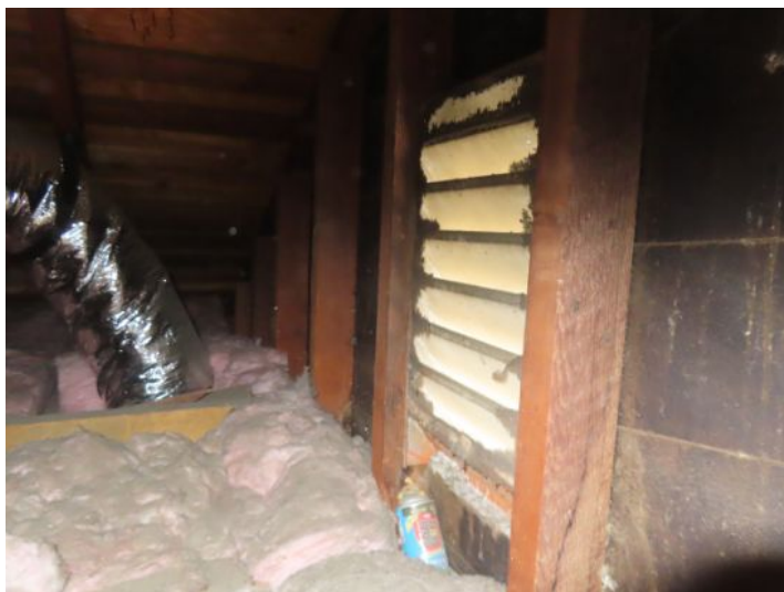
missing screens at the attic vents
