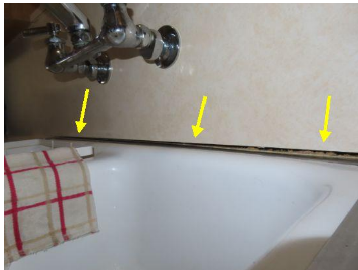
gapped at the sink area, recommend caulking
