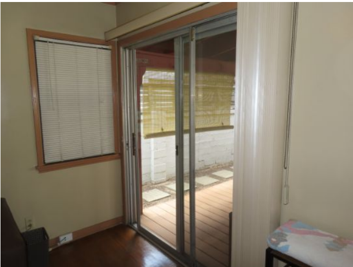
worn track, sliding door bounces
