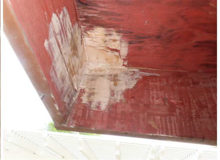
evidence of leaking at the eaves
