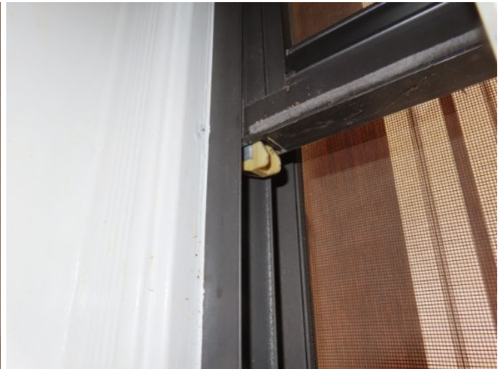
loose balance spring at the window
