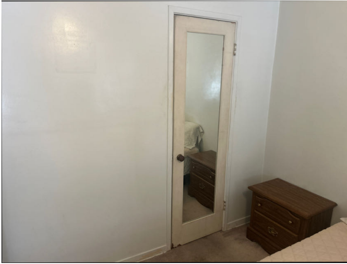
closet door did not latch
