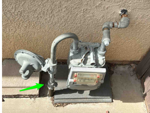
Main gas shut off valve
