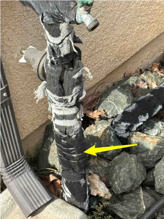
Shut off valve covered with duct tape
