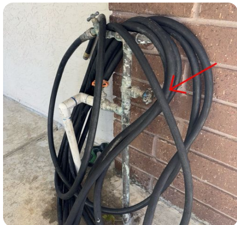
Main water control valve at garage exterior.
