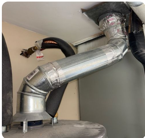
Functional water heater exhaust flue.
