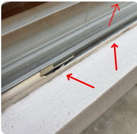
Damaged exterior cladding at bedroom window
