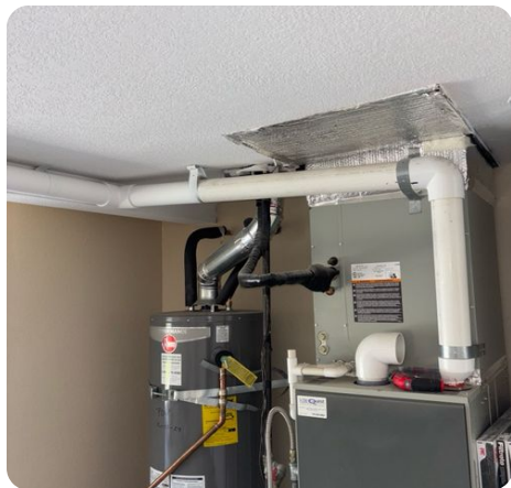
Functional furnace exhaust flue.
