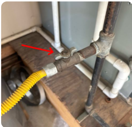
Natural gas control valve serving water heater.
