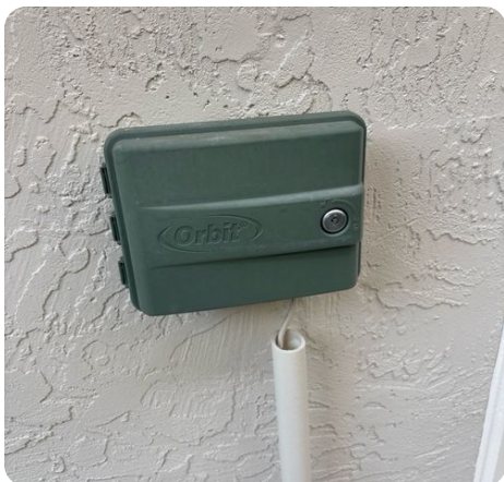
Irrigation control module at garage exterior.
