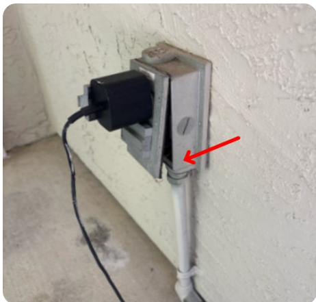
Loosely installed electrical outlet at rear patio.
