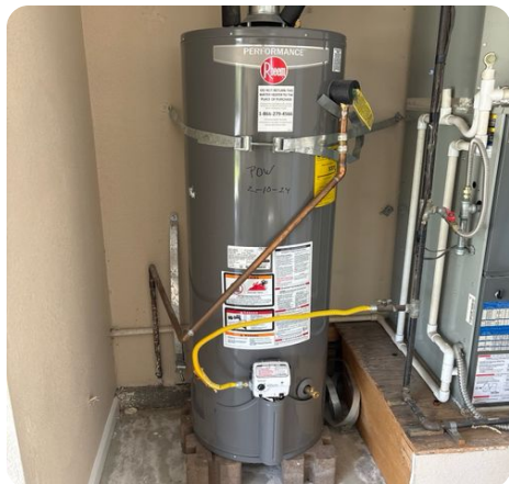
Rheem branded natural gas water heater within garage.
