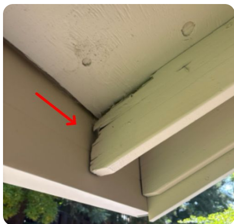
Moisture related damage at rafter tail.
