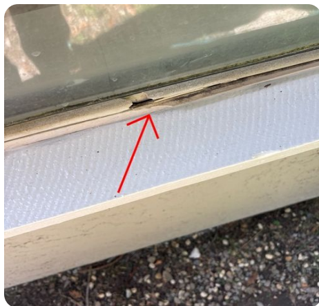
Damaged vinyl cladding at kitchen window exterior.
