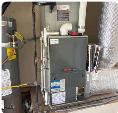
Trane branded, high efficiency, natural gas furnace within garage.
