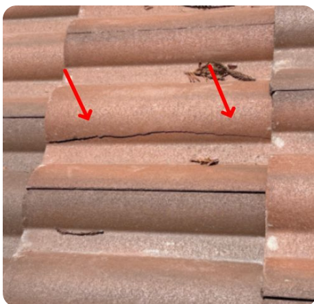
Cracked tile at upper roof surface.
