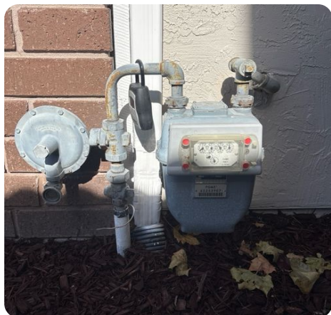
Natural gas meter at garage exterior.
