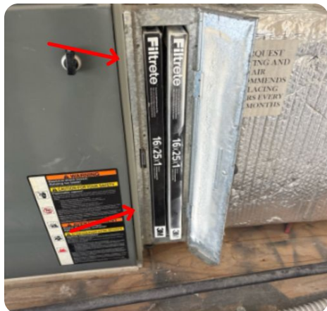
Clean, disposable HVAC filters at enclosure adjacent to furnace.
