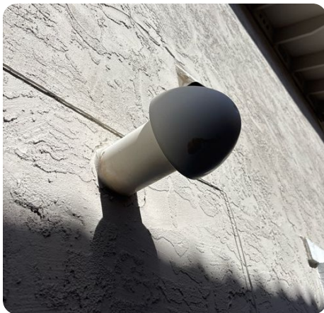
Functional furnace exhaust vent cover.
