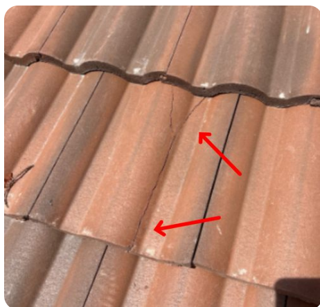
Cracked tile at upper roof surface.
