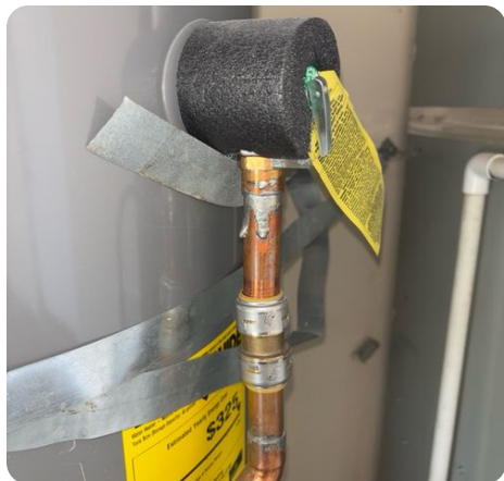
Water heater TPR valve with discharge tube.
