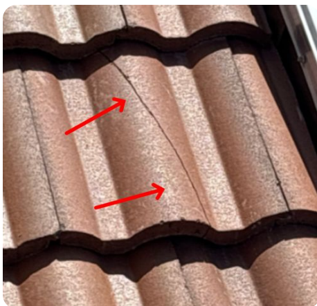
Cracked tile at upper roof surface.
