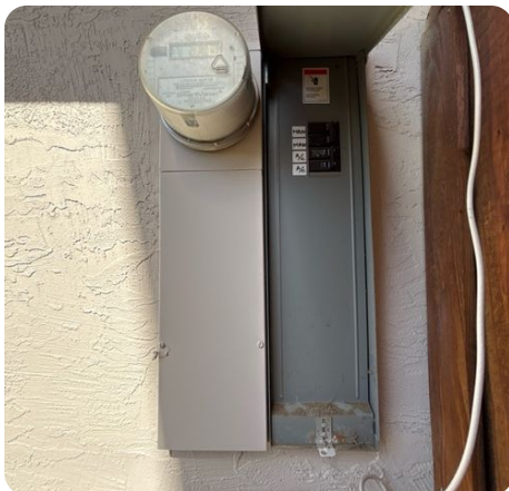
Original main service panel at garage exterior.
