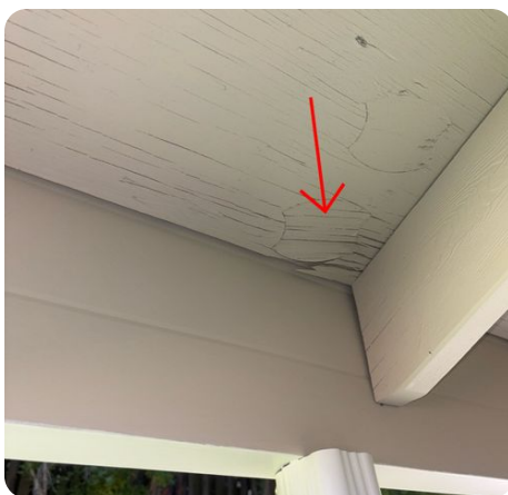
Moisture related damage at eave sheathing at kitchen exterior.
