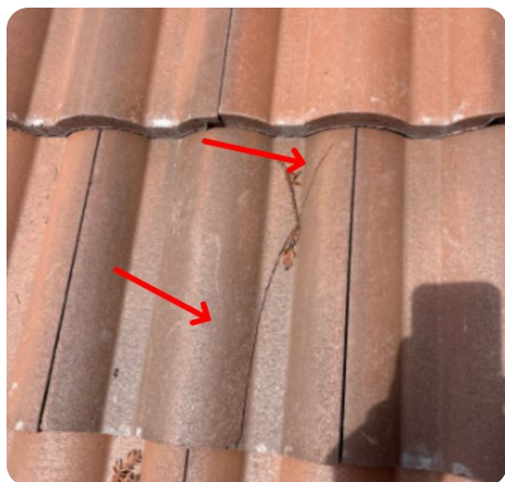
Cracked tile at upper roof surface.
