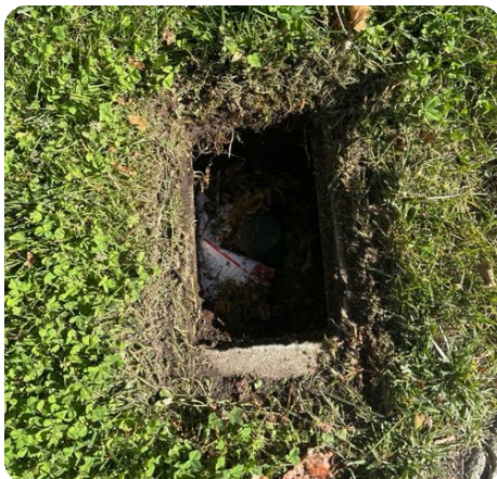
Water meter at front lawn.
