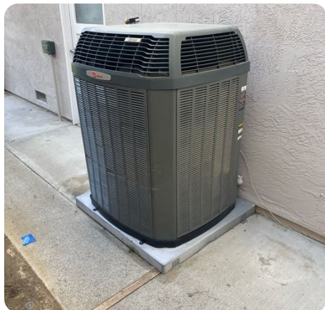
Trane branded condensing unit at bathroom exterior.
