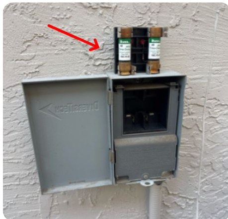
Appropriately sized condensing unit cartridge fuses at service disconnect.
