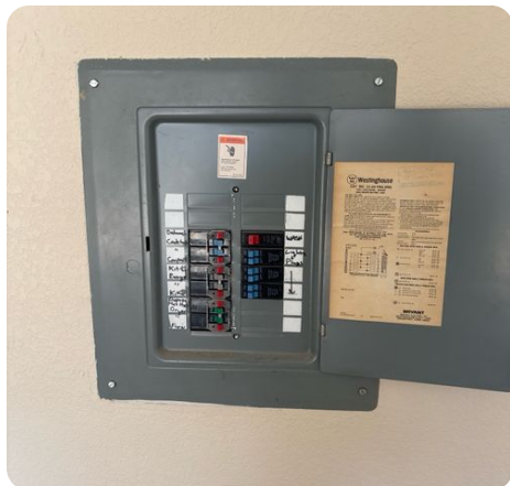
Original interior sub-panel within garage.
