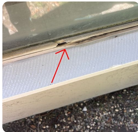
Damaged vinyl cladding at kitchen window exterior.
