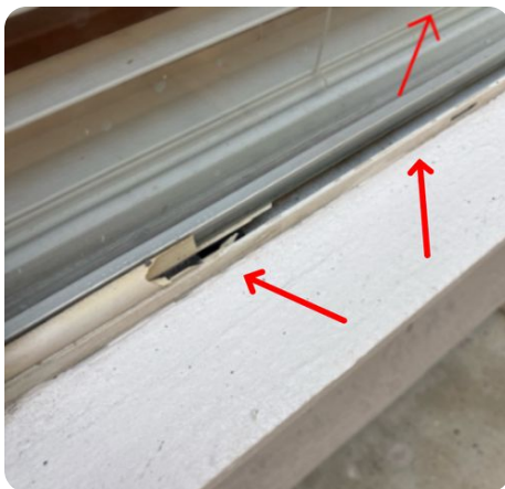
Damaged exterior cladding at bedroom window
