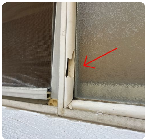
Damaged exterior window frame cladding at bathroom exterior.
