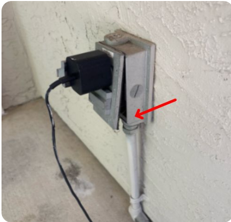
Loosely installed electrical outlet at rear patio.
