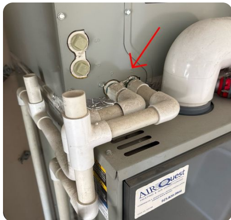
Dual HVAC condensate drain lines serving evaporation coil.
