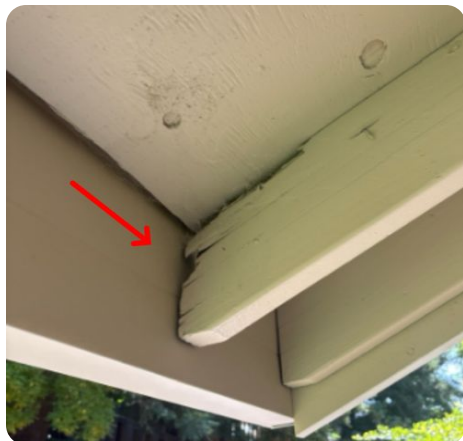
Moisture related damage at rafter tail.
