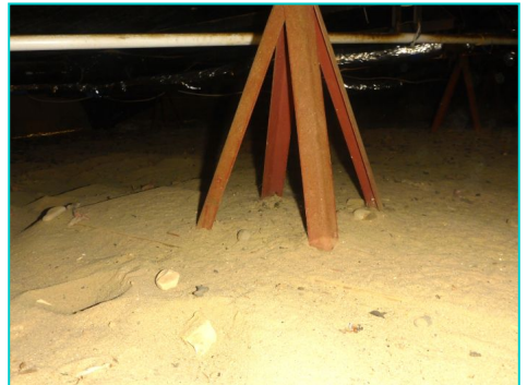
screw jacks covered in soil
