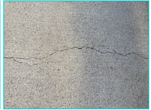
common cracks here
