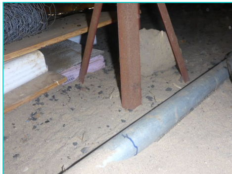
screw jacks covered in soil
