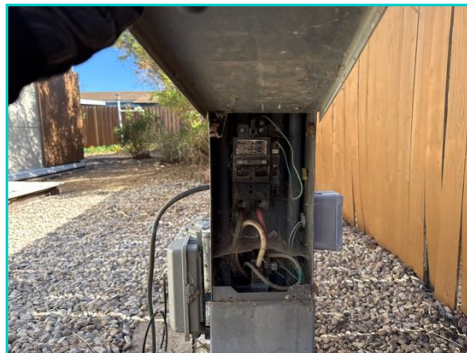
missing dead front cover
