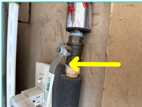
water shutoff valve
