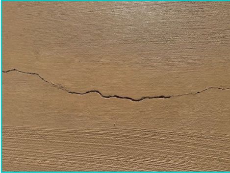
common cracks here
