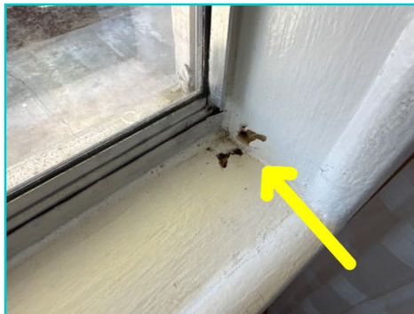
minor damage here
