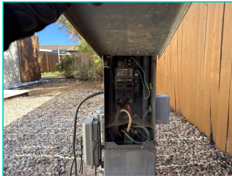
missing dead front cover
