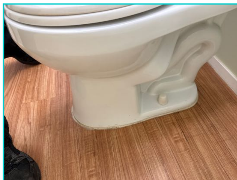
loose at floor
