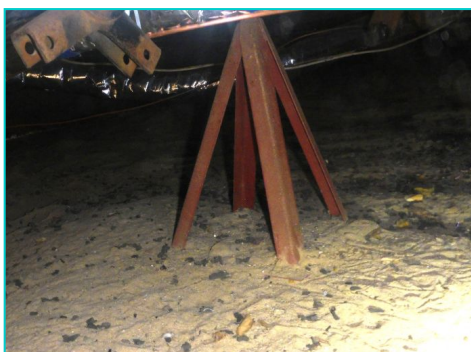
screw jacks covered in soil
