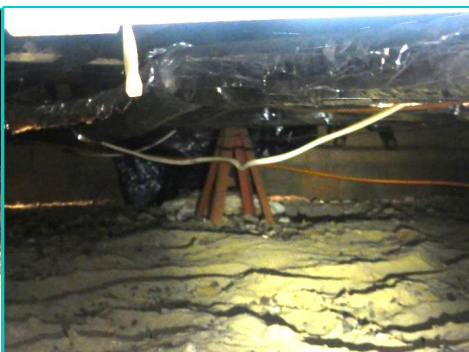
screw jacks covered in soil
