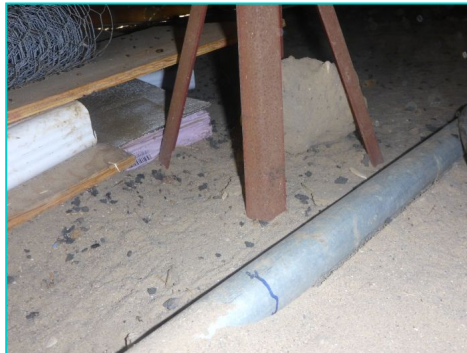
screw jacks covered in soil
