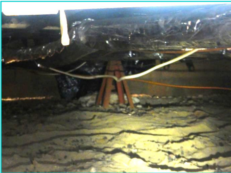
screw jacks covered in soil
