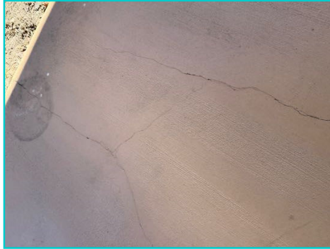
common cracks here
