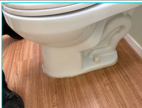
loose at floor
