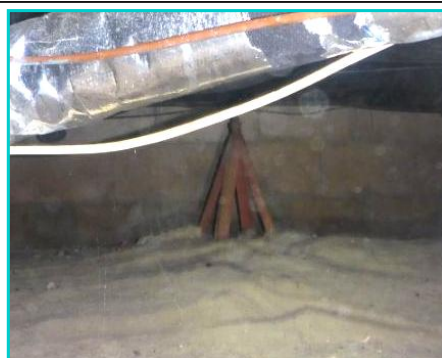
screw jacks covered in soil
