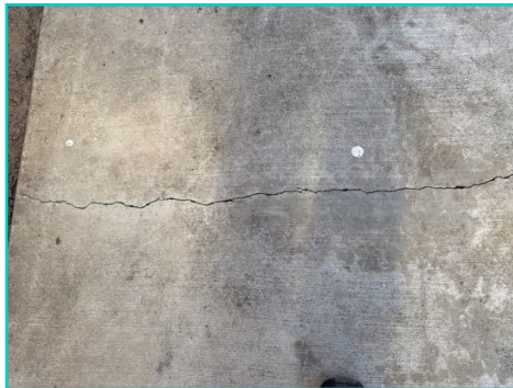
common cracks here
