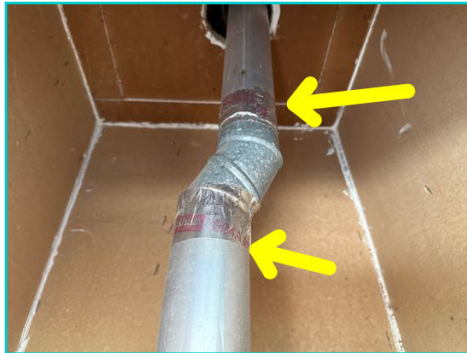
vent pipe needs screws at connections
