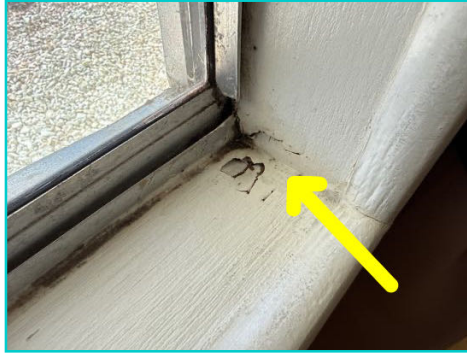
minor damage here
