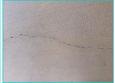
common cracks here
