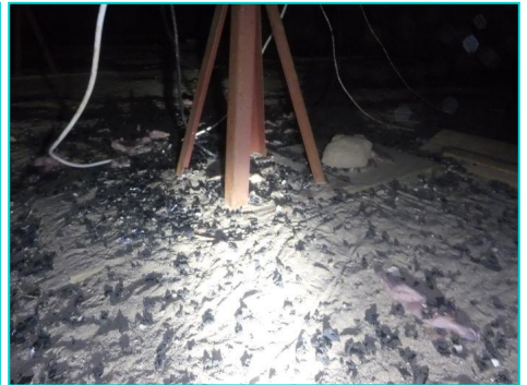
screw jacks covered in soil
