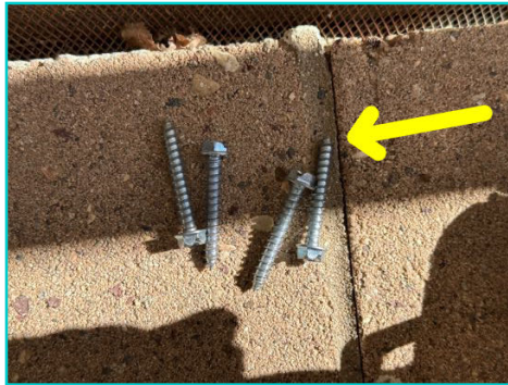
improper pointed screws
