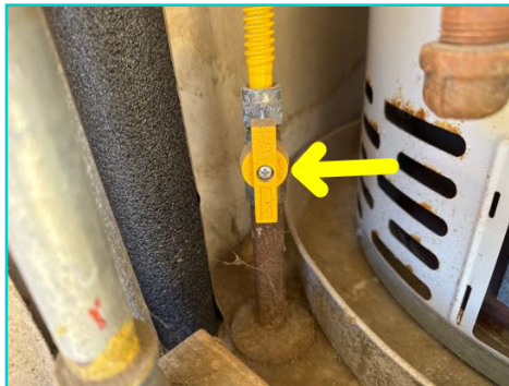
gas shutoff valve
