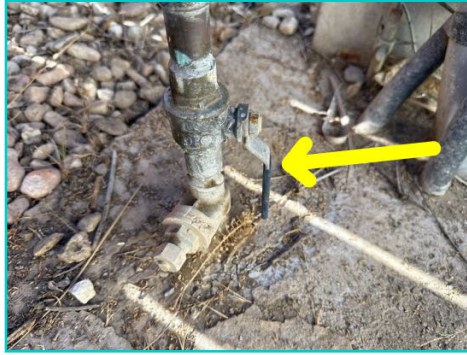
main water shutoff valve
