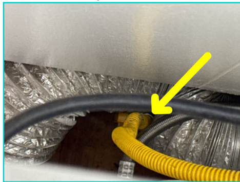
gas shutoff valve
