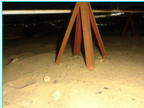
screw jacks covered in soil
