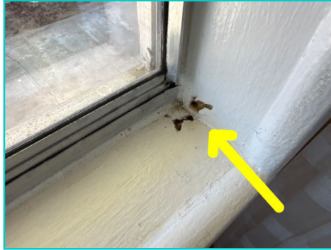
minor damage here
