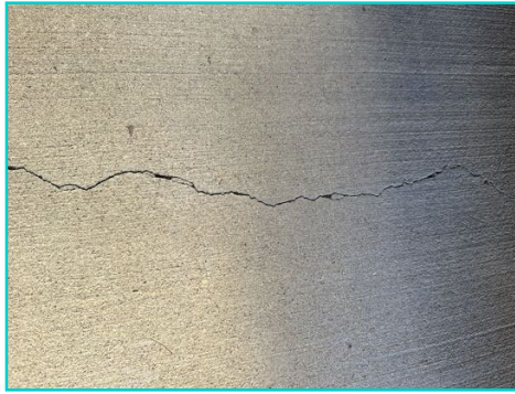
common cracks here
