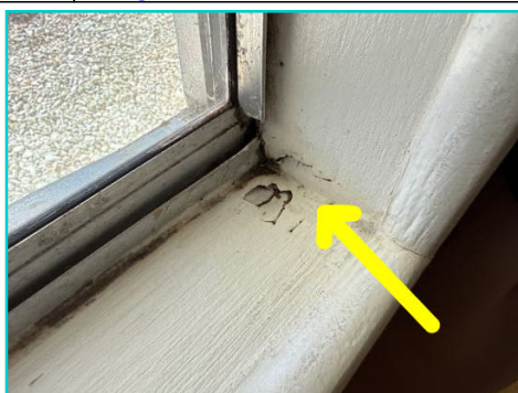
minor damage here
