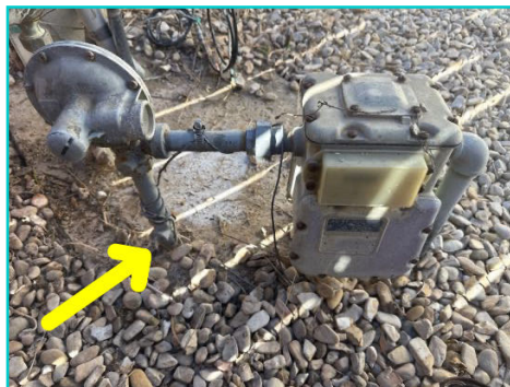
gas shutoff valve
