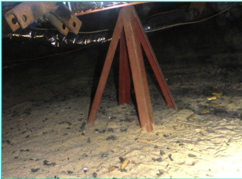
screw jacks covered in soil
