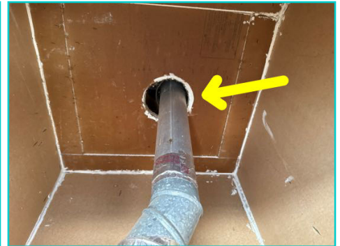
missing fire stop flange
