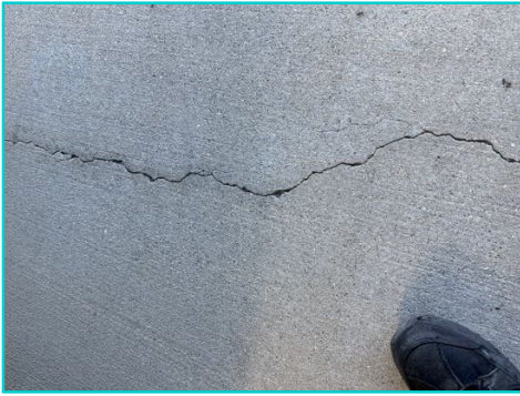
common cracks here
