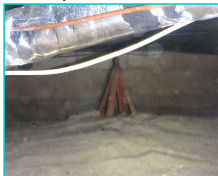
screw jacks covered in soil
