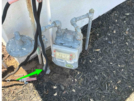
Main gas shut off valve
