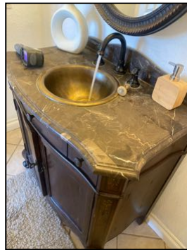
Counter top and cabinet loose at wall - not secured properly - needs to be serviced at downstairs half, upstairs hall bathrooms
