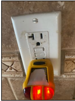
Test did not operate - right of sink - needs to be serviced
