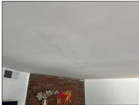
Stained area at living room - area tested dry at time of inspection - evidence of past moisture issues/leaking - consult seller
