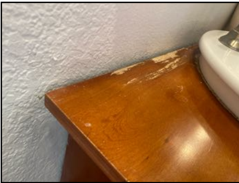
Counter top and cabinet loose at wall - not secured properly - needs to be serviced at downstairs half, upstairs hall bathrooms
