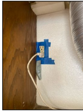
Outlet cover missing at vent cabinet - recommend service
