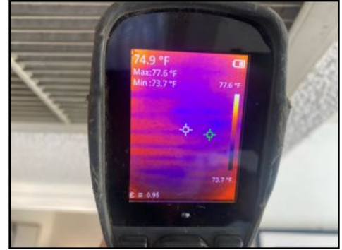
Temperature at Air Return: 74 degrees
