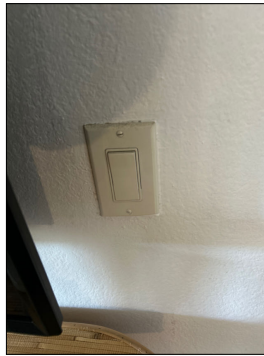
Switch ignition did not operate - needs to be serviced
