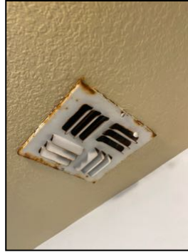
Rust present at register(s) - needs to be serviced at upstairs master bathroom
