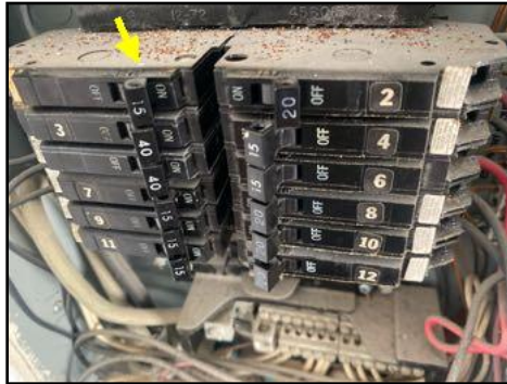
20amp Breaker in off position - cause could not be determined - recommend evaluation
