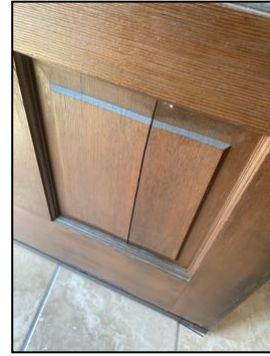
Cracked/splitting at front door - signs of age/wear - recommend service
