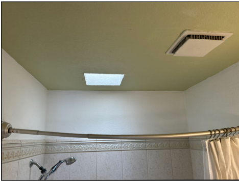
Spotty areas or signs of moisture accumulation on ceiling in areas - recommend improving ventilation in the bathroom
