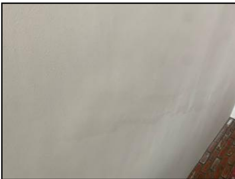
Stained area at living room - area tested dry at time of inspection - evidence of past moisture issues/leaking - consult seller
