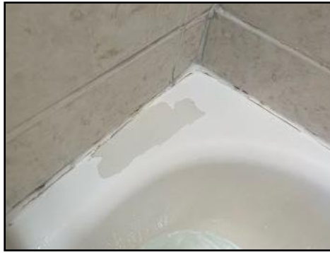
Materials are peeling/chipped at tub - minor
