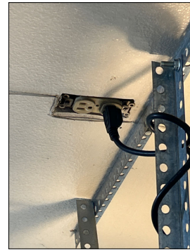
Outlet cover missing - needs to be serviced
