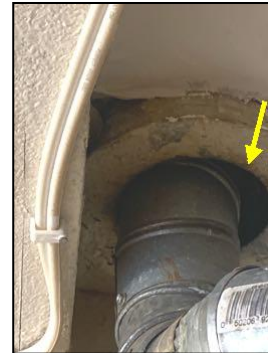
Loose connections – needs to be serviced
