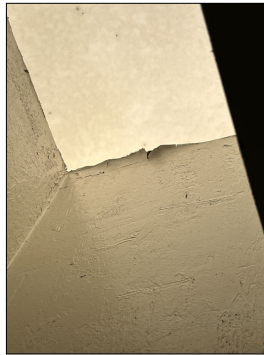
Peeling/blistered/cracking paint in areas
