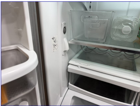
Seller: The refrigerator had a water dispensing and ice making system installed, but were turned off at the time of the inspection. Suggest commenting on the functionality of the refrigerator's water and ice maker and dispensing systems.
