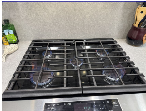
The kitchen gas oven was tested using the installed controls and it functioned normally at the time of the inspection. Verified with an infrared thermometer. See photo.
