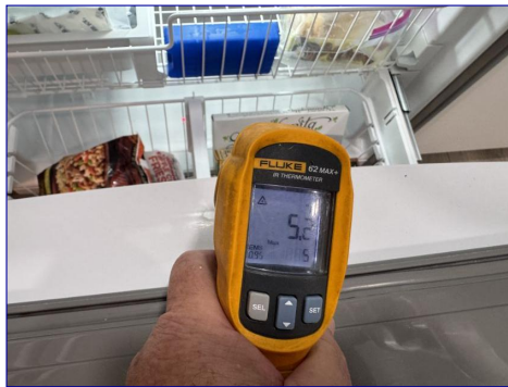
The refrigerator was tested with an infrared thermal meter showing a normal temperature and found to be functional at time of inspection. See photo.
