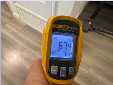
Central Heating / Cooling Systems Forced Air System Condition
