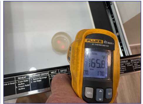
The microwave was found to be functional at the time of the inspection by placing a small cup of water inside and heating it for 40 seconds. See photo.
