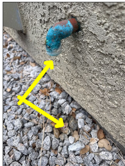
The pressure relief valve was leaking
