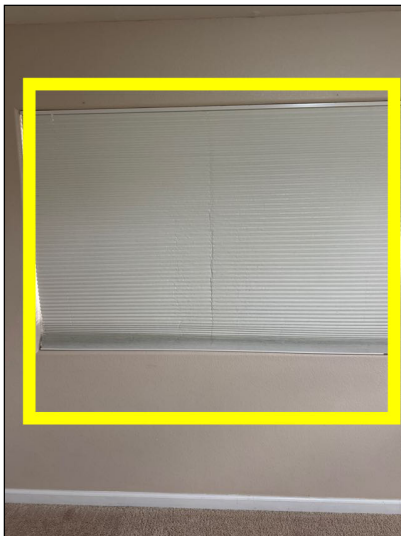
Window blind is broken and inoperable
