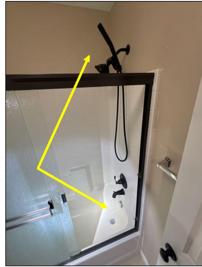
The diverter valve was leaking during operation or did not operate correctly (the diverter is the valve which diverts water from the tub faucet to the shower head).
