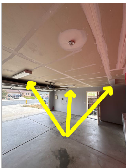
All light fixture in the garage did not respond to the switch at the time of the inspection.
