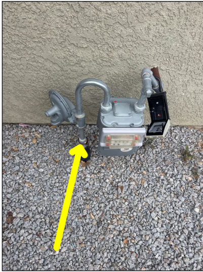
Main gas shut off to the home.
