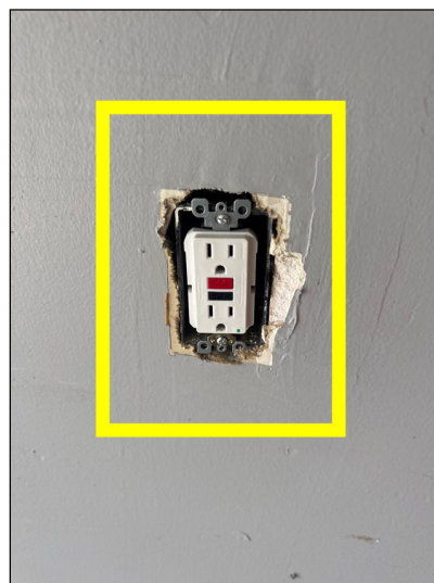
GFCI electrical receptacle was inoperable
