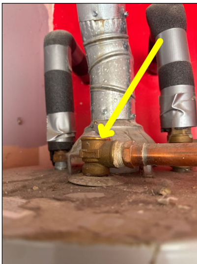
This is the TPRV valve
