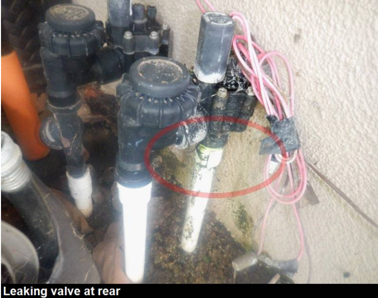
Leaking valve at rear
